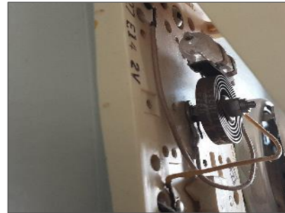
Mercury-containing thermostat in the Office (Location 5).
