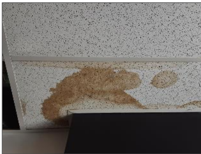
Water-stained acoustic ceiling tiles in the Corridor (Location 19).
