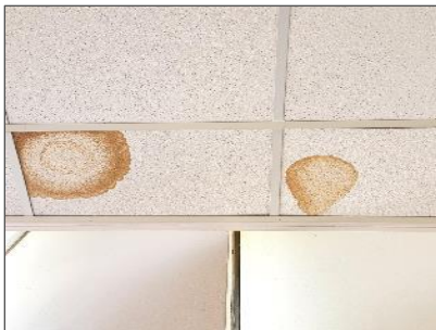
Water-stained acoustic ceiling tiles in the Staircase (Location 39).
