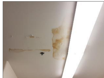
Water-stained drywall ceiling in the Men's Change Room (Location 8).
