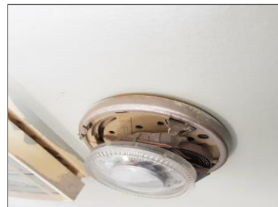
Mercury-containing thermostat in the Office (Location 5).
