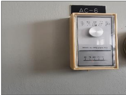
Mercury-containing thermostat in the Office (Location 5).
