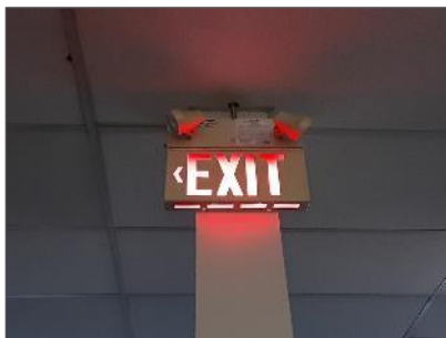
Emergency light with lead-containing battery in the Men's Change Room (Location 8).
