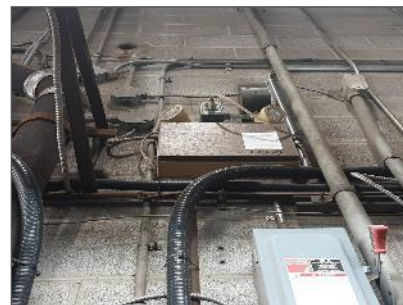
Emergency light with lead-containing battery in the Service Bay (Location 32).
