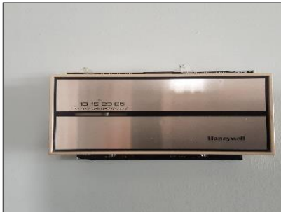
Mercury-containing thermostat in the Office (Location 5).
