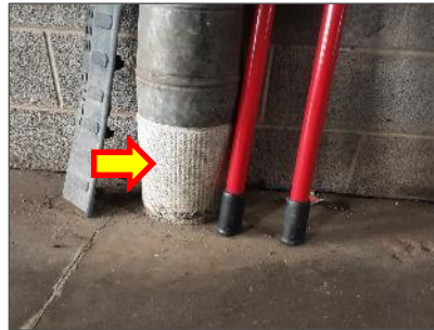
Transite pipe in the Service Bay (Location 32).
