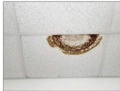
Water-stained acoustic ceiling tiles in the Corridor (Location 19).
