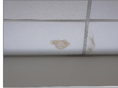
Water-stained acoustic ceiling tiles in the Men's Change Room (Location 8).
