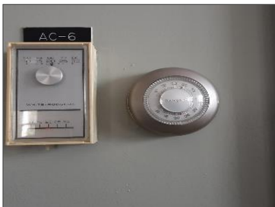
Mercury-containing thermostat in the Office (Location 5).
