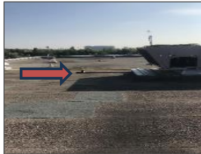
Pipe uninsulated, South roof section.
