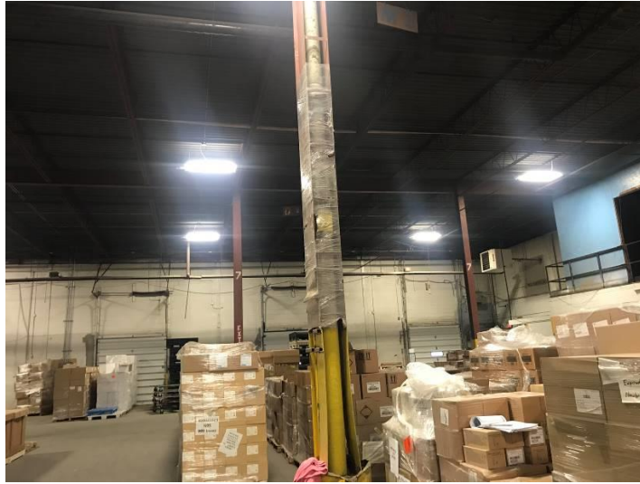
Photos 10, 11 – View of asbestos-containing Transite pipe observed in South Warehouse 1-22.
