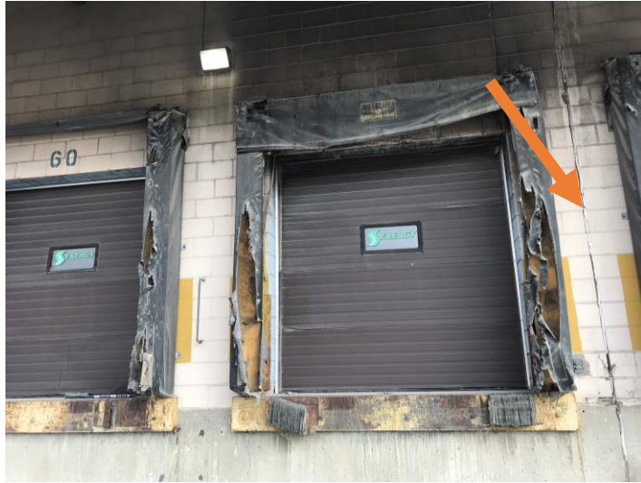
Photos 18 to 20: View of the asbestos-containing cream caulking along the exterior wall.
