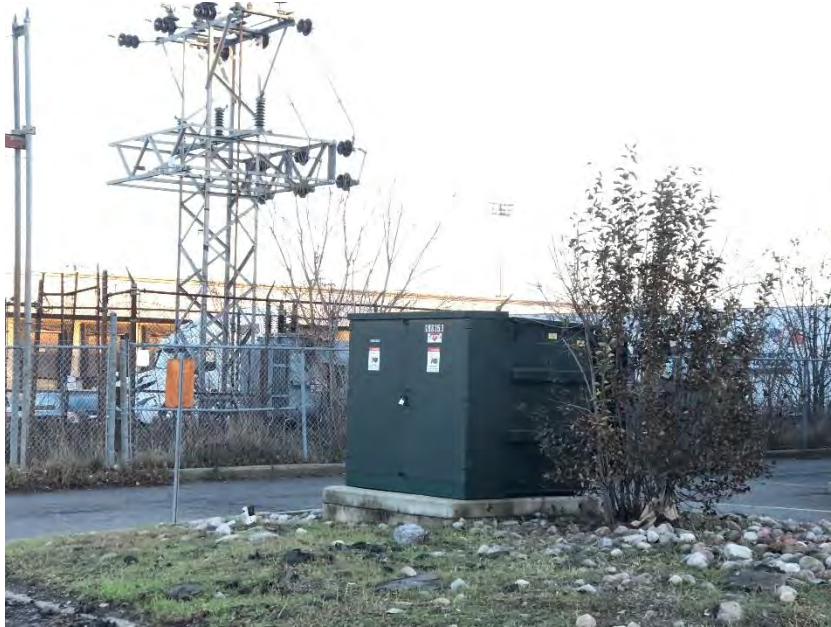
21. View of the Hydro One Site located to the west of the Site, facing northwest.
