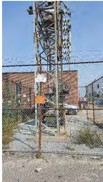
16. View of the transformer located on the southwestern portion of 36 North Queen Street, facing east.
