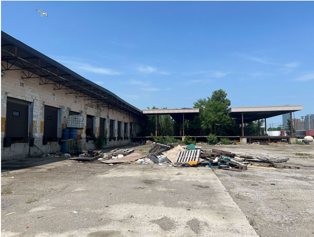
Photo #14: Typical Site Refuse at East Elevation
