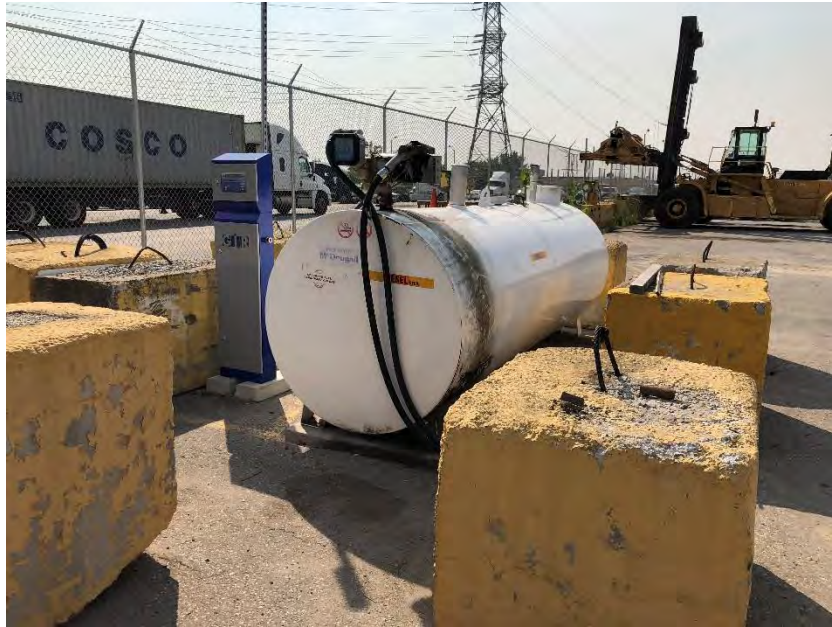
15. View of the diesel AST located on the south central portion of 36 North Queen Street, facing southwest.
