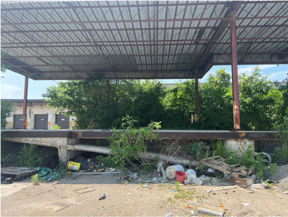
Photo #16: Typical Site Refuse at East Elevation
