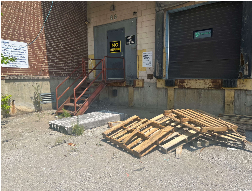
Photo #4: Typical Site Refuse at West Elevation
