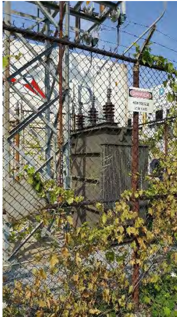
17. View of the transformer located on the north-central portion of 36 North Queen Street, facing north.
