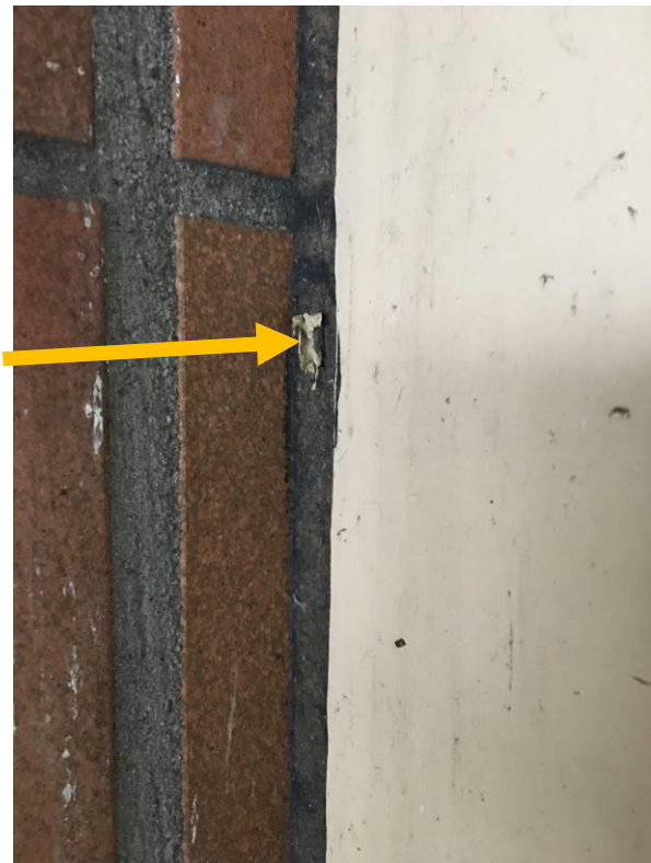
Photos 1, 2 – View of the asbestos-containing cream caulking on the wall in the Bus Bay.
