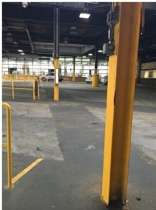
Photos 3, 4 – View of lead-containing yellow paint on metal columns.
