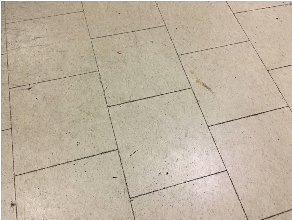
Photo 8 – View of the non-asbestos floor tiles observed on lower and upper level.
