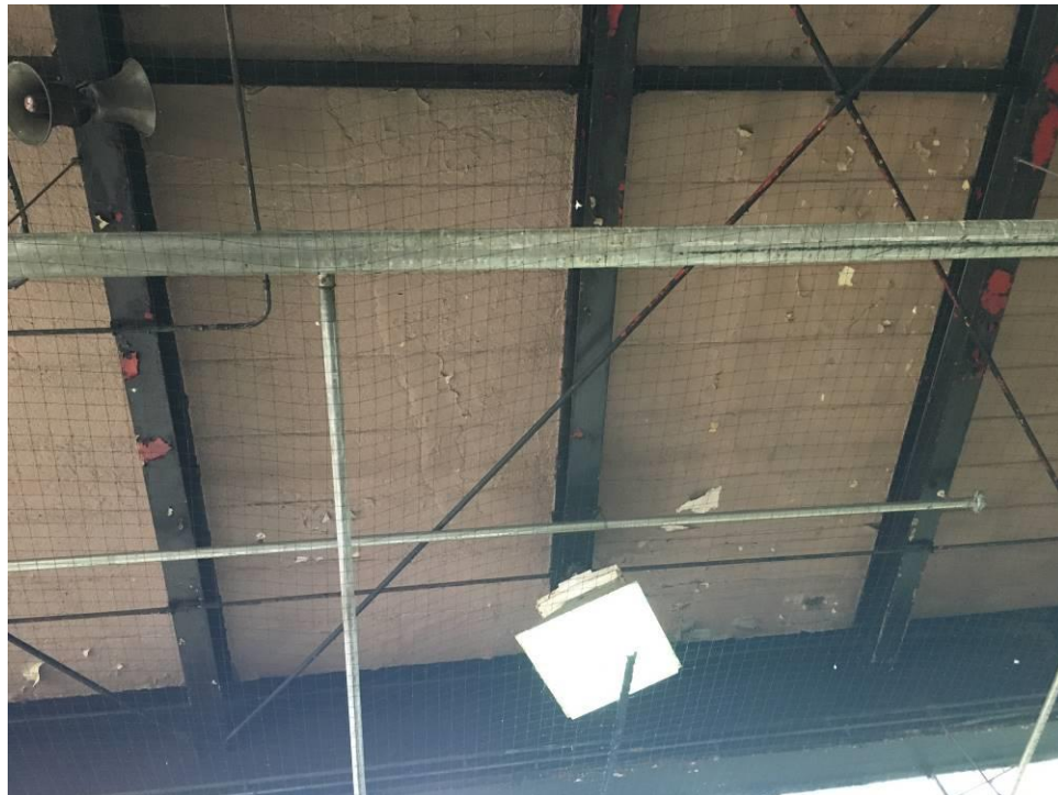
Photos 5, 6 – View of the ceiling in the Bus Bay with no lead containing paint.
