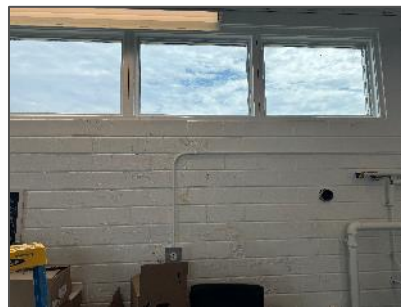
Lead-containing white paint on masonry wall – Storage Space (Location 1-01).
