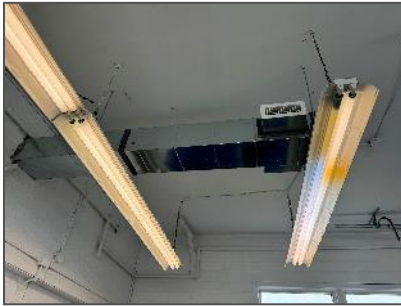
Uninsulated duct – Storage Space (Location 1-01).
