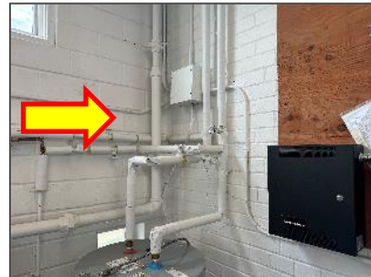
Pipes insulated with fibreglass and jacketed in paper – Storage Space (Location 1-01).
