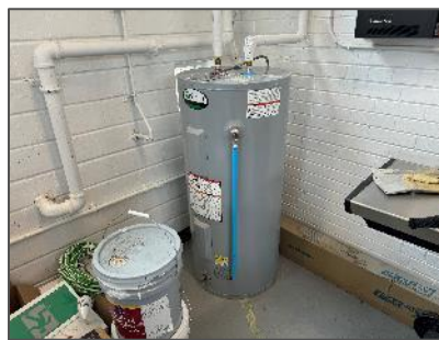
Hot water tank insulated with fibreglass and jacketed in metal – Storage Space (Location 1-01).
