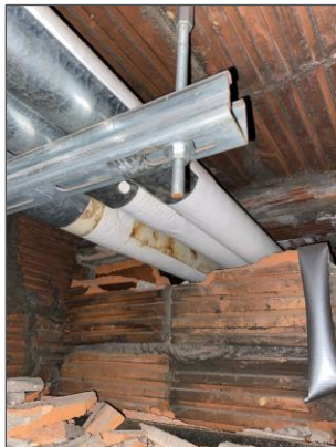
Preformed block insulated piping within East Corridor (Location 9)
