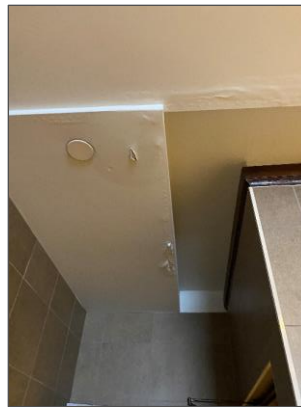
Visible water damage on drywall within Women's Washroom (Location 3)
