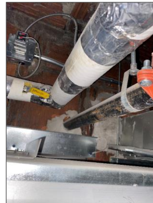
Non-asbestos pipe insulation with foil fittings.
