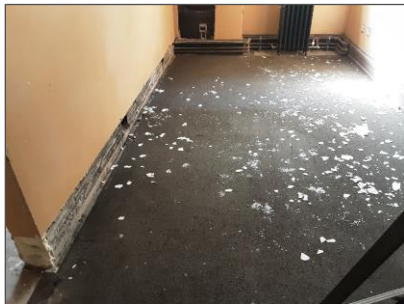
Carpet floor concealing asbestos-containing levelling compound in Location 5
