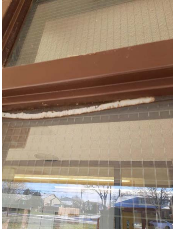
Photograph No. 3 – Glazing was observed between the glass and the frame/casing on the main entrance window. The glazing was sampled (S04A,B,C) and found to be asbestos-containing. The glazing was also sampled for PCBs (PCB3) and is non-PCB.
