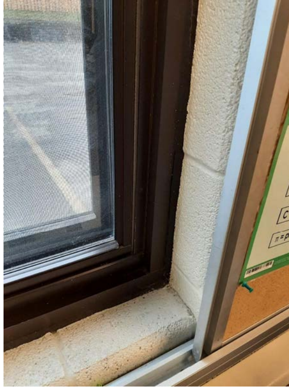
Photograph No. 1 – Black window sealant was observed around the perimeter of windows throughout the interior of the building. The sealant was sampled (S02A,B,C) and found to be asbestos-containing. The sealant was also sampled for PCBs (PCB1) and is non-PCB.
