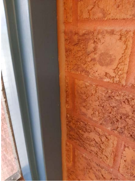
Photograph No. 5 – Brown sealant was observed around the perimeter of exterior doors. The sealant was sampled (S01A,B,C) and found to be non-asbestos. The sealant was also sampled for PCBs (PCB2) and is non-PCB.
