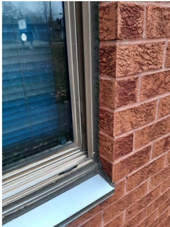
Photograph No. 2 – Black window sealant was observed around the perimeter of windows throughout the exterior of the building. The sealant was sampled (S05A,B,C) and found to be asbestos-containing. The sealant was also sampled for PCBs (PCB4) and is non-PCB.
