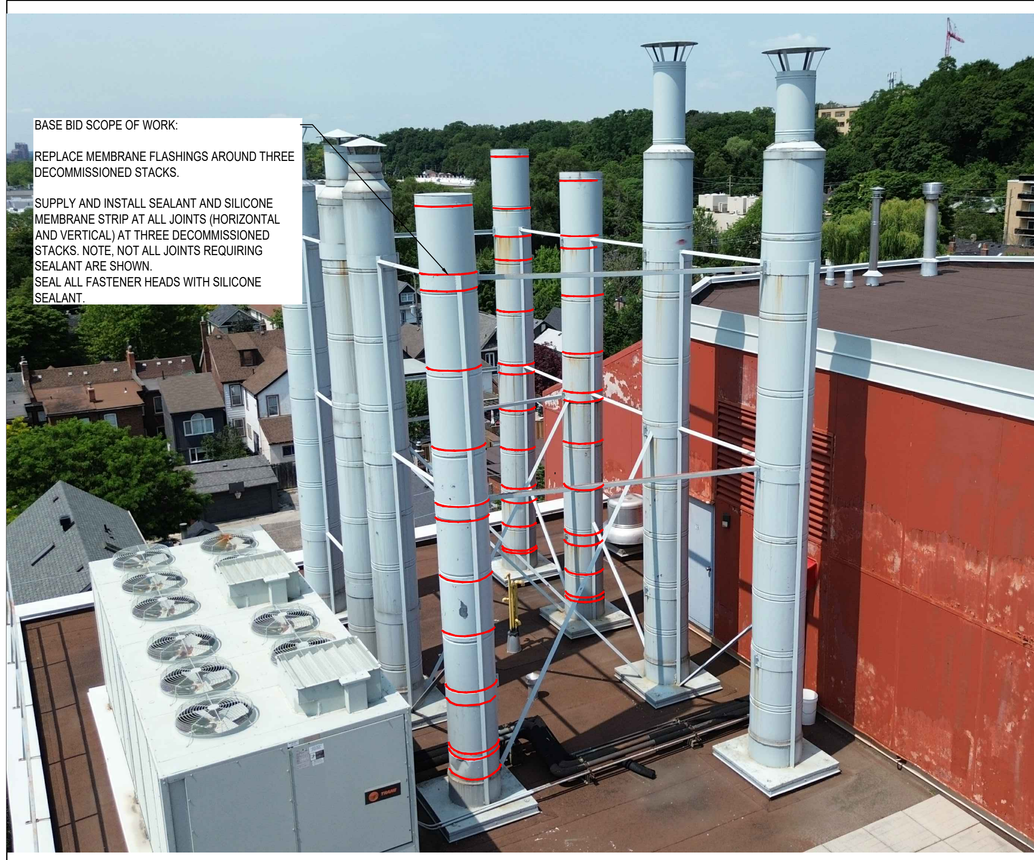
1 PHOTOGRAPH INDICATING BOILER VENTS TO BE REPAIRED (BASE BID) R503 SCALE: N.T.S.
