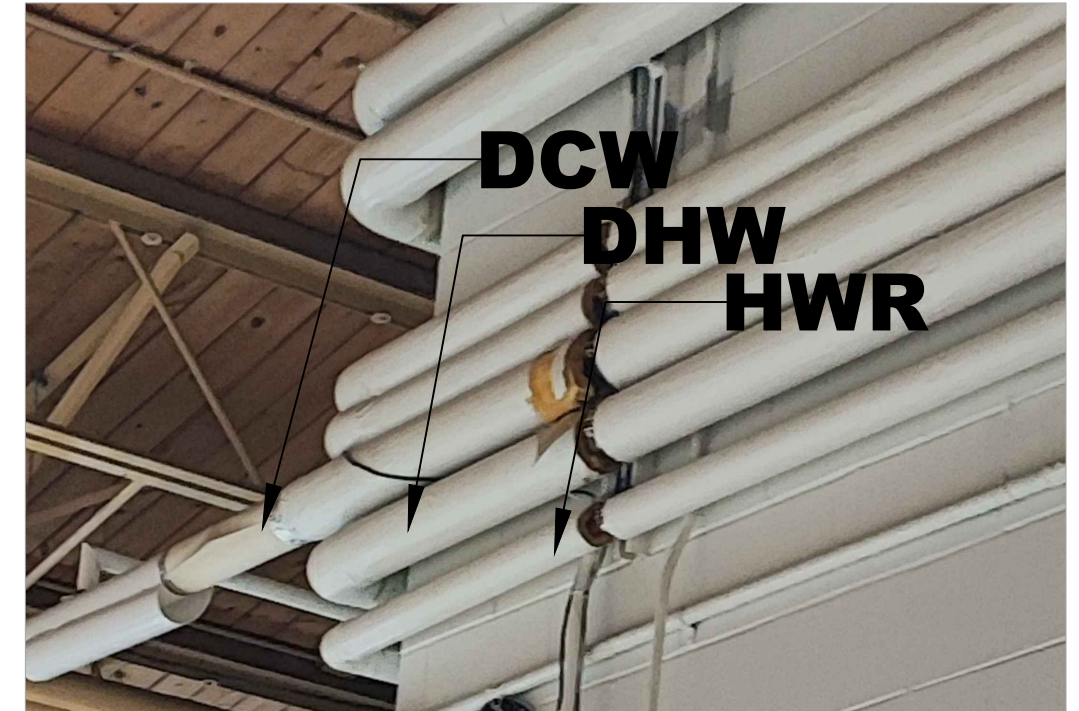
P.1. 2ND FLOOR JUNCTION OF THE DCW, DHW, HWR
