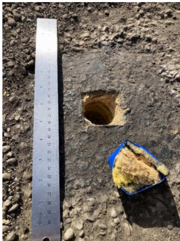
S1014B (Confirmed Asbestos), Roof materials, Roof B (Location #: 210)
