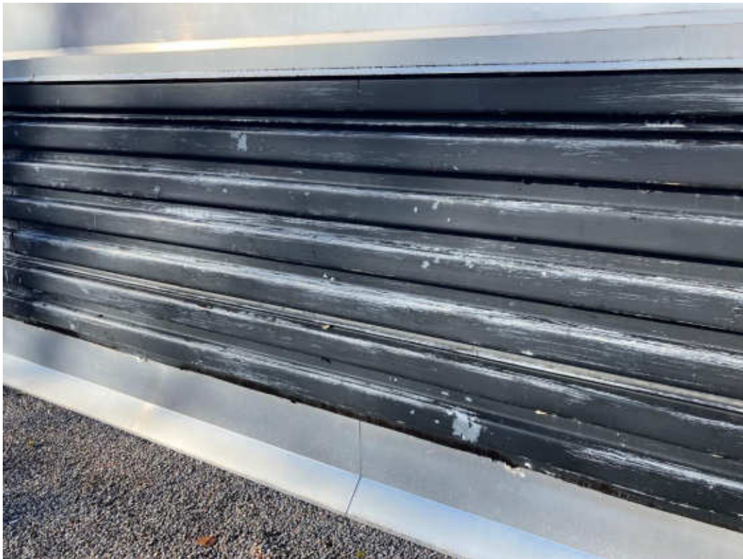
L0039 (Lead) Lead-based paint on metal on exterior of Mechanical Penthouse
