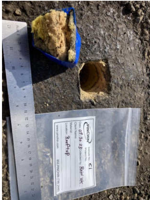
S1014C (Confirmed Asbestos), Roof materials, Roof C (Location #: 211)
