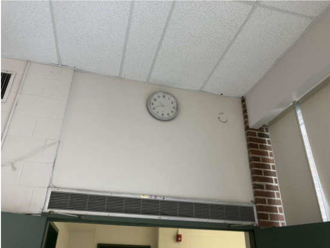
V0032 (Non-asbestos), Wall, Plaster, Cafeteria (Location #: 103) above doors and as bulkheads for windows
