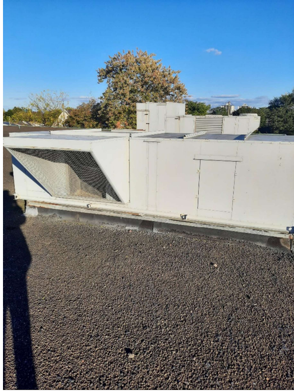
Photograph No. 5 – Roof top air handling unit was observed and may containing ozone depleting refrigerants.
