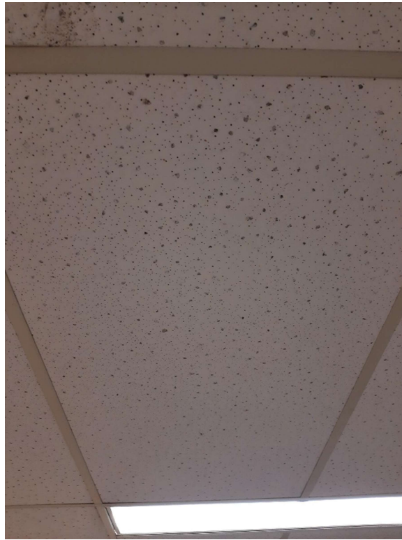
Photograph No. 1 – 2’x4’ Small dimple random pinhole ceiling tiles were observed throughout the interior and sampled (S02A,B,C). The ceiling tiles are asbestos-containing.
