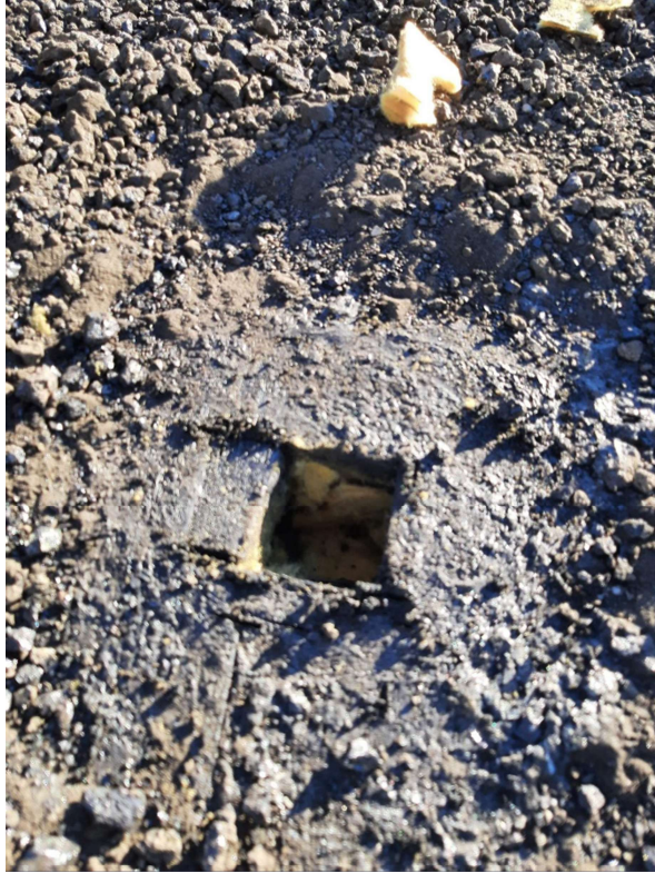
Photograph No. 3 – The roof composition was inspected and consists of a tar membrane, fiberglass insulation and the steel deck. The tar membrane was sampled (SS07A,B,C) and is non-asbestos.
