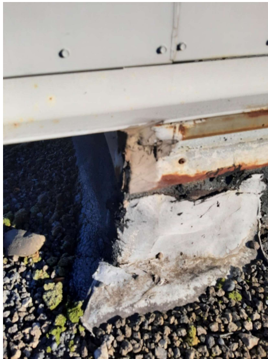
Photograph No. 4 – The mechanical sealant observed on the RTU was sampled (S01A,B,C) and is non-asbestos.
