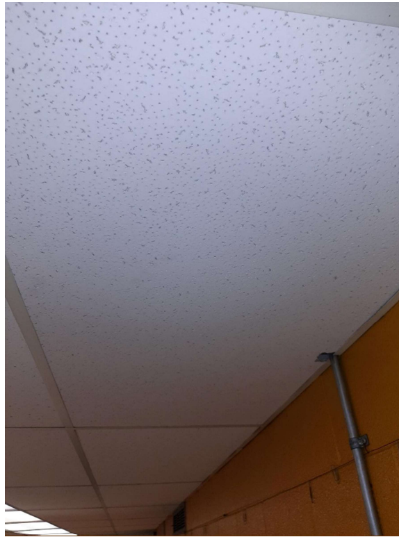
Photograph No. 9 – 2'x4' Small fissure random pinhole ceiling tiles were observed in Room 112. These tiles have a 04/02/11 date stamp and are not considered asbestos-containing; however, a mixture of asbestos and non-asbestos tiles are present throughout the room.
