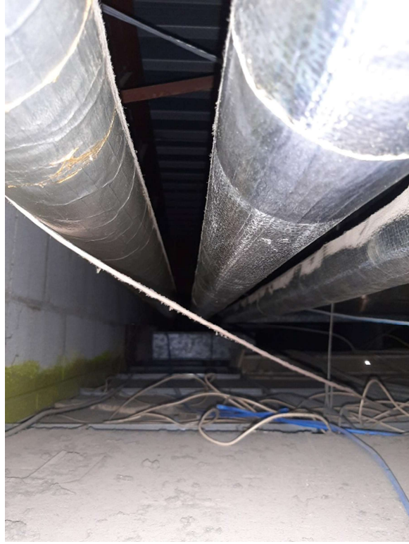
Photograph No. 7 – Foil wrapped fiberglass pipe straights were observed above drop ceilings.
