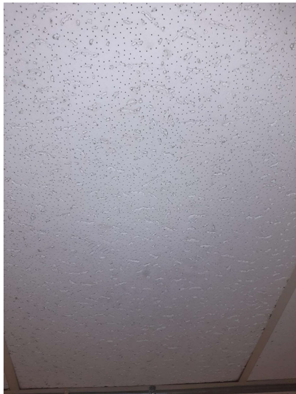
Photograph No. 8 – 2'x4' Large fissure random pinhole ceiling tiles were observed in Room 112 and were sampled (S05A,B,C). The ceiling tiles are non-asbestos; however, a mixture of asbestos and non-asbestos tiles are present throughout the room.
