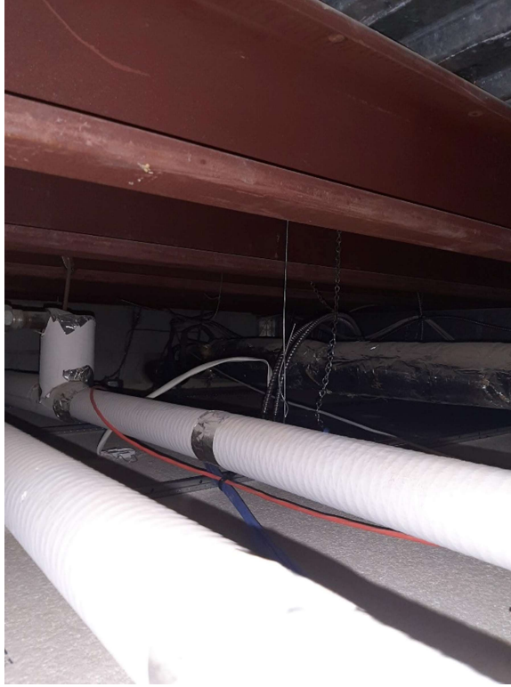
Photograph No. 7 – Non-asbestos fiberglass pipe insulation was observed above the drop ceiling in the second floor corridor
