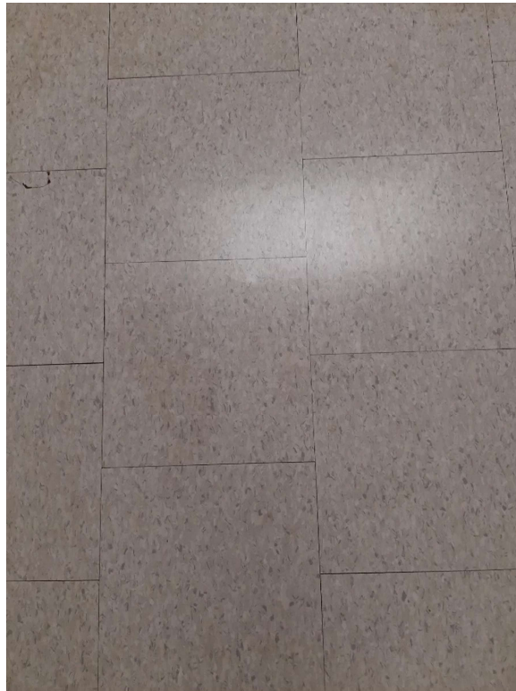
Photograph No. 5 – 12”x12” grey with white and grey oatmeal pattern vinyl floor tiles observed in the second floor corridor were sampled (S06A,B,C). The vinyl floor tiles and associated mastic are non-asbestos.
