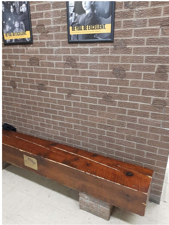
Photograph No. 4 – The bench brick mortar was sampled (S04A,B,C) and is non-asbestos.
