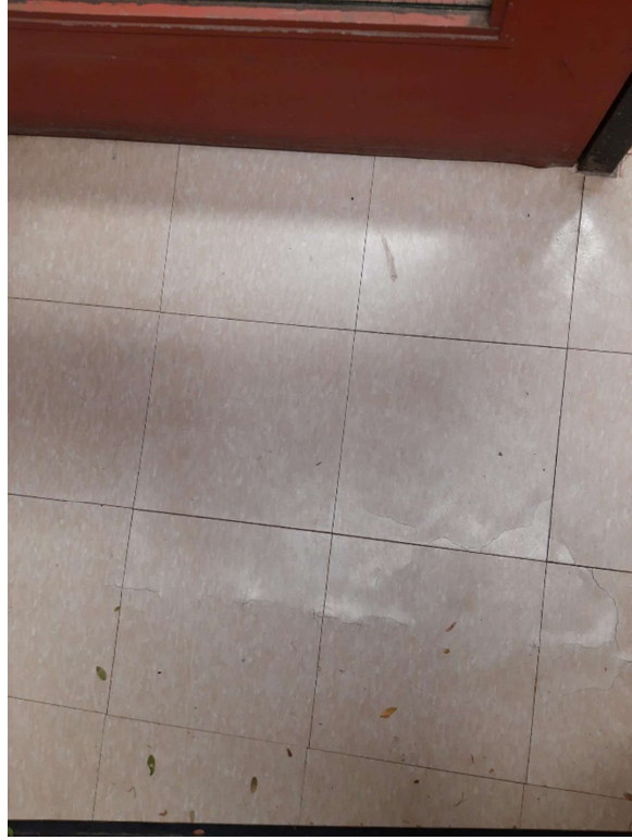
Photograph No. 3 – 12”x12” Brown with white fleck vinyl floor tile was observed in Vestibule 115 and was sampled (S03A,B,C). The vinyl floor tile and associated mastics are non-asbestos.
