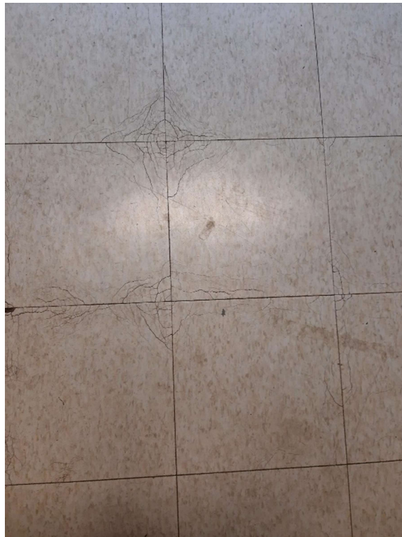
Photograph No. 2 – 12”x12” White with beige fleck vinyl floor tile observed in Vestibules 107, 124, and 130 was sampled (S02A,B,C). The vinyl floor tile and associated mastics are non-asbestos.
