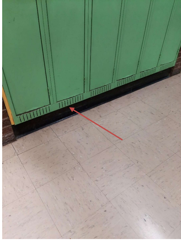
Photograph No. 5 – The vinyl baseboard observed in the corridors was sampled (S05A,B,C). The baseboard and associated mastics are non-asbestos.
