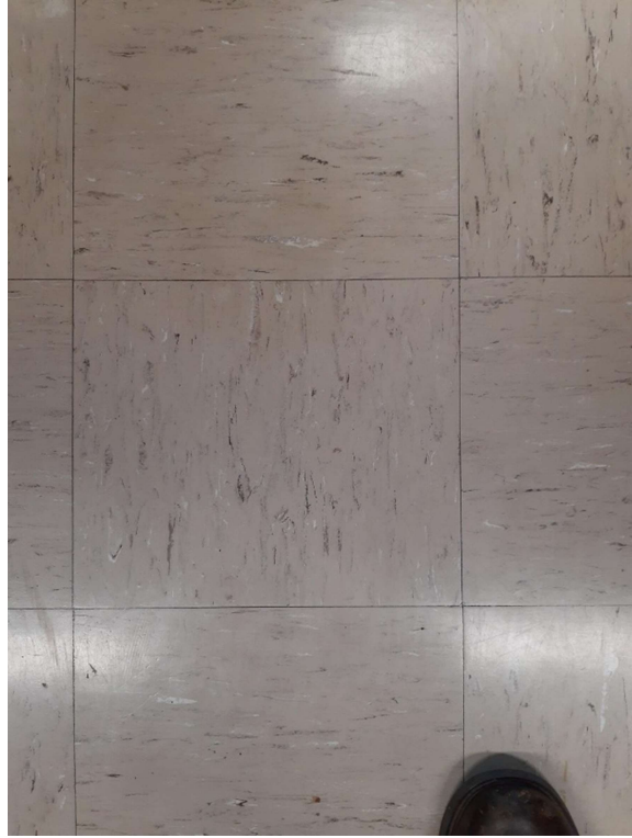
Photograph No. 1 – 12”x12” Brown with black and white fleck vinyl floor tile was observed throughout the corridors and was sampled (S01A,B,C). The vinyl floor tile is asbestos-containing; however, the associated mastic is non-asbestos.
