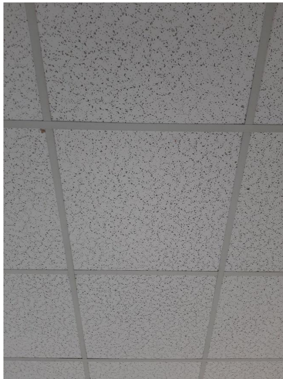
Photograph No. 6 – 2'x2' Small fissure random pinhole ceiling tile was observed within the main corridor and was sampled (S04A,B,C). The ceiling tile is non-asbestos.
