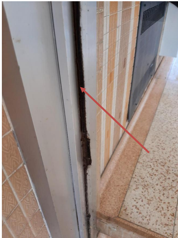
Photograph No. 2 – A small amount of black glazing was observed on the windows at the main entrance. The black glazing was sampled (S06A,B,C) and is asbestos-containing.
