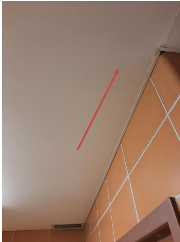
Photograph No. 1 – Drywall was observed on the ceiling of Washroom 1059.1059A, and 1059B. The compound was sampled (S02A,B,C) and is asbestos-containing.
