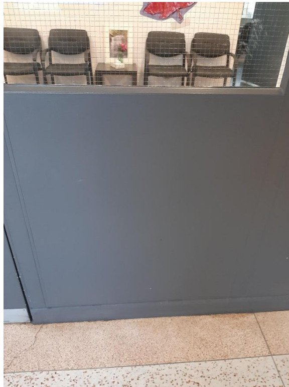
Photograph No. 8 – Grey paint was observed on the main office doors/frames and was sampled (LP05). The paint is low level lead-containing.
