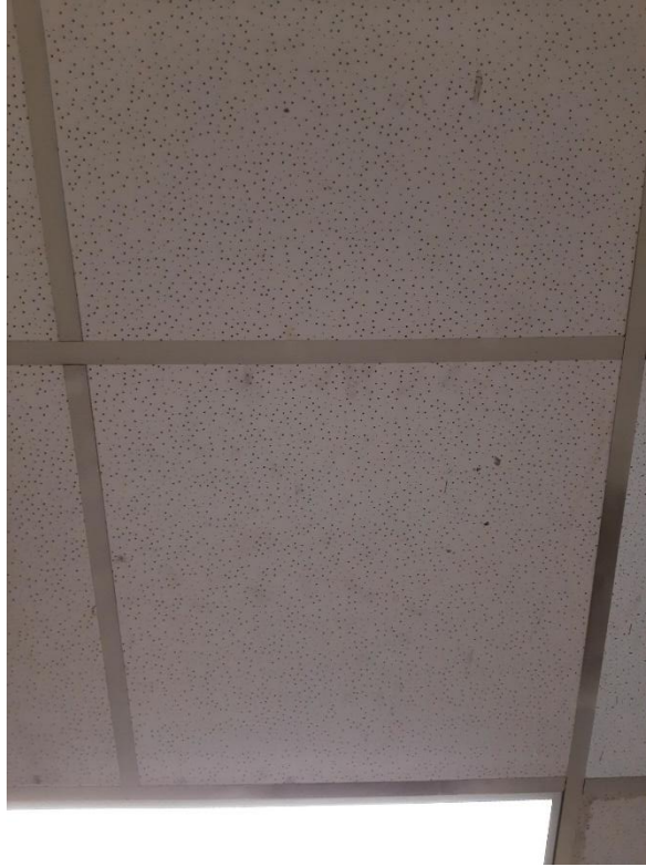
Photograph No. 5 – 2'x2' Random pinhole ceiling tile was observed within the main corridor and was sampled (S03A,B,C). The ceiling tile is non-asbestos.
