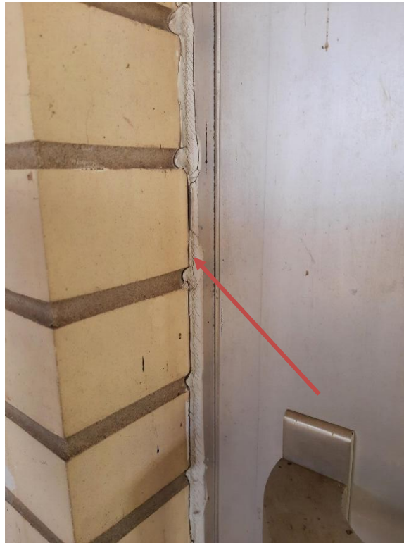
Photograph No. 3 – White sealant was observed on the exterior of the main entrance and was sampled (S08A,B,C). The white sealant is asbestos-containing. It was also analyzed for PCB content (PCB-2) and is non-PCB.
