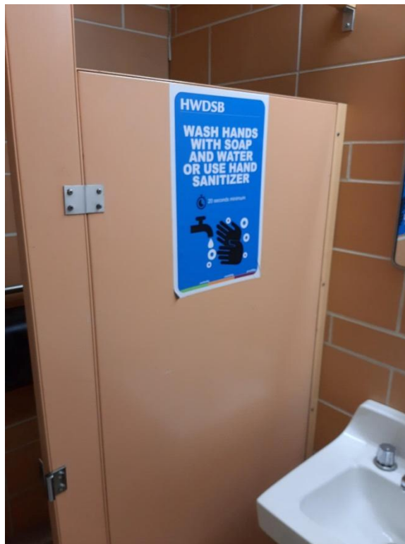
Photograph No. 4 – The orange paint observed on the stalls within Washroom 1059 was sampled (LP02) and is lead-containing.
