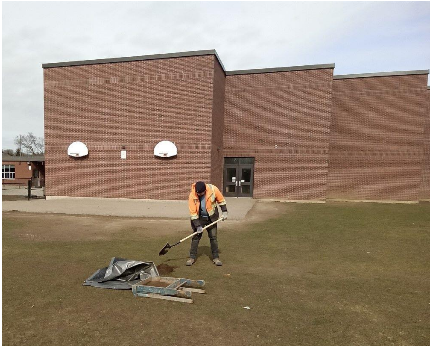
Image 1: View of school building with associated paved areas adjacent; test pit survey in progress.
