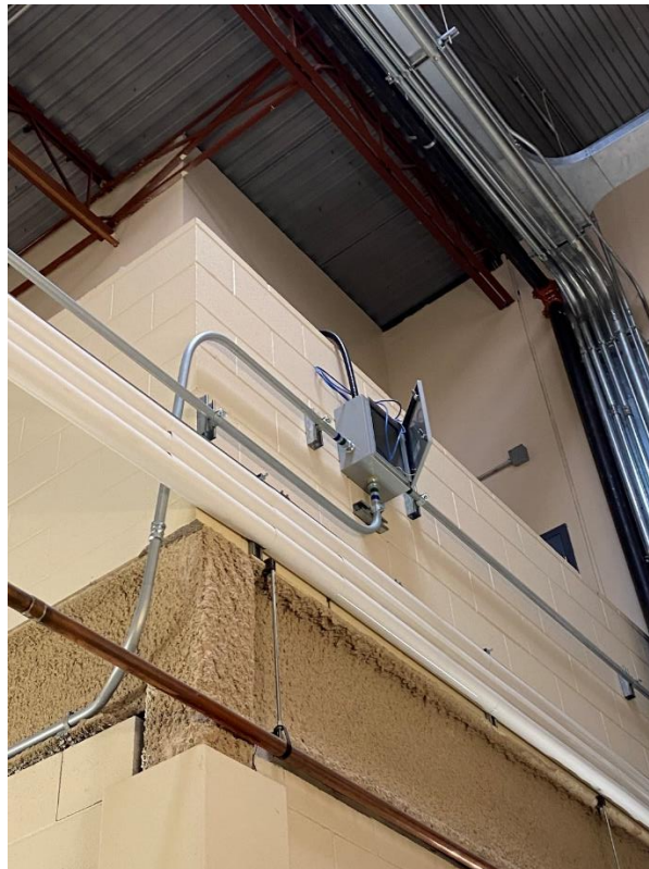
Picture 6: Black Flexible Conduit from Junction Box to Camera Location: First Floor Exterior Stair Corridor Wall by B140 Drawing Reference: DWG 505 Note 19
