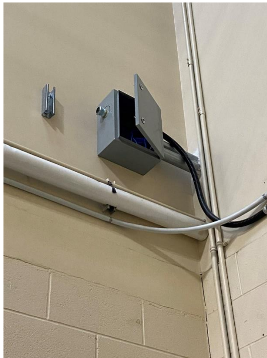
Picture 4: Junction Box with Punchout Location: First Floor Corridor by C168 Drawing Reference: DWG 505 Note 18
