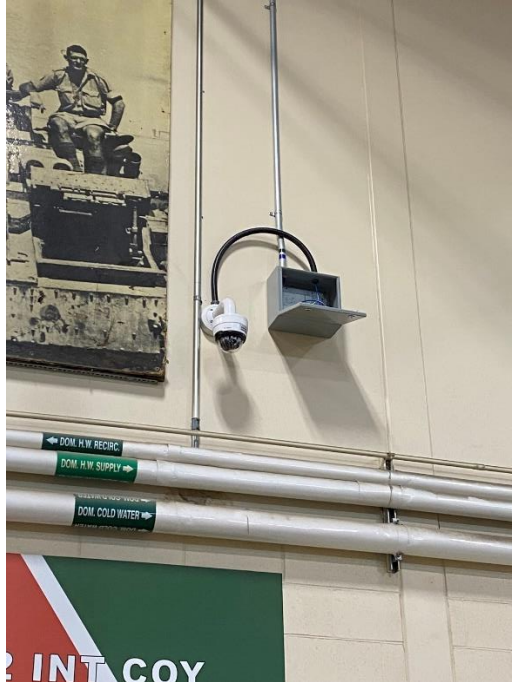
Picture 3: Junction Box Placed in the Incorrect Orientation Location: First Floor Above Double Doors to C164 Drawing Reference: DWG 505 Note 20
