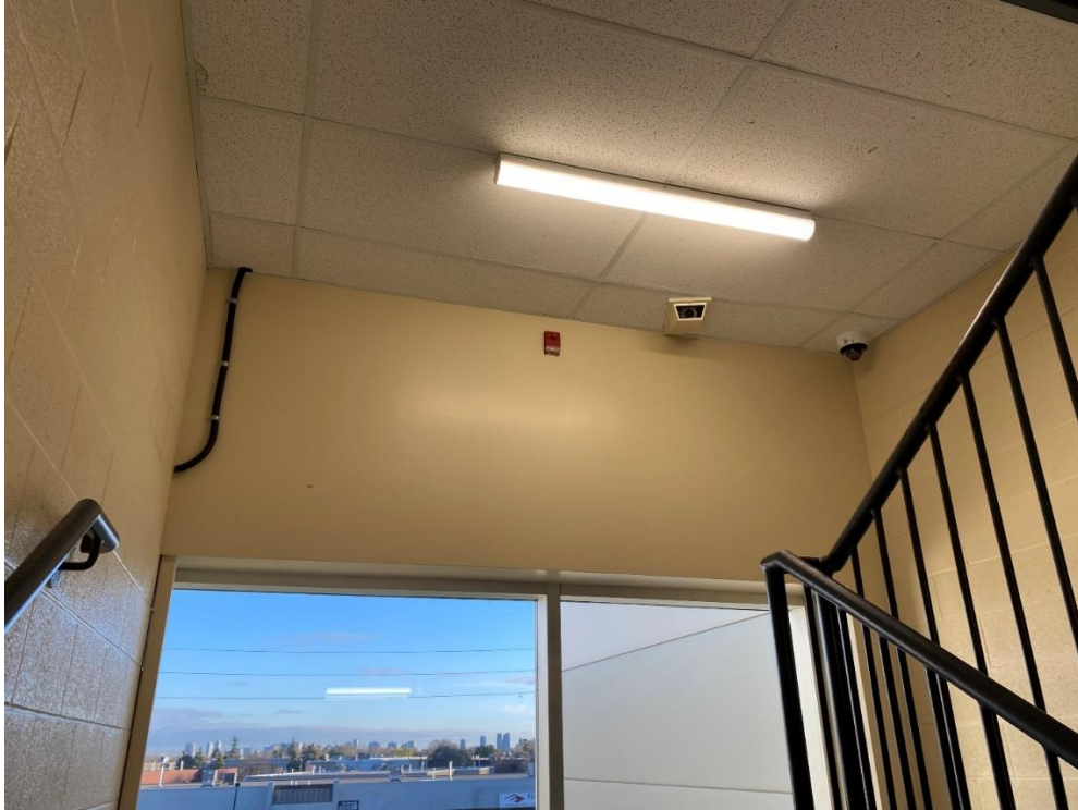
Picture 15: Black Flexible Conduit from Junction Box to Camera Location: 2 nd Floor Stair #2 Drawing Reference: DWG 507 Note 13
