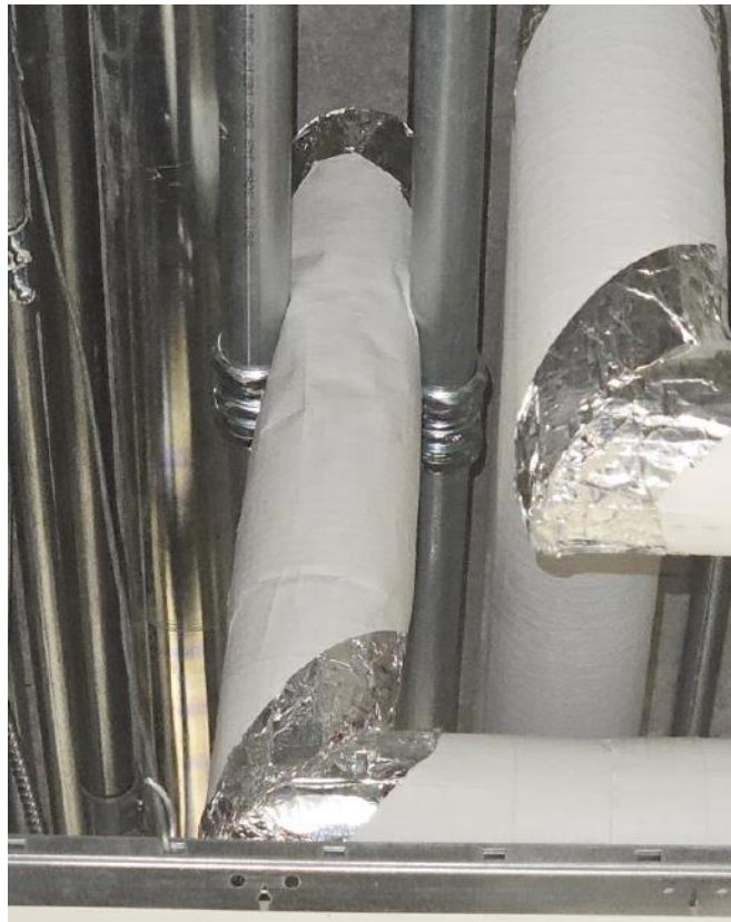
Picture 2: Existing Conduit installed against Plumbing Pipe Location: Basement Corridor Drawing Reference: DWG 504 Note 15
