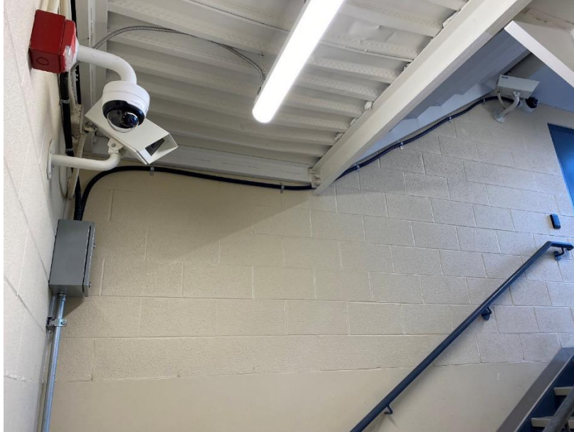
Picture 1: Black Flexible Conduit from Junction Box to Camera at the door Location: Basement Stair #2 Drawing Reference: DWG 504 Note 14
