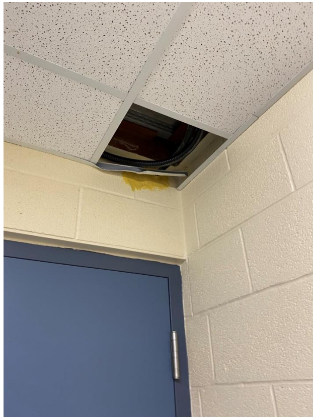
Picture 14: Flex Conduit Not Connected to Camera Location: 2 nd Floor Stair #3 Drawing Reference: DWG 507 Note 12
