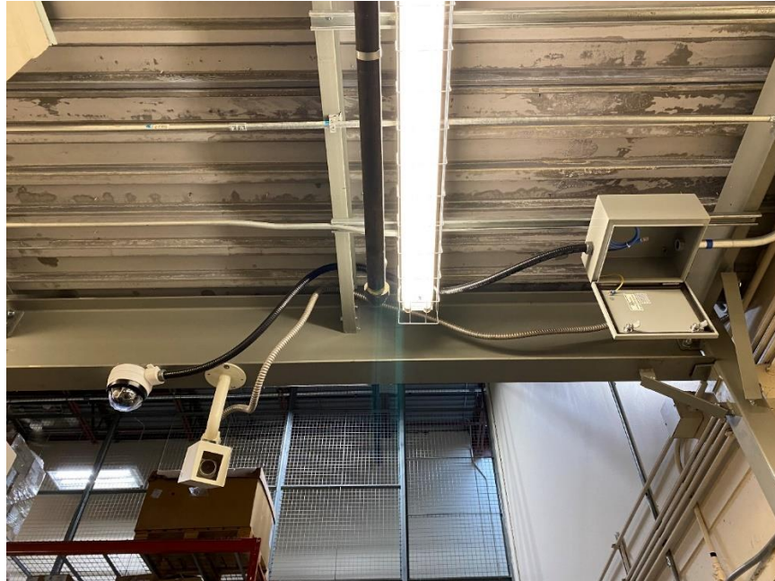
Picture 5: Black Flexible Conduit from Junction Box to Camera Location: First Floor C156 Drawing Reference: DWG 505 Note 19
