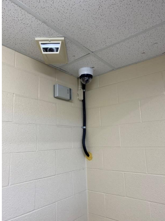
Picture 11: Black Flexible Conduit from Junction Box to Camera Location: First Floor Stair #2 Drawing Reference: DWG 506 Note 14
