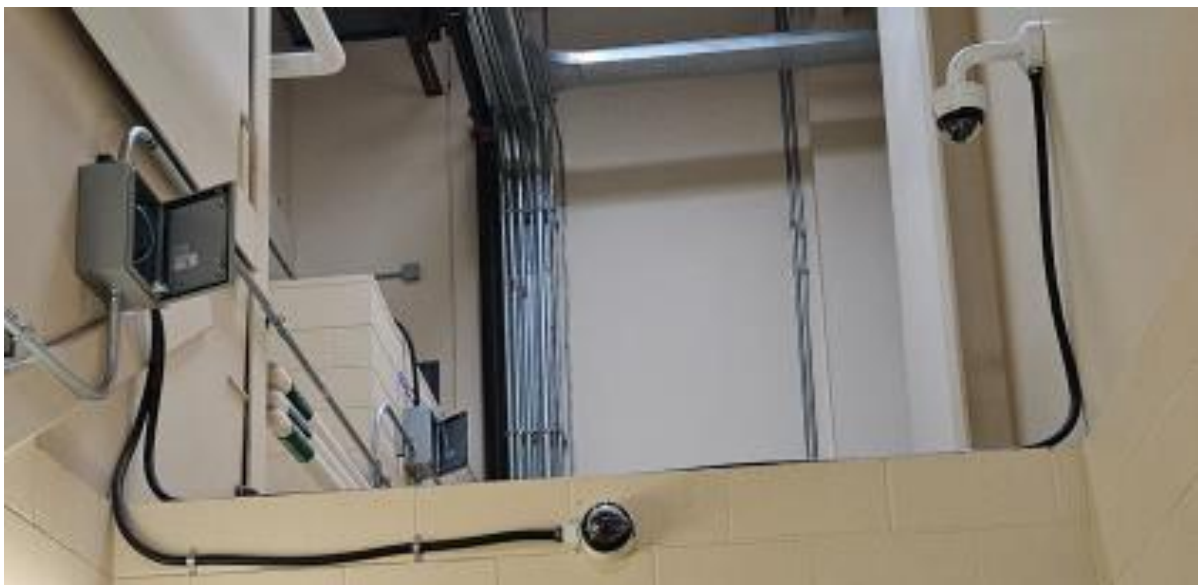
Picture 8: Black Flexible Conduit from Junction Box to Camera Location: First Floor Double Doors by C174B Drawing Reference: DWG 505 Note 19
