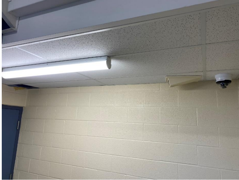
Picture 13: Flex Conduit Not Connected to Camera Location: 2 nd Floor Stair #3 Drawing Reference: DWG 507 Note 12
