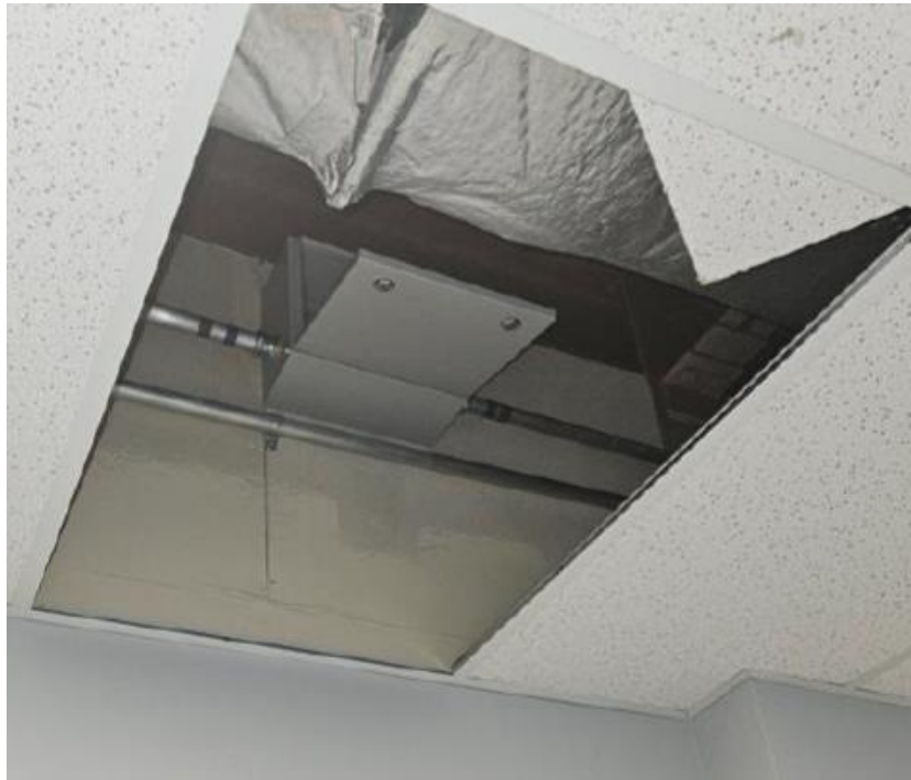
Picture 16: Incorrect Junction Box Orientation Location: 3 rd Floor Corridor Drawing Reference: DWG 508 Note 16
