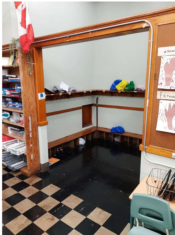
Photograph No. 6 – The green paint observed in Classroom 211 and Storage room 108C was sampled (LP02) and is lead-containing.
