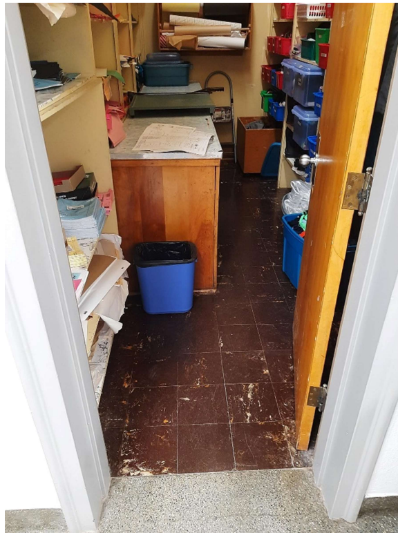
Photograph No. 8 – 9”x9” Brown with beige marble pattern vinyl floor tiles were observed in storage Room 116 and was sampled (S07A,B,C). The vinyl floor tiles are asbestos-containing; however, the associated mastic is non-asbestos.
