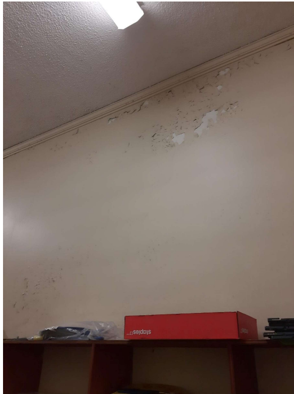
Photograph No. 5 – The yellow paint observed in Classroom 203 was sampled (LP03) and is lead-containing.
