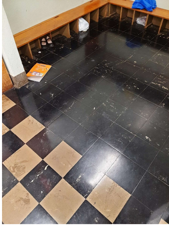
Photograph No. 1 – 9”x9” Green/beige and black with beige marble pattern vinyl floor tiles were observed in Classrooms 203 and 211. The tiles were sampled (S01A,B,C) and found to be asbestos-containing. The associated mastic is also asbestos-containing.
