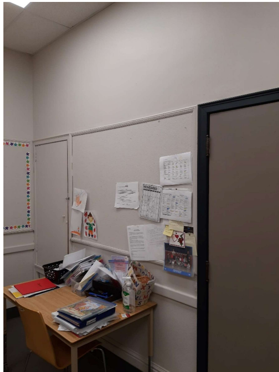
Photograph No. 9 – Potentially concealed asbestos-containing mastics may be present underneath corkboards.
