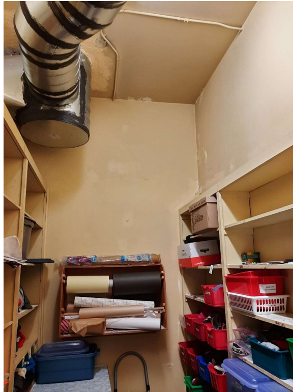
Photograph No. 8 – The yellow paint observed within storage Room 116 was sampled (LP4) and is lead-containing.
