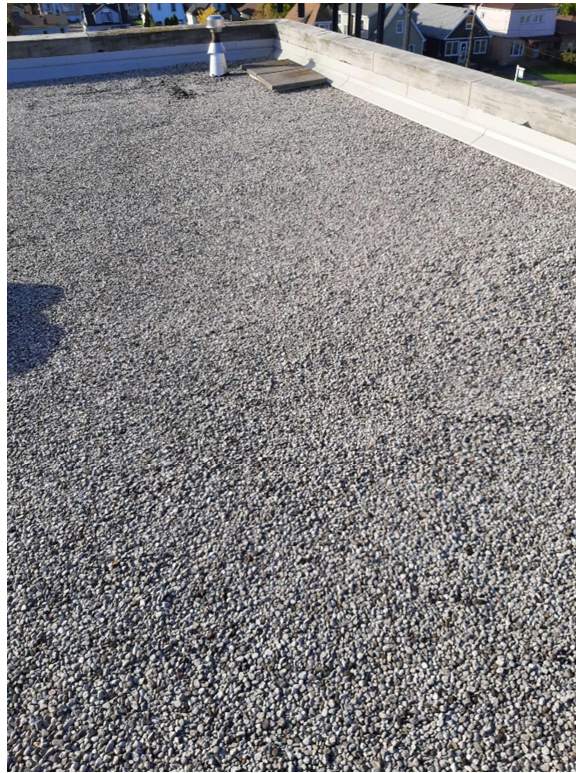
Photograph No. 7 – The roof system was sampled (S04A,B,C / S05A,B,C / S06A,B,C) and is non-asbestos.
