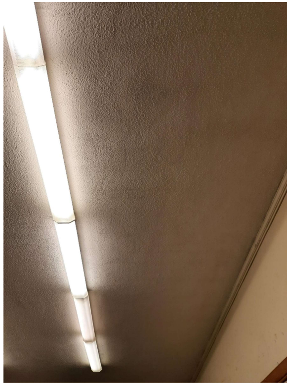
Photograph No. 2 – A texture coat ceiling was observed throughout the interior and was sampled (S03A,B,C,D,E,F,G). The texture coat ceiling is asbestos-containing.
