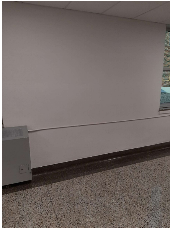
Photograph No. 3 – Plaster walls were observed throughout the interior. The plaster was sampled (S02A-G) and is non-asbestos.
