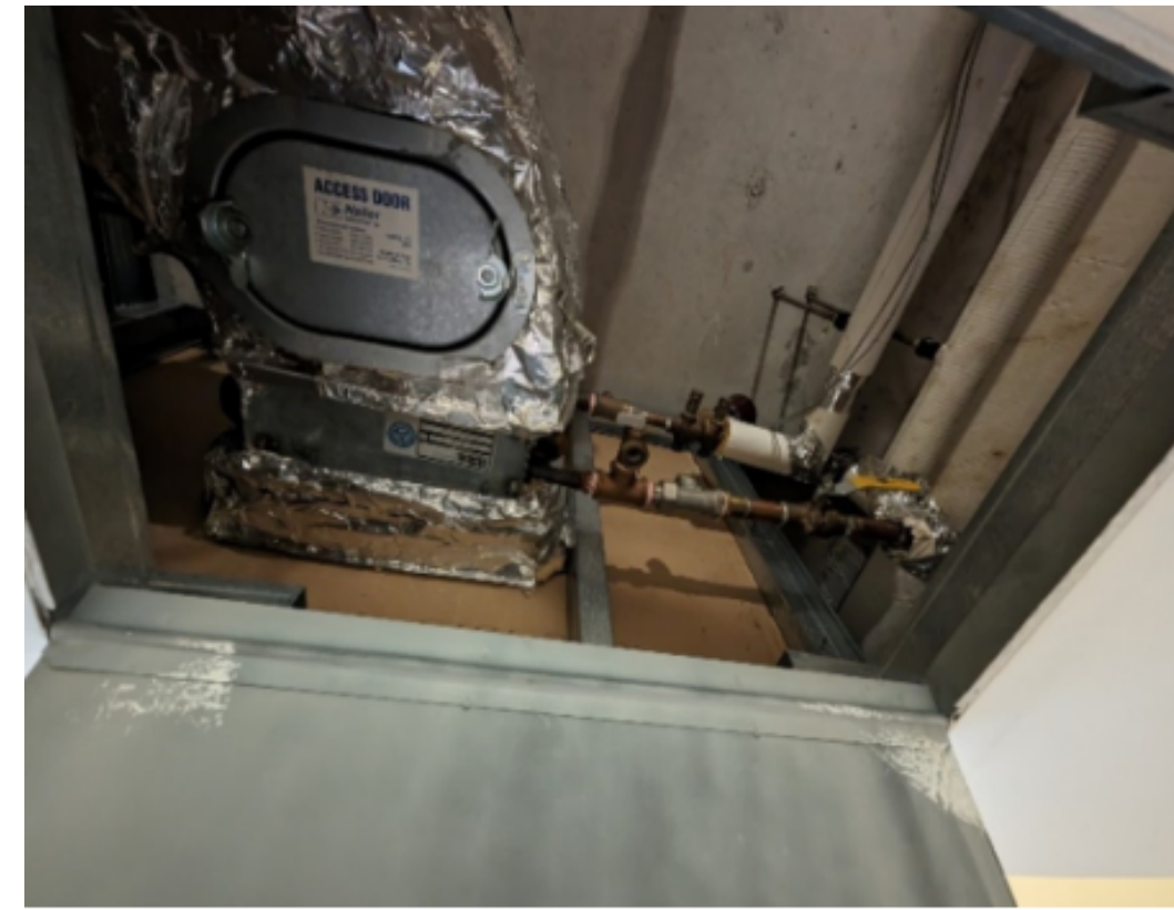
ECP-01: DUCTWORK REHEAT COIL WITHIN CEILING
