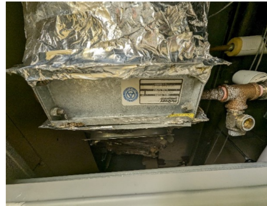
ECP-02: DUCTWORK REHEAT COIL WITHIN CEILING
