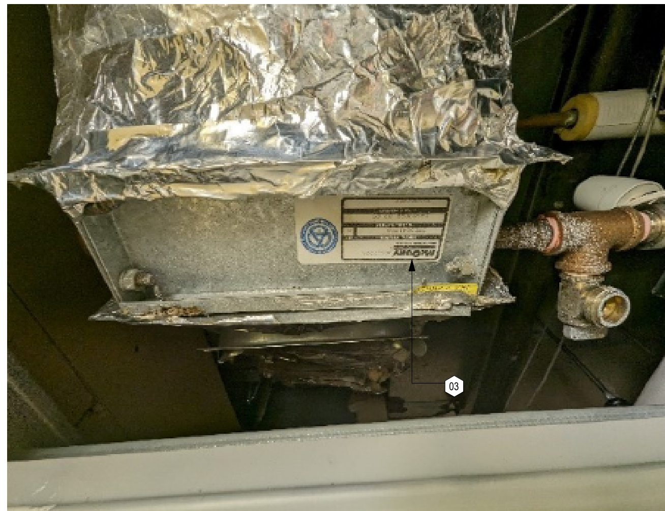
ECP-19: REHEAT COIL IN CEILING SPACE
