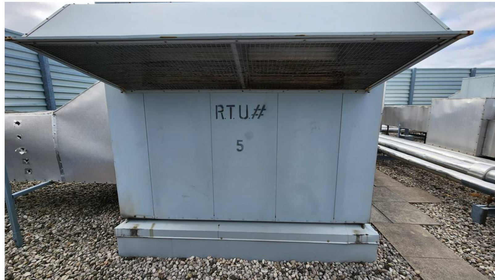
ECP #12_TYPICAL RTU
