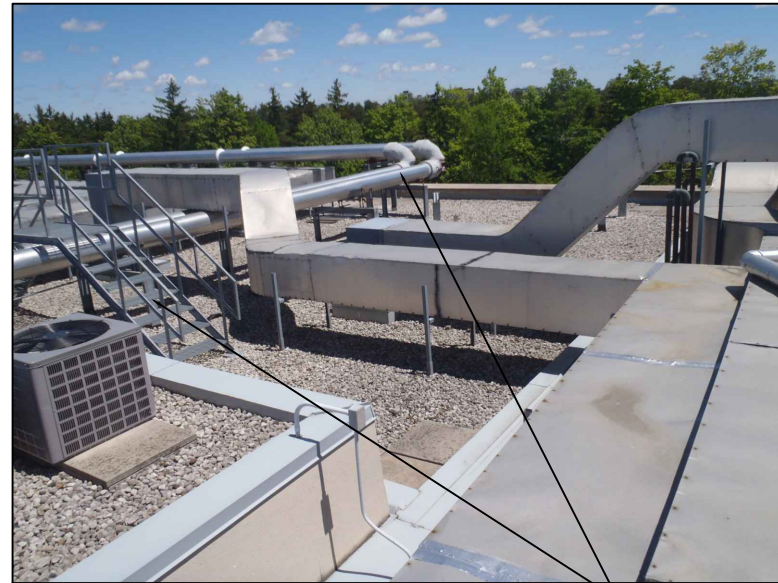
2 PHOTOGRAPH OF EXISTING DUCT OVERPASS AND PIPING PROTECT ALL OVERPASS AND PIPING INSULATION FROM DAMAGE M-6.0 N.T.S.
