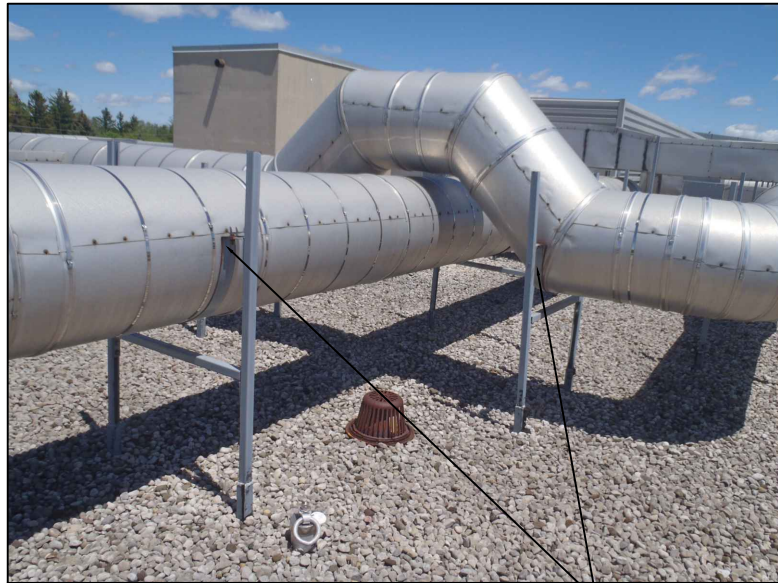
1 PHOTOGRAPH OF EXISTING DUCT AND SUPPROTS PROTECT ALL ROUND DUCT SUPPORTS FROM DAMAGE M-6.0 N.T.S.
