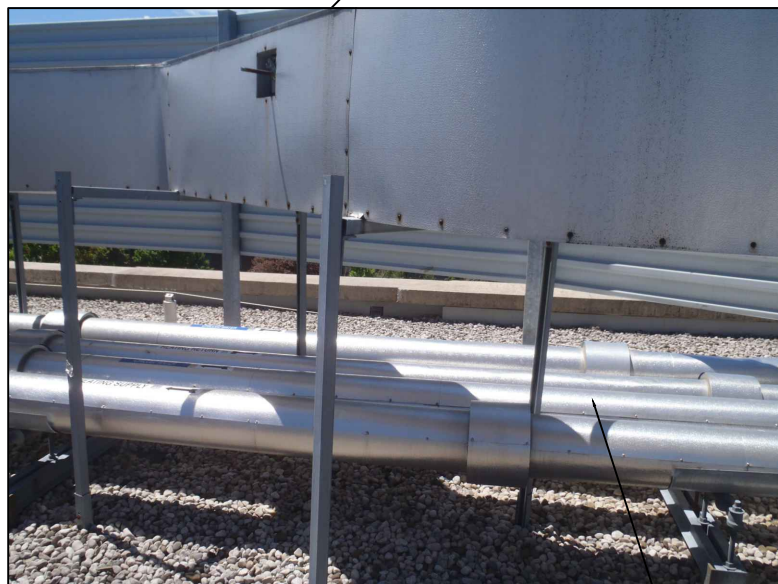
4 PHOTOGRAPH OF EXISTING DUCT ACCESSORIES AND PIPING PROTECT PIPING INSULATION FROM DAMAGE M-6.0 N.T.S.
