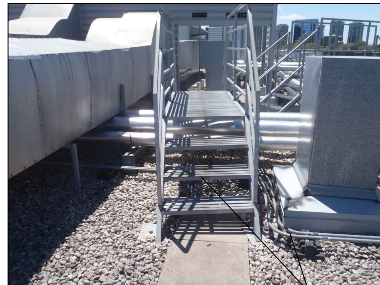
6 PHOTOGRAPH OF EXISTING OVERPASS AND ROOF CURB PROTECT OVERPASS AND CONDUITS FROM DAMAGE M-6.0 N.T.S.
