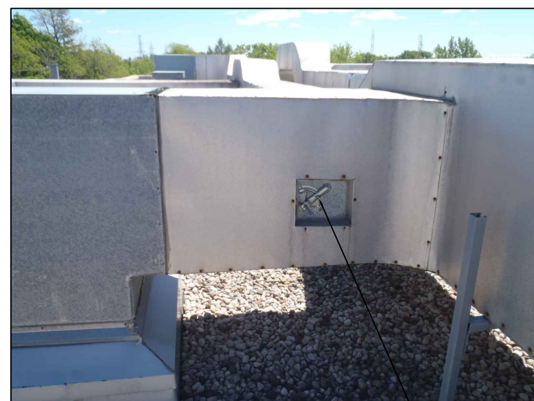
8 PHOTOGRAPH OF EXISTING CONTROL ACCESSORIES PROTECT CONTROL ACCESSORIES FROM DAMAGE M-6.0 N.T.S.
