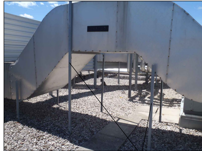
3 PHOTOGRAPH OF EXISTING DUCT SUPPORT PROTECT ALL RECTANGULAR DUCT SUPPORTS FROM DAMAGE M-6.0 N.T.S.
