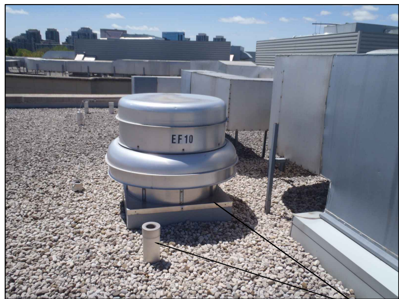
7 PHOTOGRAPH OF EXISTING EXHAUST FAN AND PLUMBING STACK PROTECT EQUIPMENT AND PLUMBING STACK FROM DAMAGE M-6.0 N.T.S.
