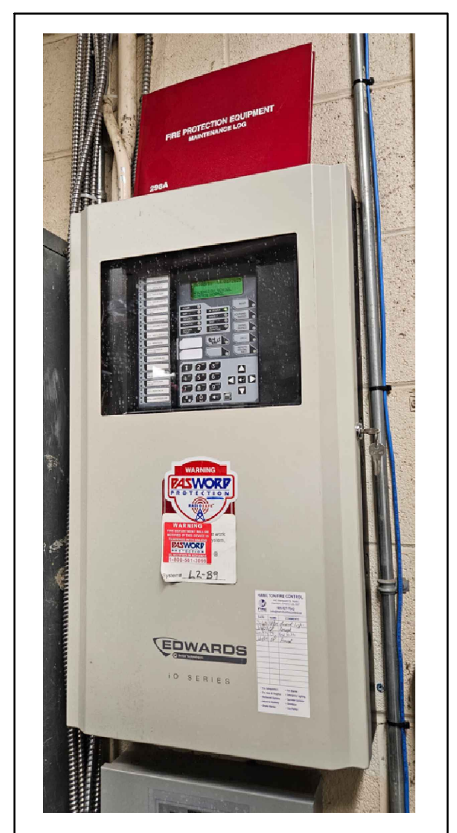
EXISTING FIRE ALARM PANEL
