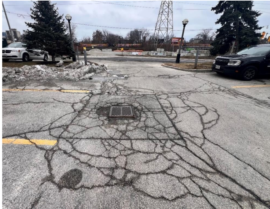
Figure 1: Parking Lot Entrance from Macpherson Ave, Facing South. Extensive, severe longitudinal and transverse cracking. Frequent, moderate to severe alligator cracking. Frequent, moderate shoving. Extensive, slight to moderate coarse aggregate loss and raveling. Frost heave settlement and associated cracking around catch basin, moderate to severe random cracking along catch basin. [RG, January 2024]
