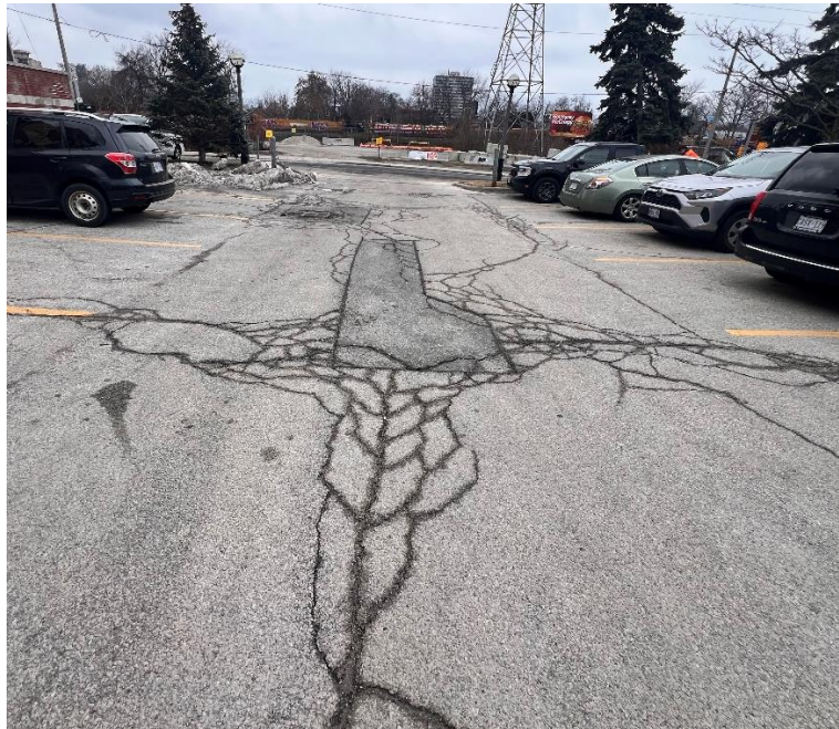
Figure 8: Facing South. Extensive, severe longitudinal and transverse cracking. Extensive, slight to moderate random cracking. Frequent, slight to moderate segregation. Extensive, slight to moderate coarse aggregate loss and raveling. Intermittent, slight to moderate wheel track rutting. Asphalt patch in poor to fair condition and moderate patch boundary deterioration. [RG, January 2024]
