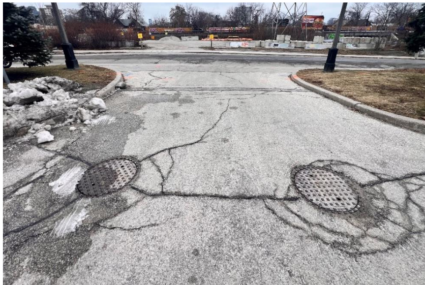
Figure 2: Parking Lot Entrance from Macpherson Ave, Facing South. Frequent, Moderate longitudinal and transverse cracking. Frequent, moderate shoving. Extensive, slight to moderate coarse aggregate loss and raveling. Frost heave settlement and associated cracking around maintenance access holes, moderate to severe random cracking along maintenance access holes. [RG, January 2024]
