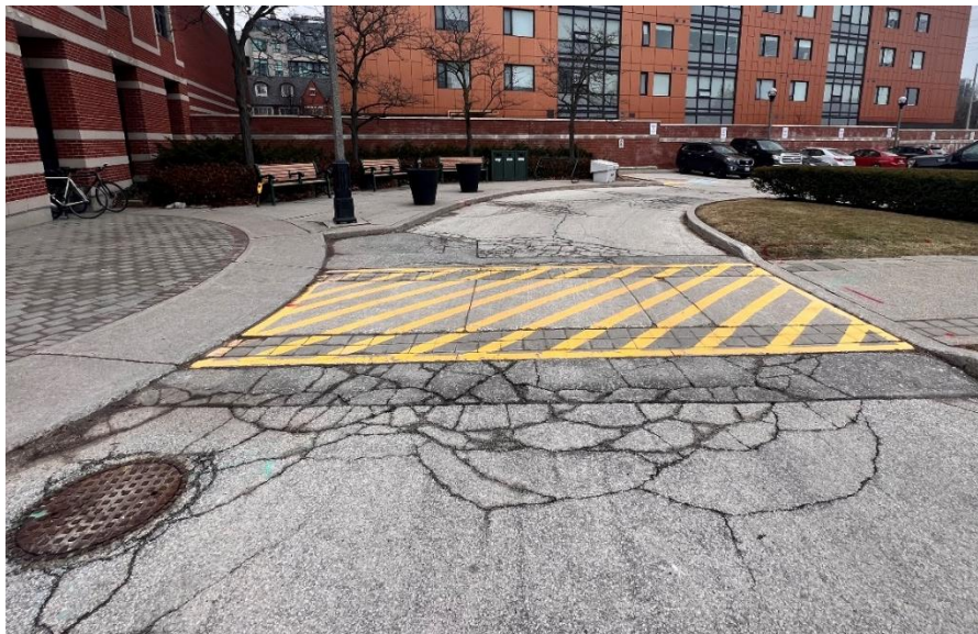
Figure 4: Infront of the main building entrance, Facing South-East. Extensive, severe longitudinal and transverse cracking. Frequent, moderate to severe alligator cracking. Extensive, moderate to severe random cracking. Frequent, moderate to severe segregation. Extensive, moderate to severe coarse aggregate loss and raveling. Asphalt patch in poor to fair condition and moderate patch boundary deterioration. [RG, January 2024]
