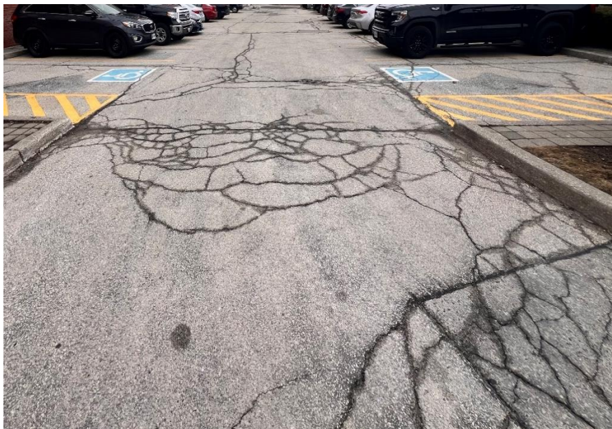
Figure 6: Facing South. Extensive, moderate to severe longitudinal and transverse cracking. Frequent, moderate to severe alligator cracking. Frequent, moderate to severe segregation. Frequent, slight to moderate shoving. Extensive, slight to moderate coarse aggregate loss and raveling. [RG, January 2024]
