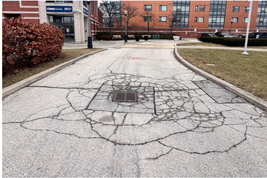
Figure 3: Parking Lot Entrance from Spadina Ave, Facing East. Frequent, moderate to severe alligator cracking. Extensive, slight to moderate coarse aggregate loss and raveling. Frost heave settlement and associated cracking around catch basin, moderate to severe random cracking along catch basin. Asphalt patch in poor to fair condition and moderate patch boundary deterioration. [RG, January 2024]
