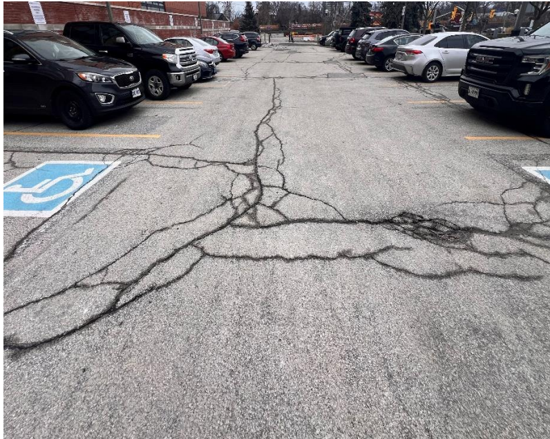
Figure 7: Facing South. Extensive, severe longitudinal and transverse cracking. Frequent, slight to moderate segregation. few, slight to moderate distortions/shoving. Extensive, moderate to severe coarse aggregate loss and raveling with pothole formation. Intermittent, slight to moderate wheel track rutting. [RG, January 2024]
