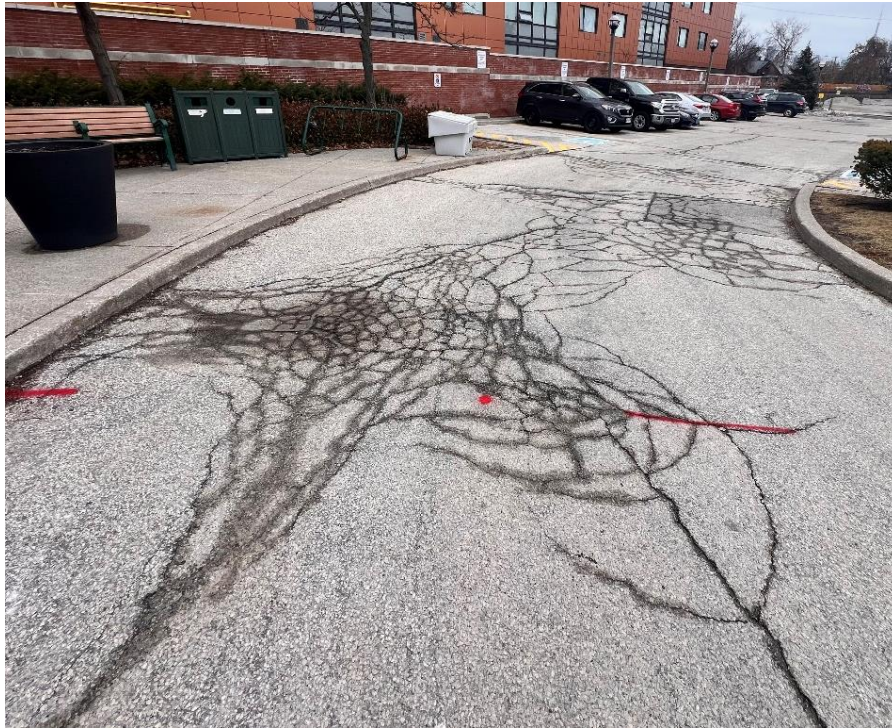
Figure 5: Facing South. Extensive, moderate to severe longitudinal and transverse cracking. Frequent, moderate to severe alligator cracking. Extensive, moderate to severe random cracking. Intermittent, moderate to severe edge of pavement cracking. Frequent, slight to moderate severe shoving. Extensive, slight to moderate coarse aggregate loss and raveling. [RG, January 2024]
