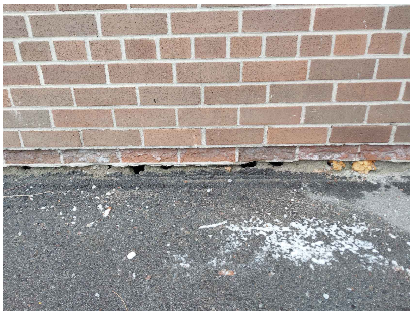
11. DETERIORATED BRICK CLADDING AND CONCRETE BLOCK FOUNDATION
