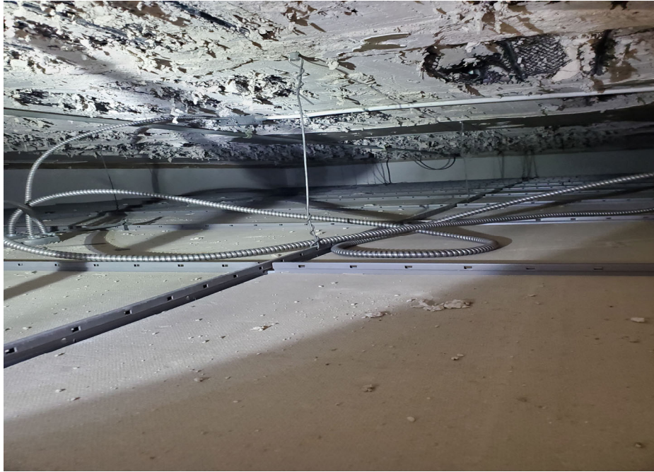
Location #350 (Stair) – Smooth plaster delaminated from lath, debris on lay-in ceiling
