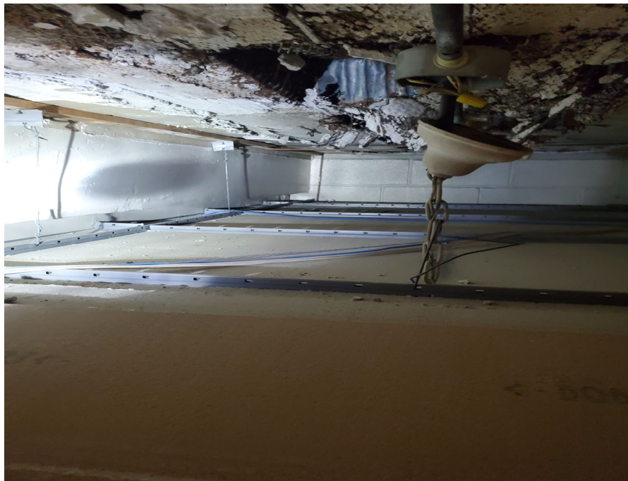
Location #332 (Classroom) – Smooth plaster delaminated from lath, debris on lay-in ceiling
