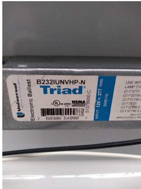
Photograph 9: View of a non-PCB containing light ballast observed at the Subject Location.
