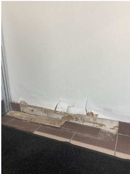
Photo 5: Water-damaged drywall on east wall prior to abatement (Loc. 1037)
