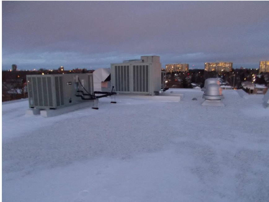
Photograph 10: View of the air handling units suspected to contain ozone depleting refrigerant observed on the roof at Subject Location.
