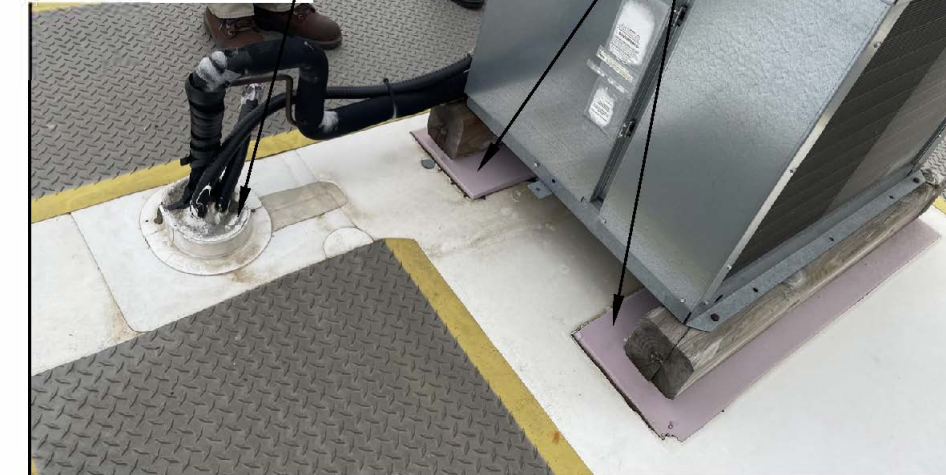
PHOTO 4: EXISTING AIR COOLED CONDENSING UNIT ON ROOF SERVING FREEZER 218
