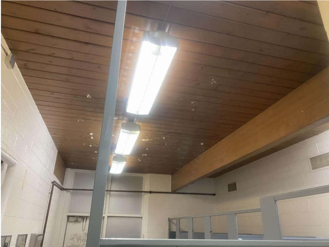
Mercury, V9500(Presumed), Mercury Vapour Lamp, Corridor (Location #: 5202)
