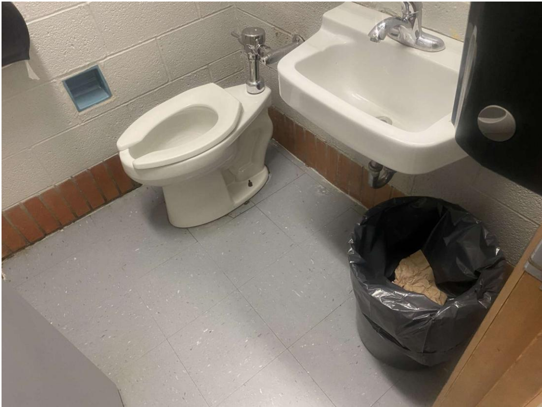
S0011C (None), grey, Floor, Caulking, Staff Washroom (Location #: 5197)
