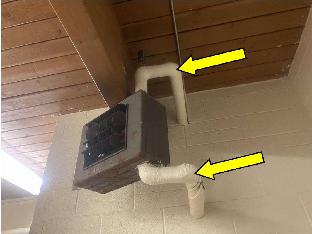
S0001A (Confirmed Asbestos), Piping, Parging Cement, Boy's Washroom (Location #: 5218)
