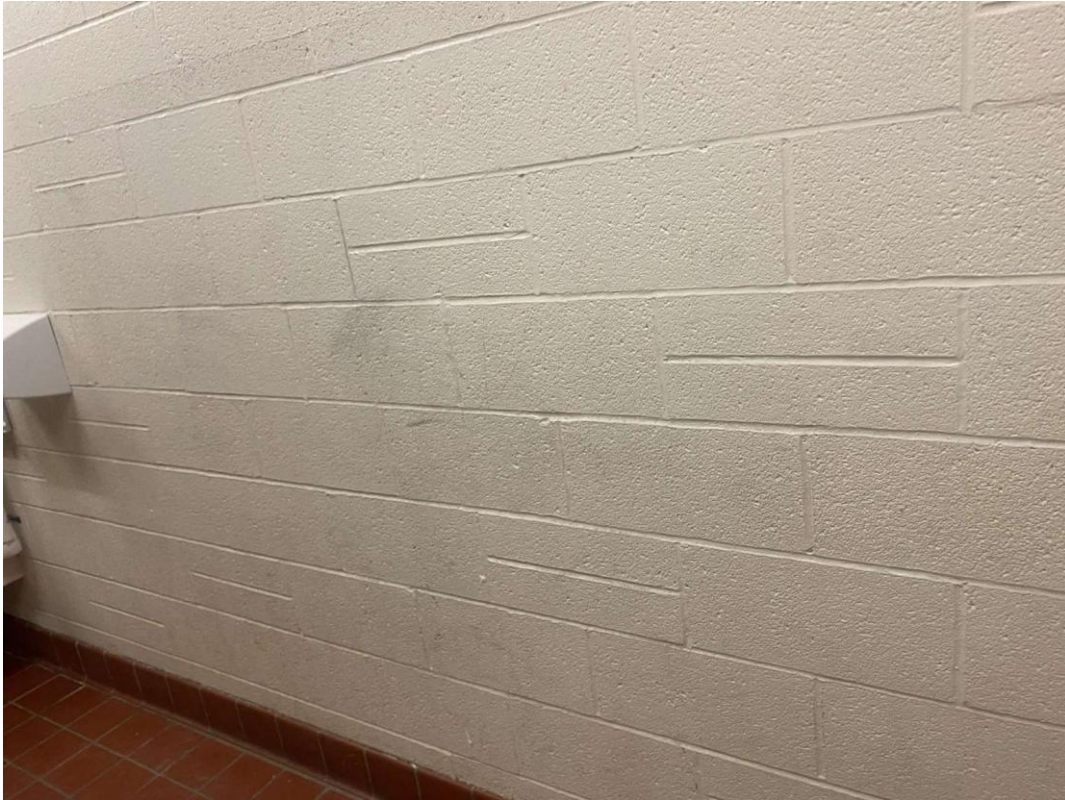
S0007A (None), On block, Wall, Paint, Boy's Washroom (Location #: 5218)
