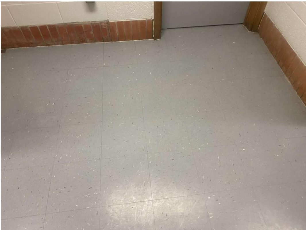
S0008A (None), 12x12 grey with white and black fleck, Floor, Vinyl Floor Tile and Mastic, Corridor (Location #: 5202)
