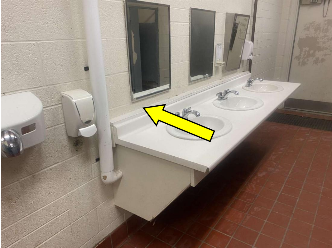
S0003A (None), White, Other, Caulking, Boy's Washroom (Location #: 5218)
