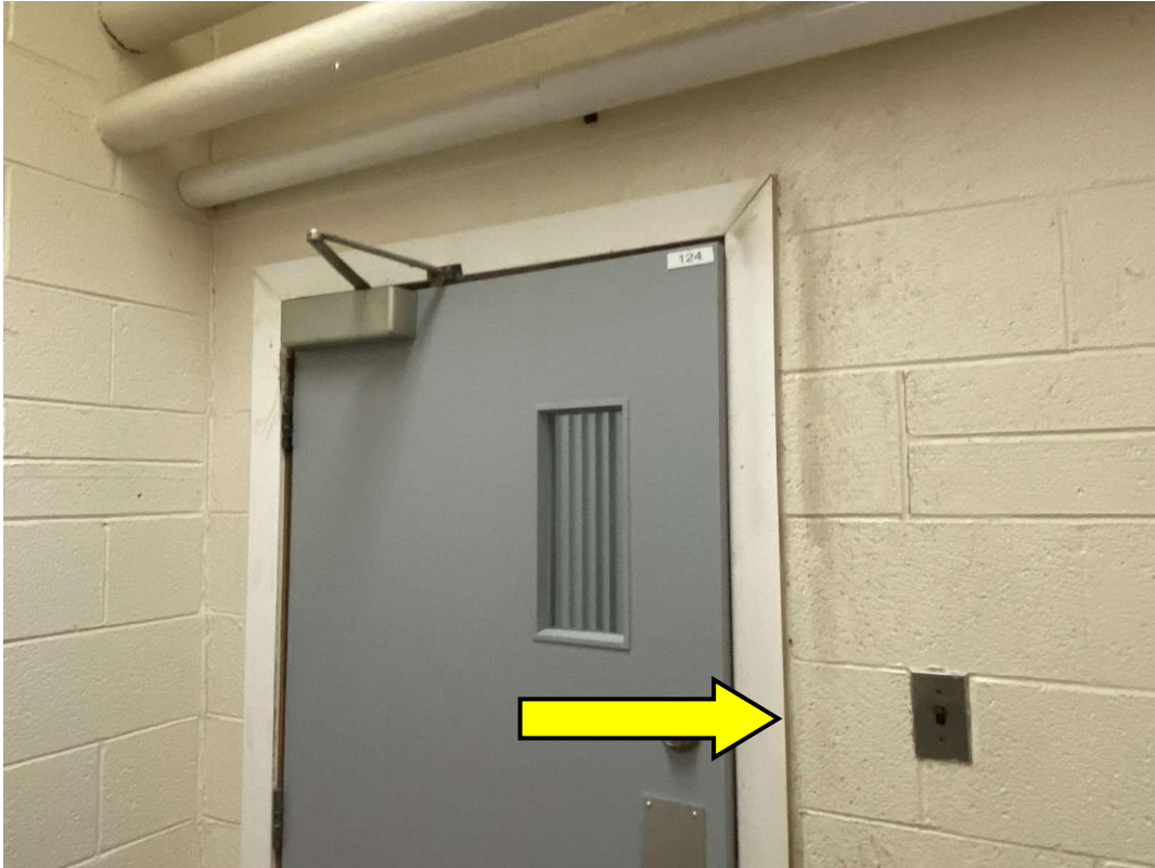
S0005A (None), White, Other, Door Frame, Caulking, Girls Washroom (Location #: 5216)
