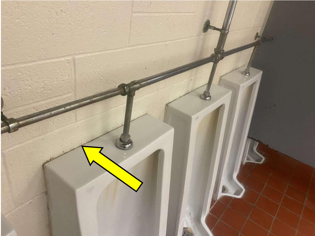
S0009A (None), White on urinal, Other, Caulking, Boys Washroom (Location #: 5189)
