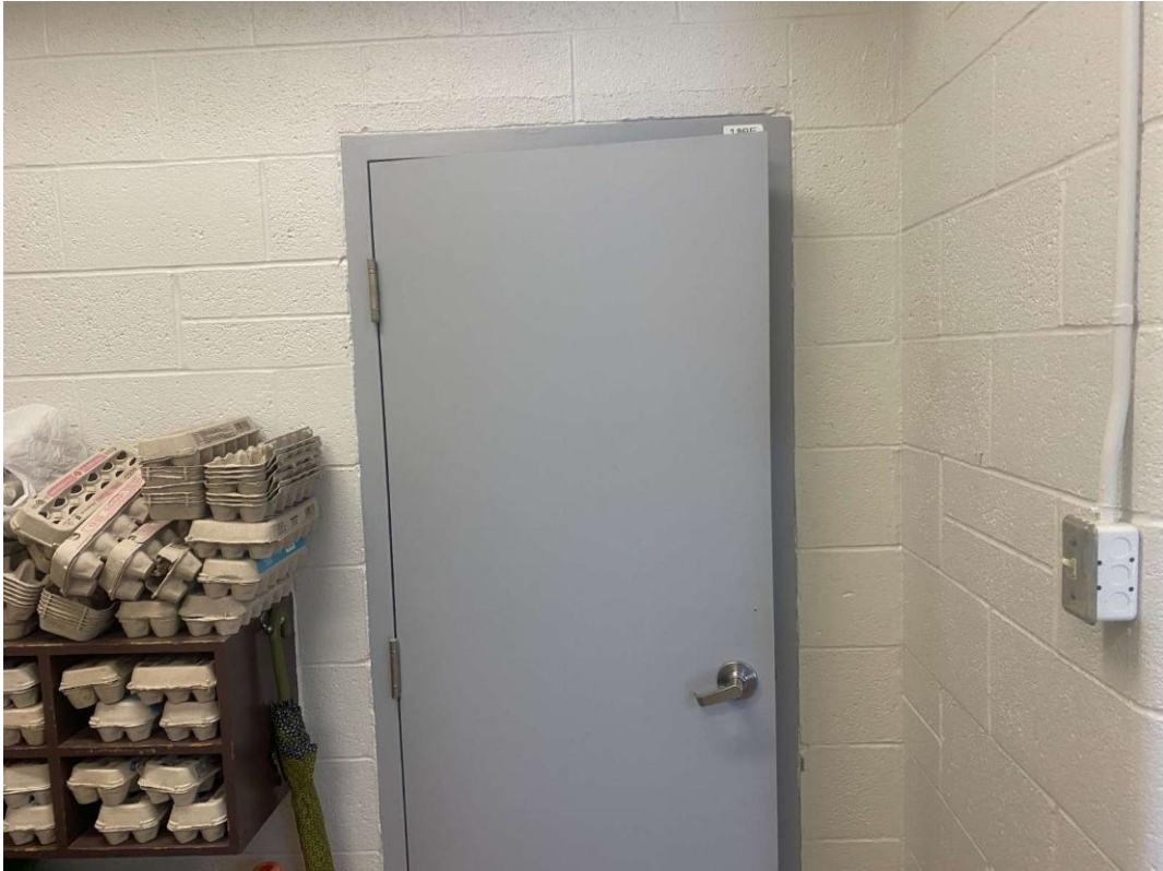
L0005(Lead, None), grey on door and frame, Other, Washroom (Location #: 5178)
