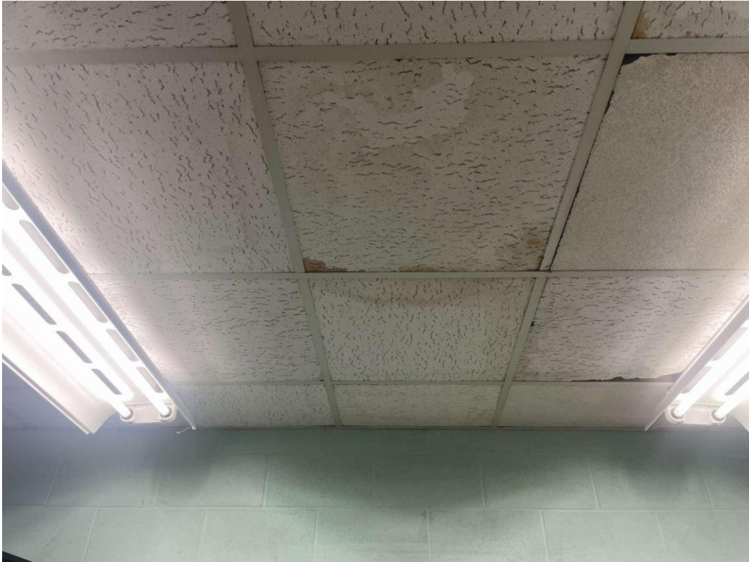
S0067A (Confirmed Asbestos), 24x24 pinhole and deep fissure, Ceiling, Ceiling Tiles (lay-in), Storage (Location #: 2376)
