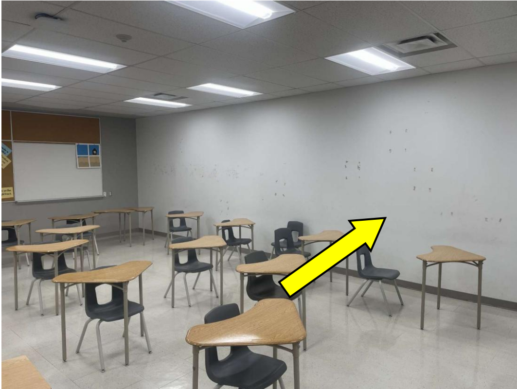
L0035(Lead, None), Paint on drywall, Wall, Classroom (Location #: 2570)
