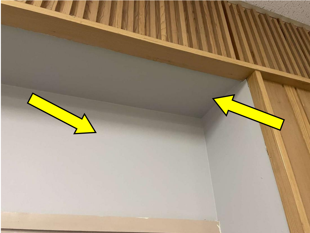
S0069A (Confirmed Asbestos), Wall, Bulkhead, Drywall and joint compound, Teacher Workstation (Location #: 2379)
