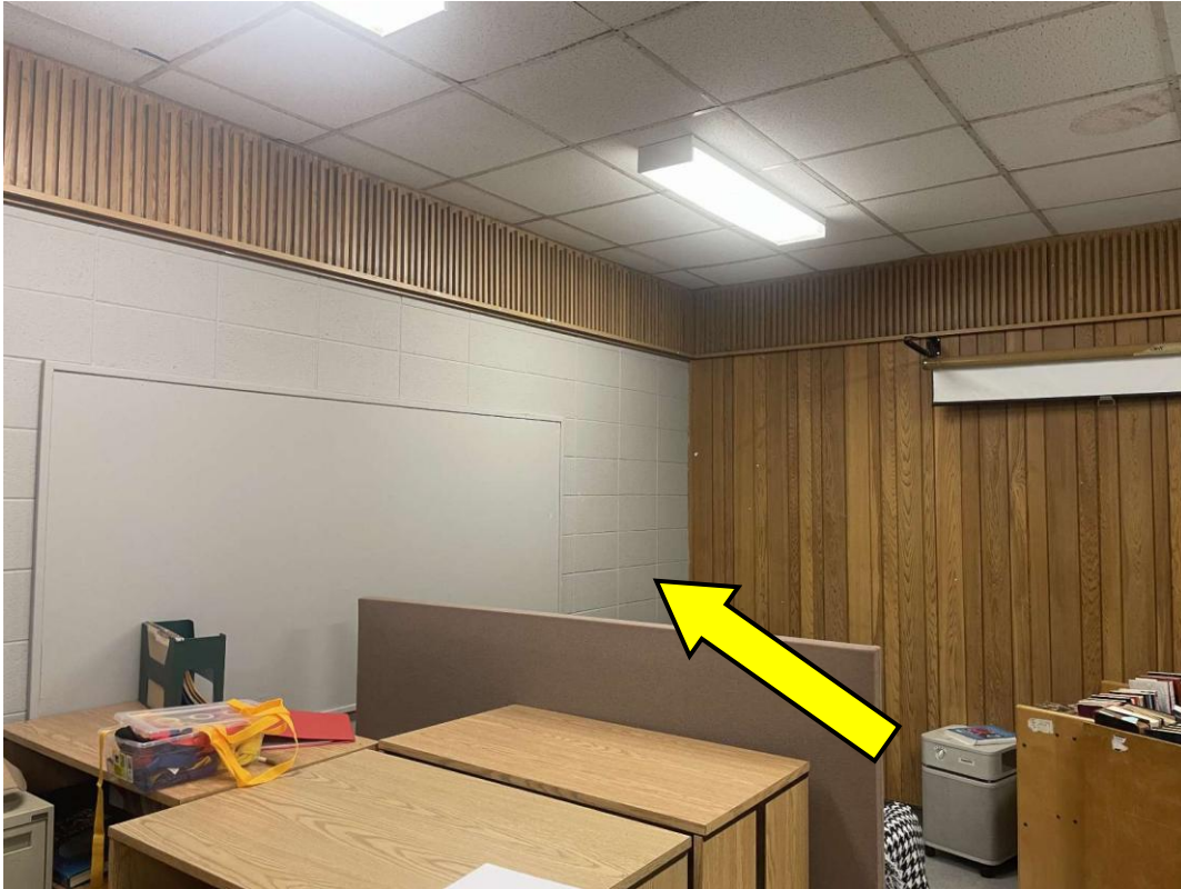
S0063A (None), Paint on block, Wall, Paint, Teacher Workstation (Location #: 2379)
