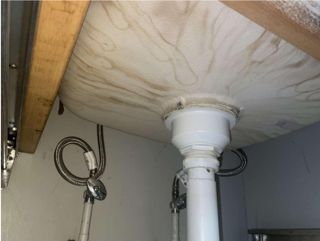
S0061A (None), Other, Sink, Mastic, White, Teacher Workstation (Location #: 2379)
