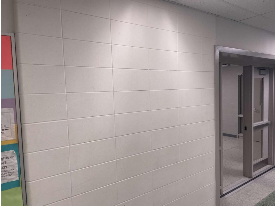
S0071A (None), paint on block, Wall, Paint, Corridor (Location #: 2576)
