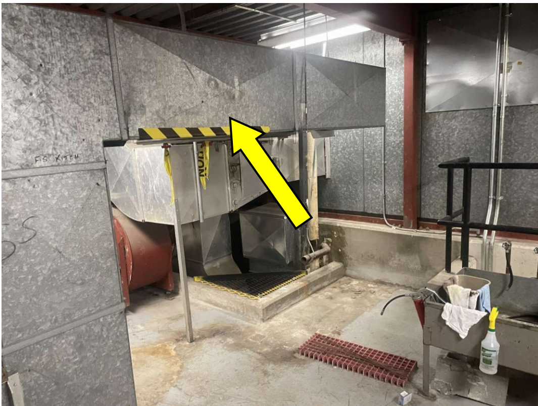
Duct, All, Not Insulated, Pipe Chase And Mechanical Penthouse (Location #: 2583)
