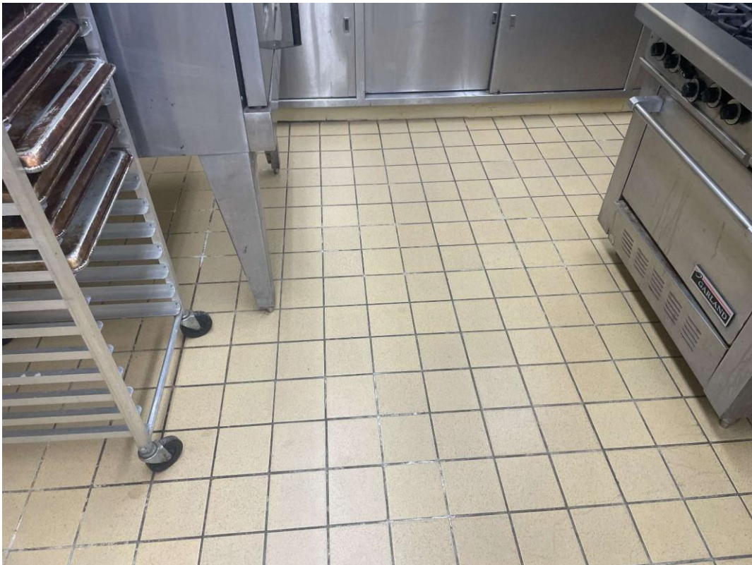
V9500 (Presumed Asbestos), Floor, Thin-set, Storage (Location #: 2377)
