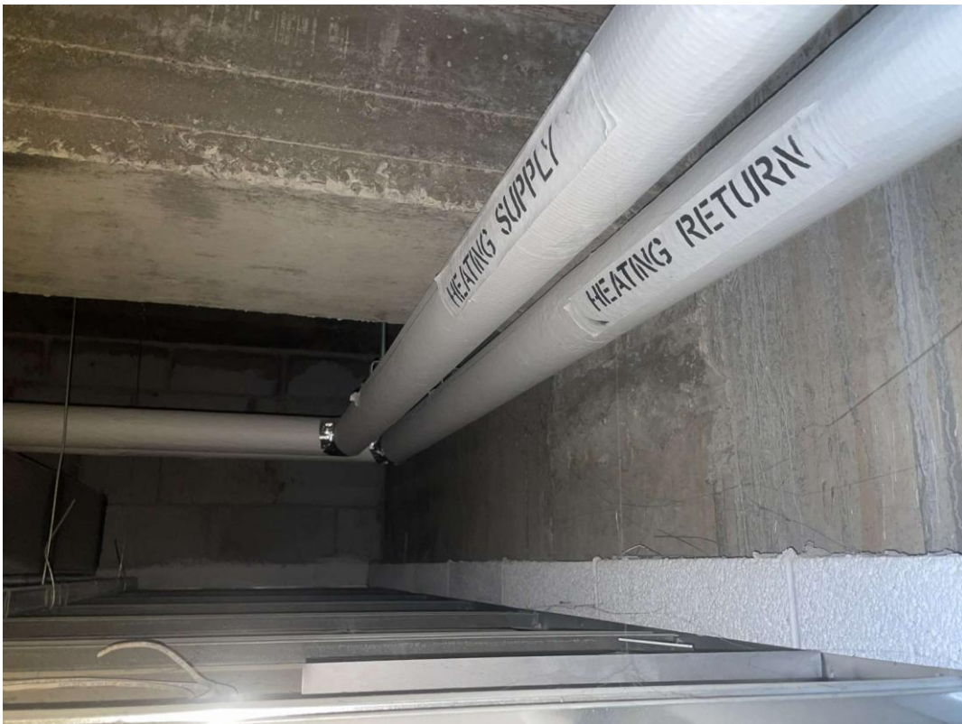
Piping, Fibreglass, Girls Changeroom (Location #: 2367)
