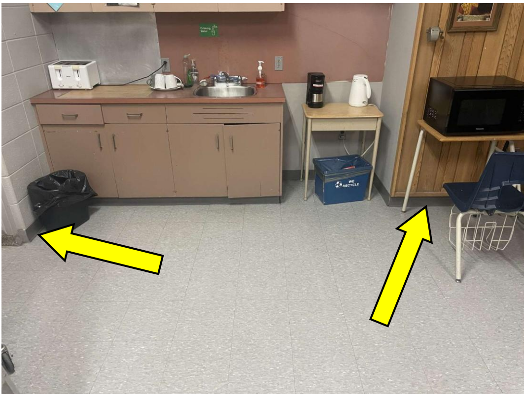
S0064A (None), Baseboard mastic, Wall, Mastic, Brown, Teacher Workstation (Location #: 2379)
