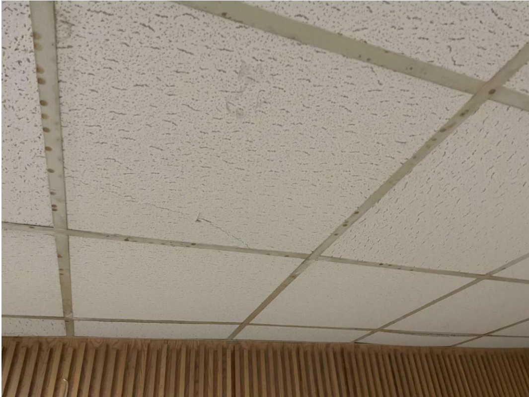
V0000 (None), 24x24 pinhole and large fissures, date stamped 09/07/03, Ceiling, All, Ceiling Tiles (lay-in), Teacher Workstation (Location #: 2379)
