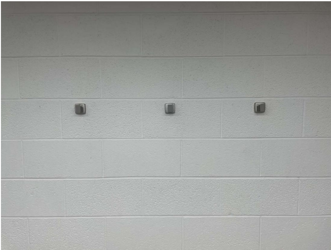
S0071B (None), Paint on block, Wall, Paint, Girls Changeroom (Location #: 2367)
