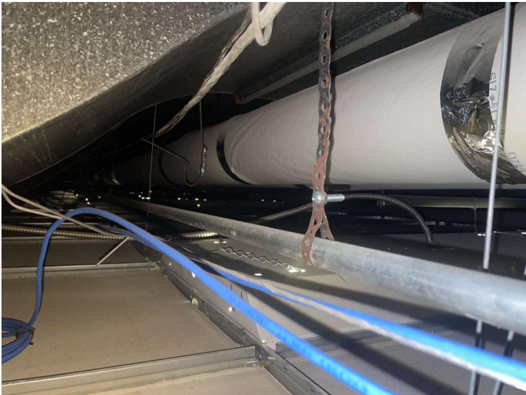
Piping, All, Fibreglass, Corridor (Location #: 2414)
