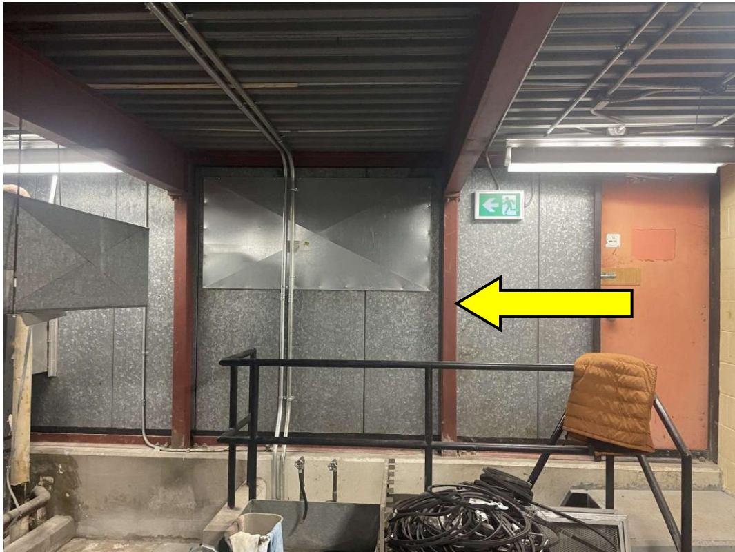
L0029(Lead, High), Structure, Pipe Chase And Mechanical Penthouse (Location #: 2583)
