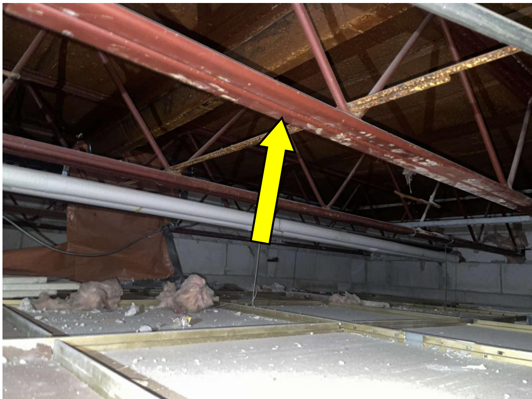
L0032(Lead, High), Red on structure, Structure, Teacher Workstation (Location #: 2379)
