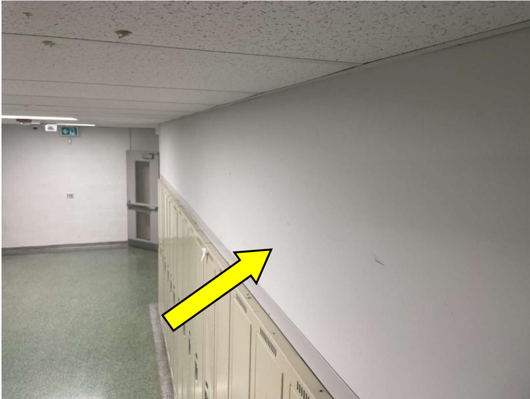
L0033(Lead, None), White on walls, Wall, Corridor (Location #: 2415)
