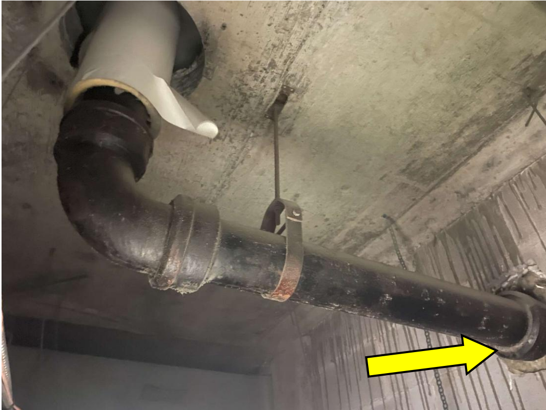
Pb Products, V9500(Presumed), BELL AND SPIGOT FITTINGS, Rain water leader, Corridor (Location #: 2576)
