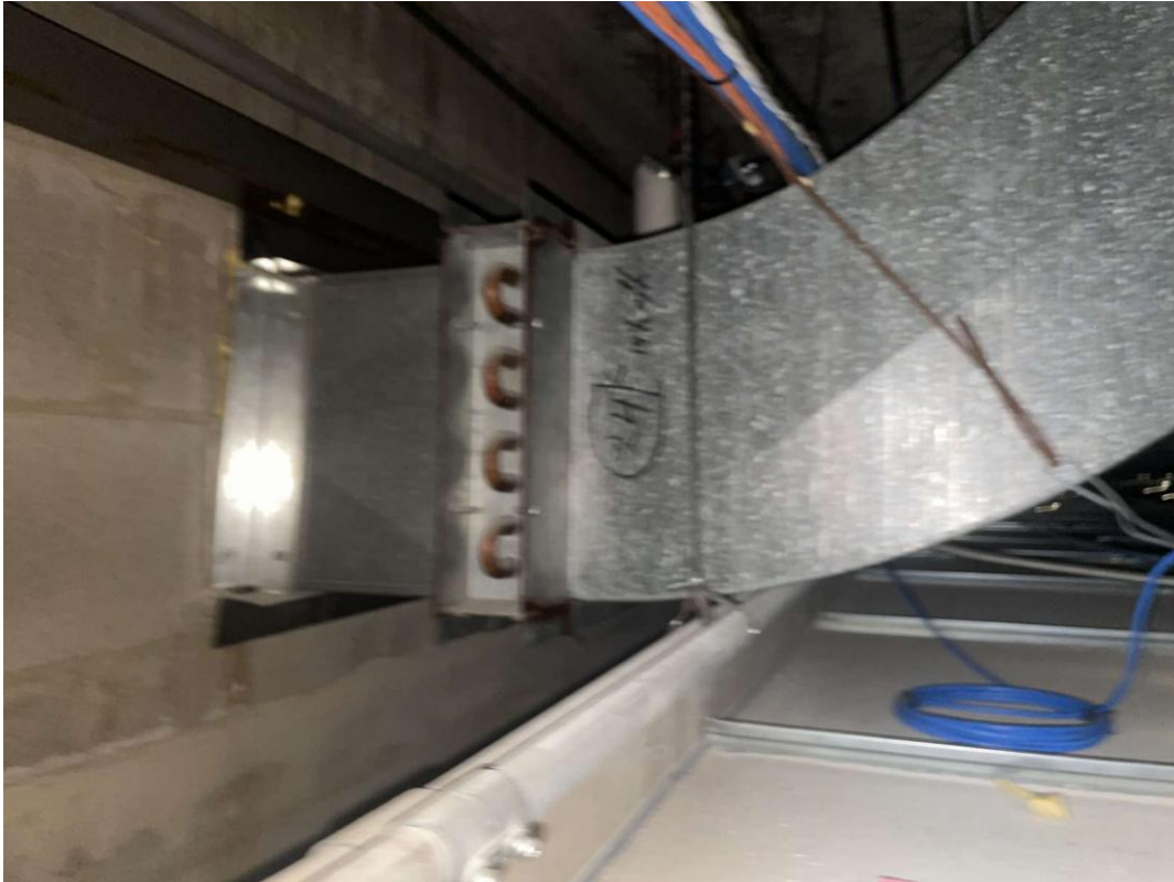
Duct, All, Not Insulated, Corridor (Location #: 2414)
