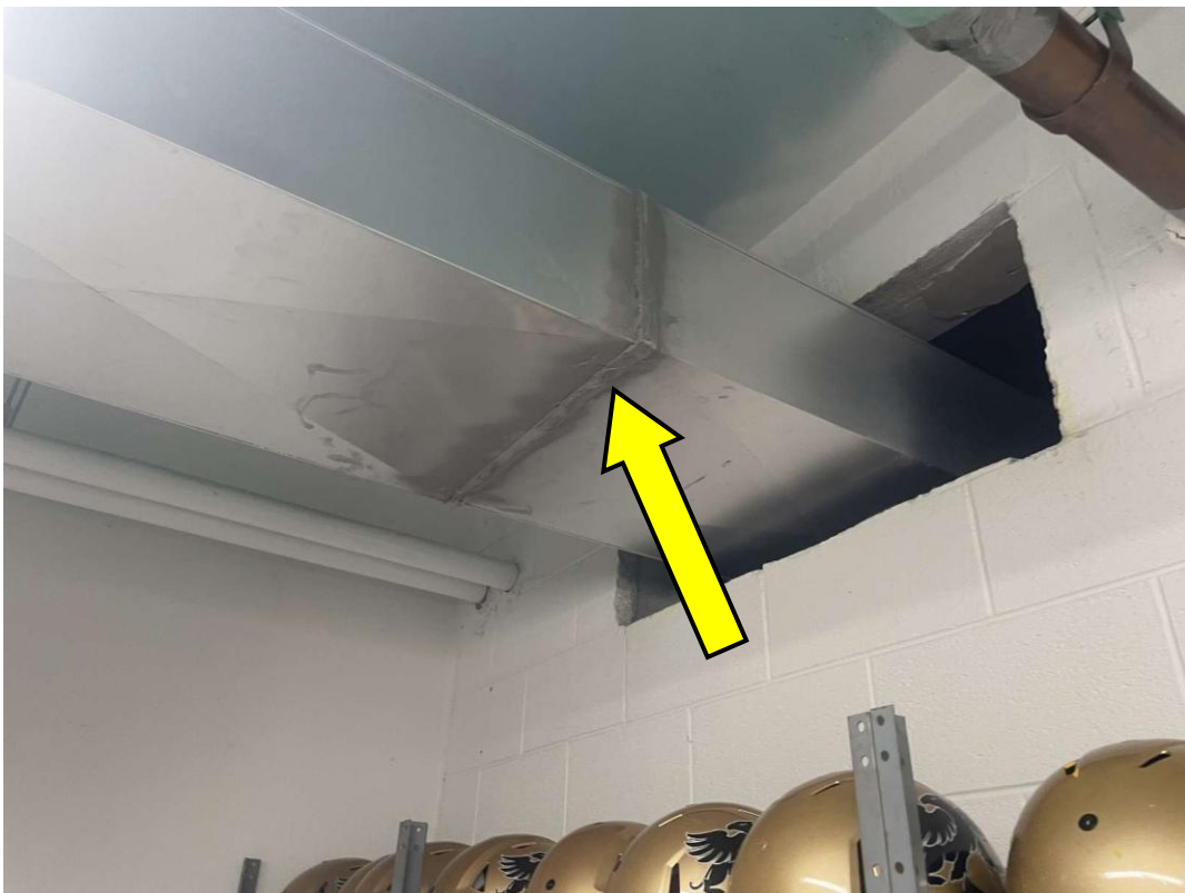
S0072A (None), Duct, Mastic, Grey, Storage (Location #: 2364)
