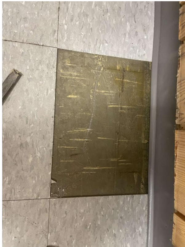
S0062A (Confirmed Asbestos), 12x12 grey with grey and white fleck, on top of 9x9 Grey with white streaks, Floor, Vinyl Floor Tile and Mastic, Teacher Workstation (Location #: 2379)
