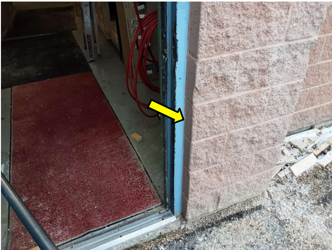
S0018A (None), Light brown, Other, Door, Caulking, Exterior 1991 (Location #: 19)
