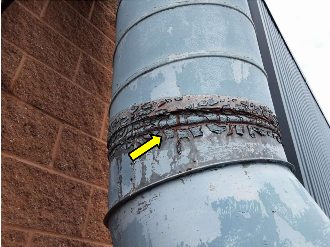
S0015A (None), Red on sawdust collector, Duct, Mastic, Exterior 1991 (Location #: 19)
