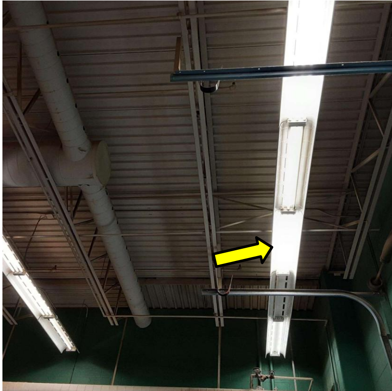
Mercury, V9500(Presumed), Mercury Vapour Lamp, Construction Shop (Location #: 22)
