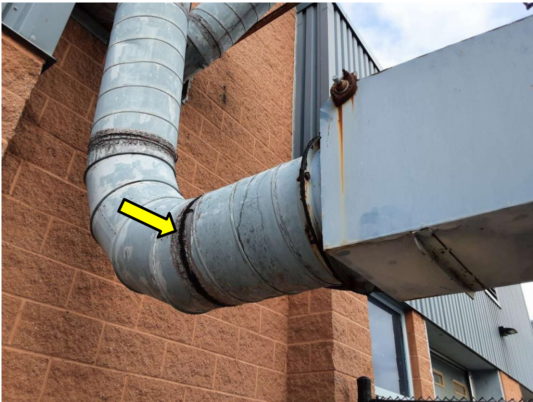
S0014A (None), Black on sawdust collector, Duct, Mastic, Exterior 1991 (Location #: 19)
