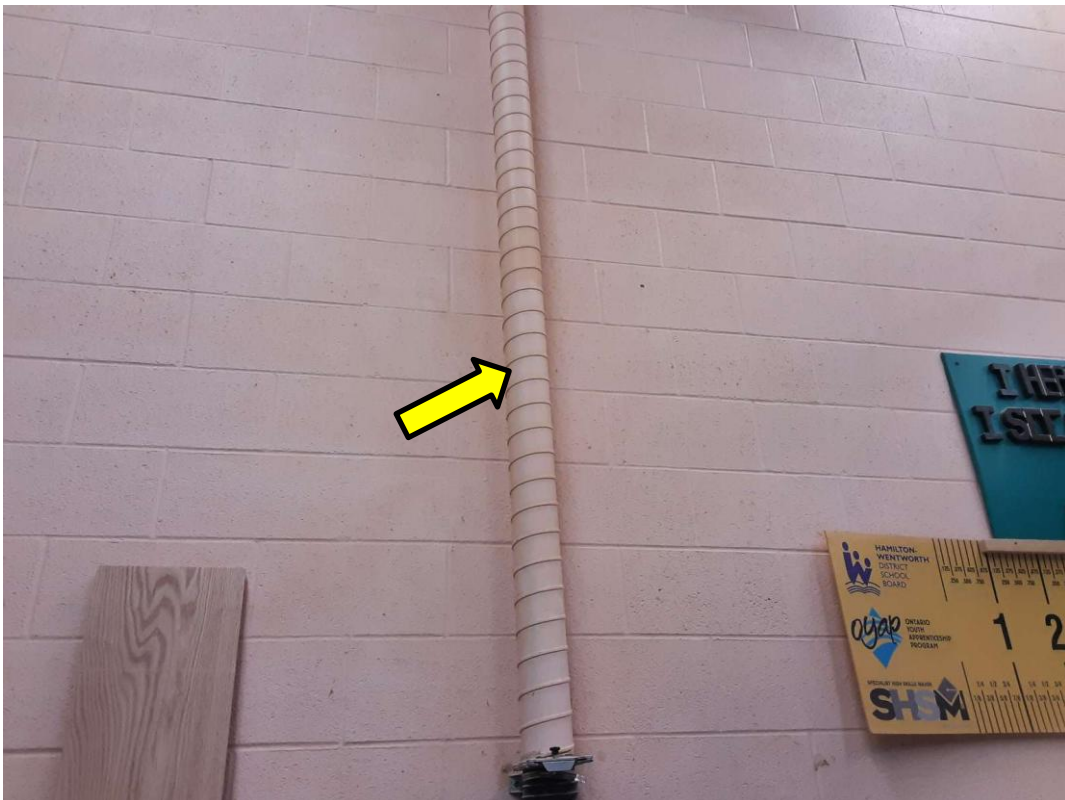
L0015(Lead, None), Salmon, Duct, Construction Shop (Location #: 22)
