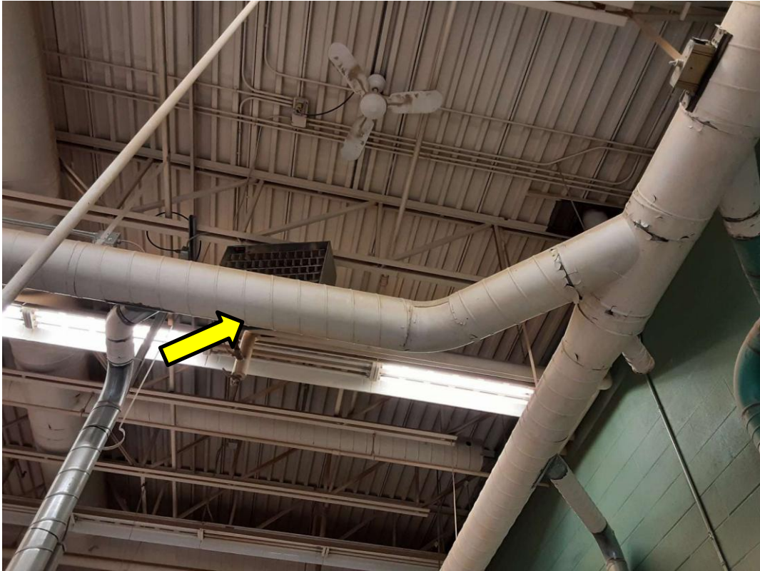
L0010(Lead, None), Cream on dust collector, Duct, Construction Shop (Location #: 22)
