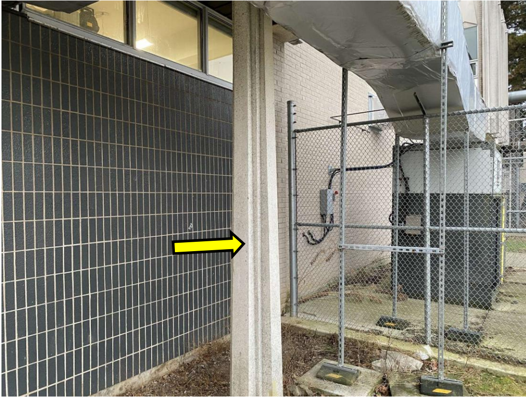
S0040 (Confirmed Asbestos), Wall, Column, Texture Finish - Non Friable, Exterior at 7562 and 7690 (Location #: 75620)
