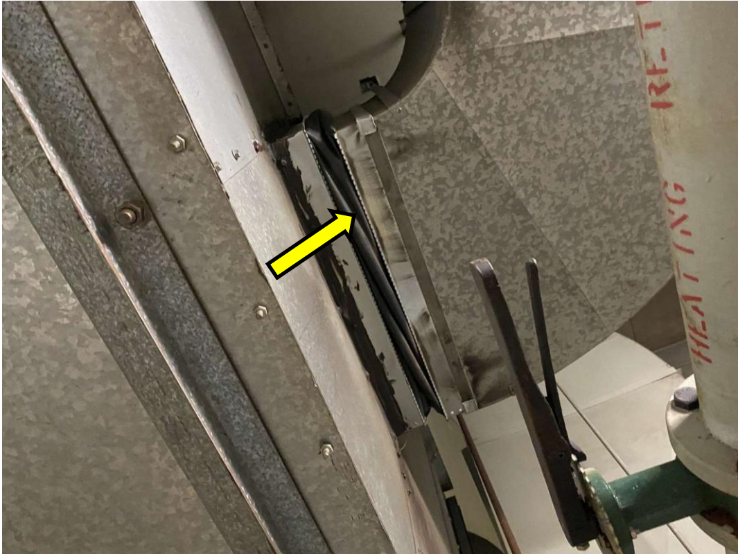
V9500 (Presumed Asbestos), Textile vibration damper, Duct, Exhaust, Textile, Mechanical Room (Location #: 7692)
