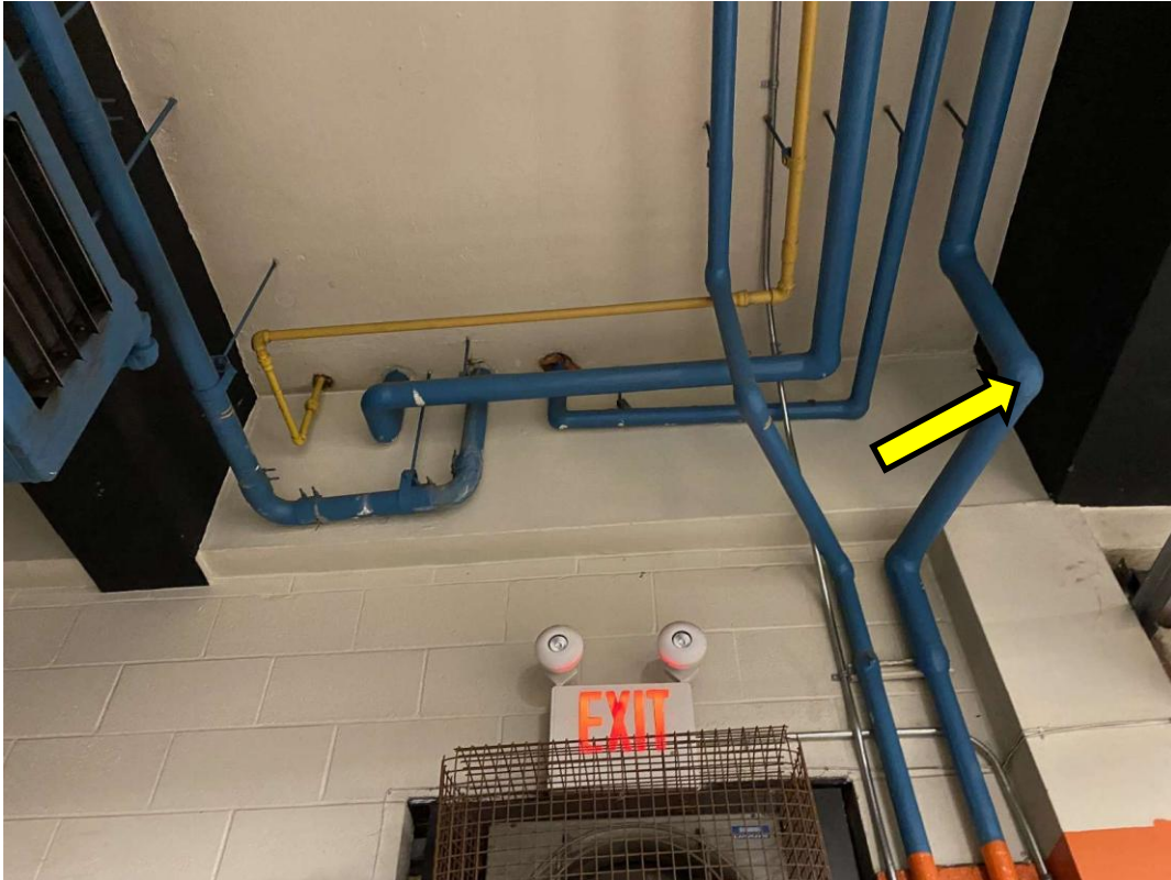
V0021 (Confirmed Asbestos), Piping, Parging Cement, Classroom (Location #: 7558)
