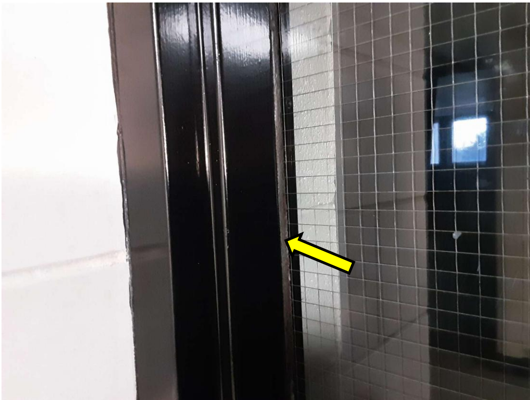
S0051A (Confirmed Asbestos), Black butyl sealants, Wall, Window Liner, Caulking, Corridor (Location #: 7752)
