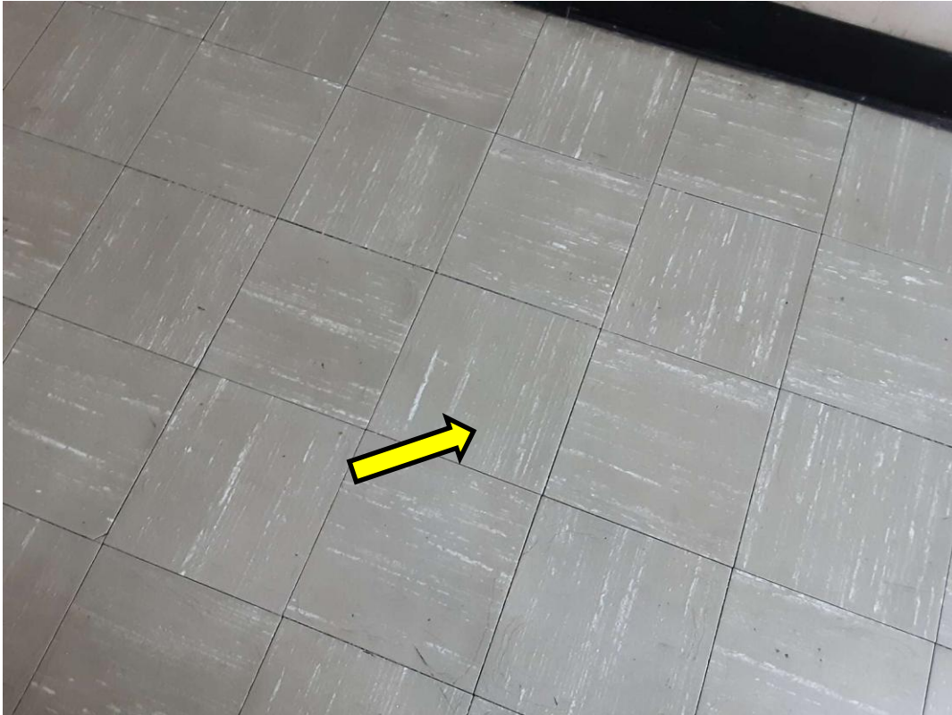
V0052 (Confirmed Asbestos), 12" x 12" Olive with white streaks; S0052B; phase c, Floor, Floor Levelling Compound, Corridor (Location #: 7696)
