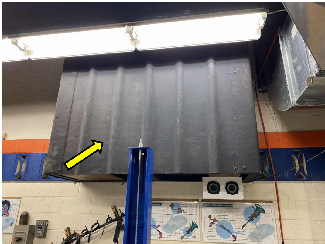
V0064 (Confirmed Asbestos), Transite, Other, Cement Product, Classroom (Location #: 7558)
