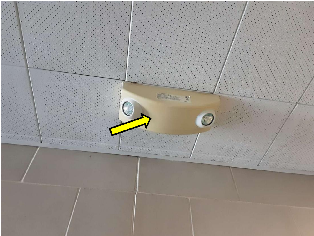
Pb Products, V9500(Presumed), Batteries in emergency lights, Corridor (Location #: 7696)
