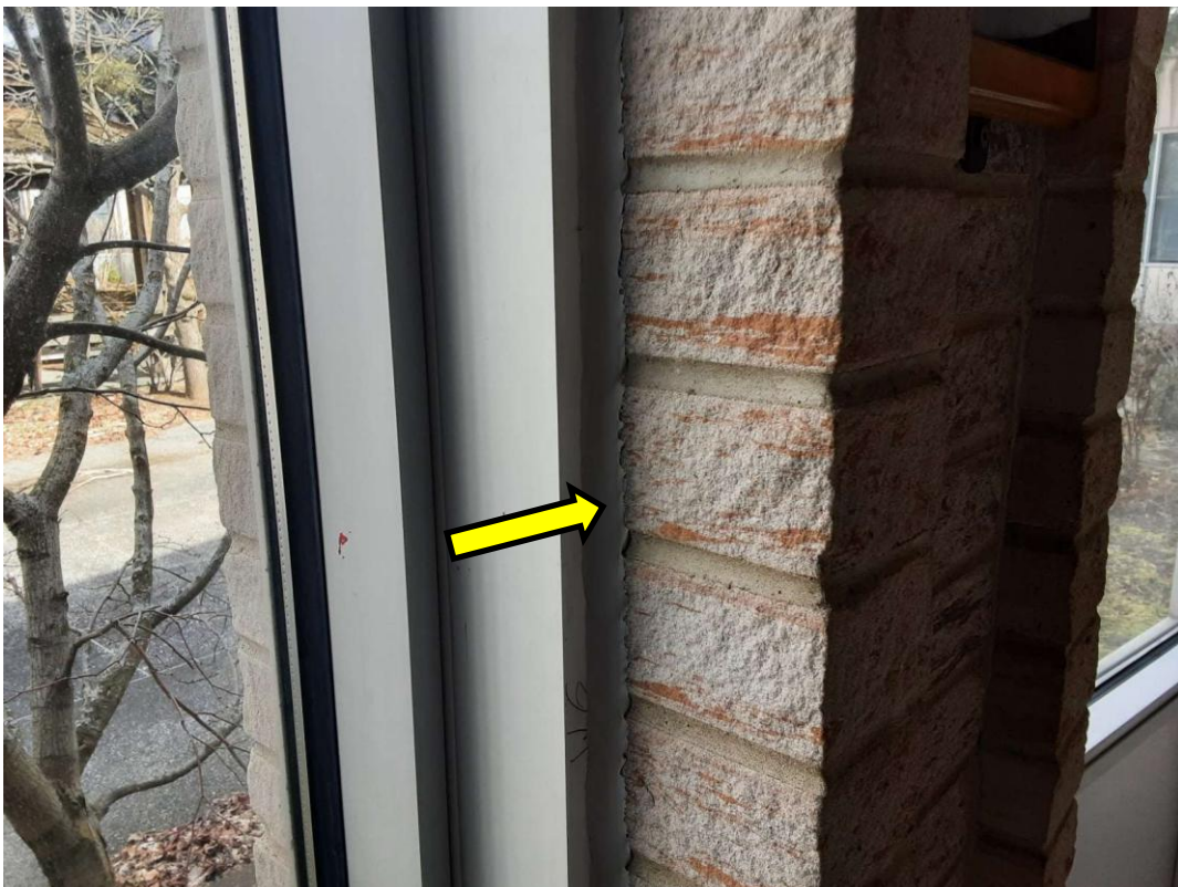
V0053 (None), Grey on window frame, Wall, Window, Caulking, Corridor (Location #: 7596)
