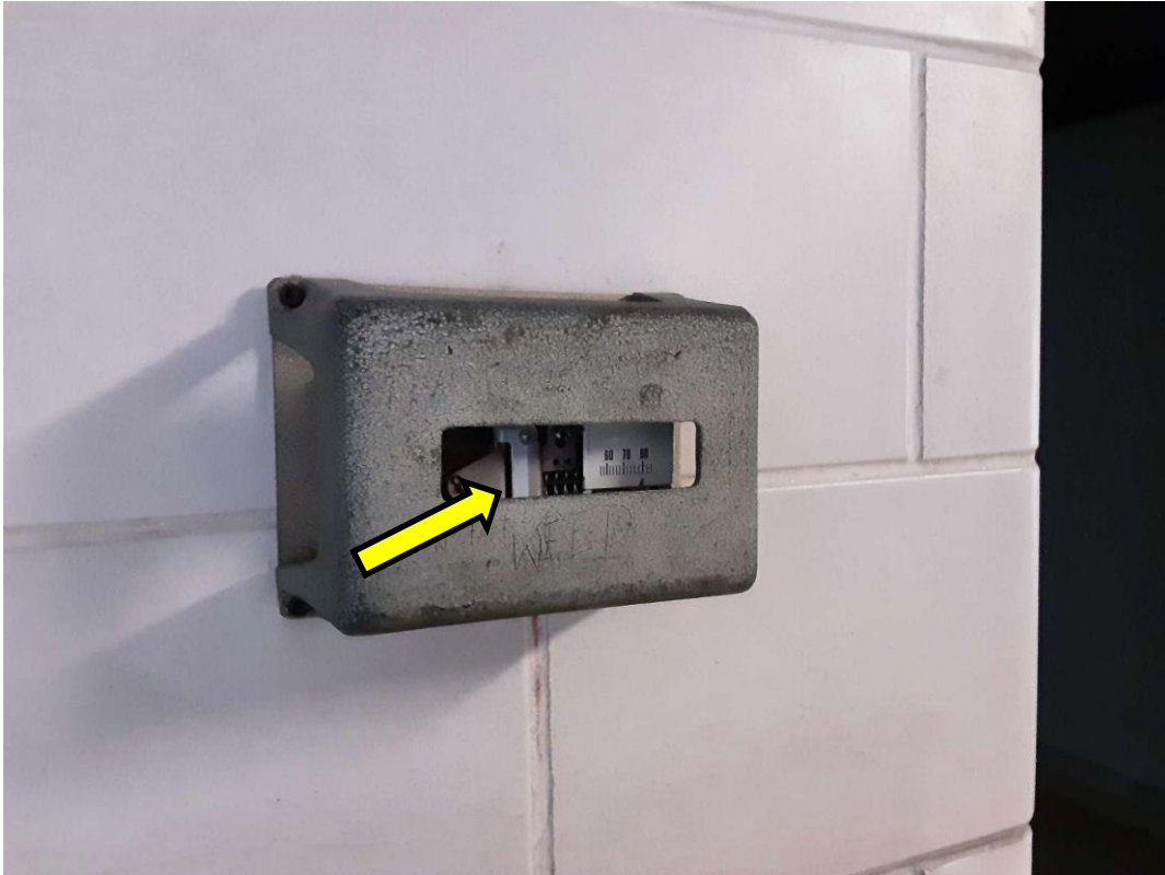
Mercury, V9000(Presumed), Thermostat, Corridor (Location #: 7708)
