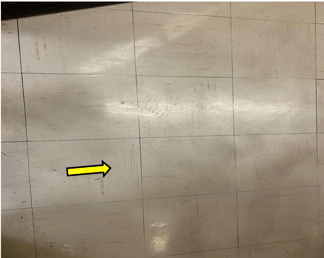
S0075A (None), 12x12 beige with brown streaks, Floor, Vinyl Floor Tile and Mastic, Office (Location #: 7698)
