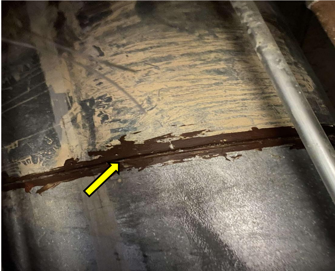
S0062B (Confirmed Asbestos), Dark Brown, Duct, Mastic, Corridor (Location #: 7554)
