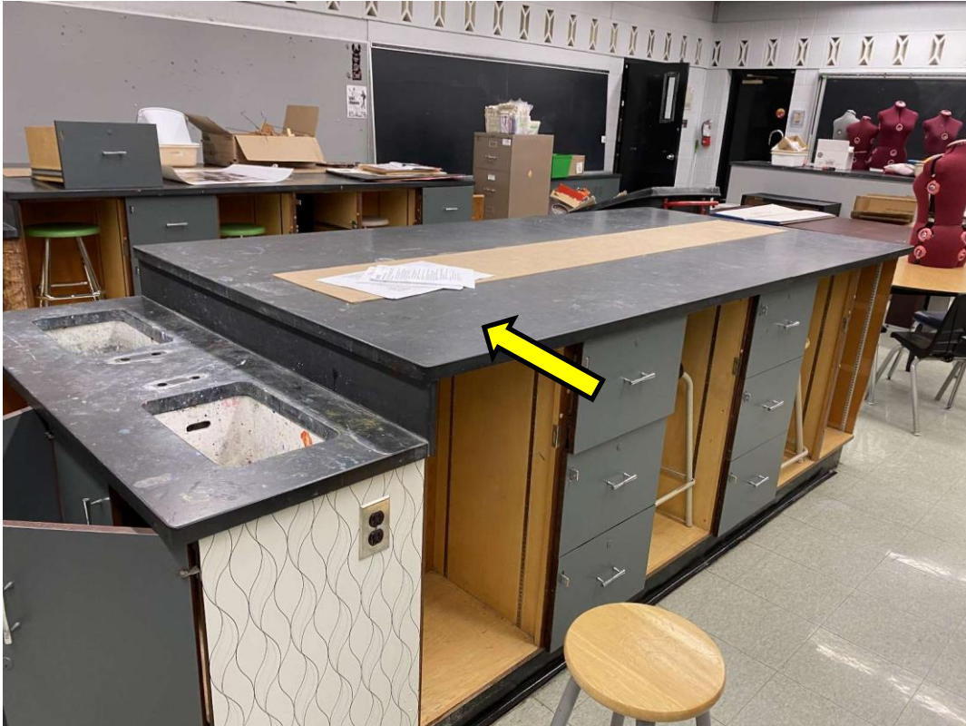
S0069A (Confirmed Asbestos), Other, Bakelite, Classroom (Location #: 7689)
