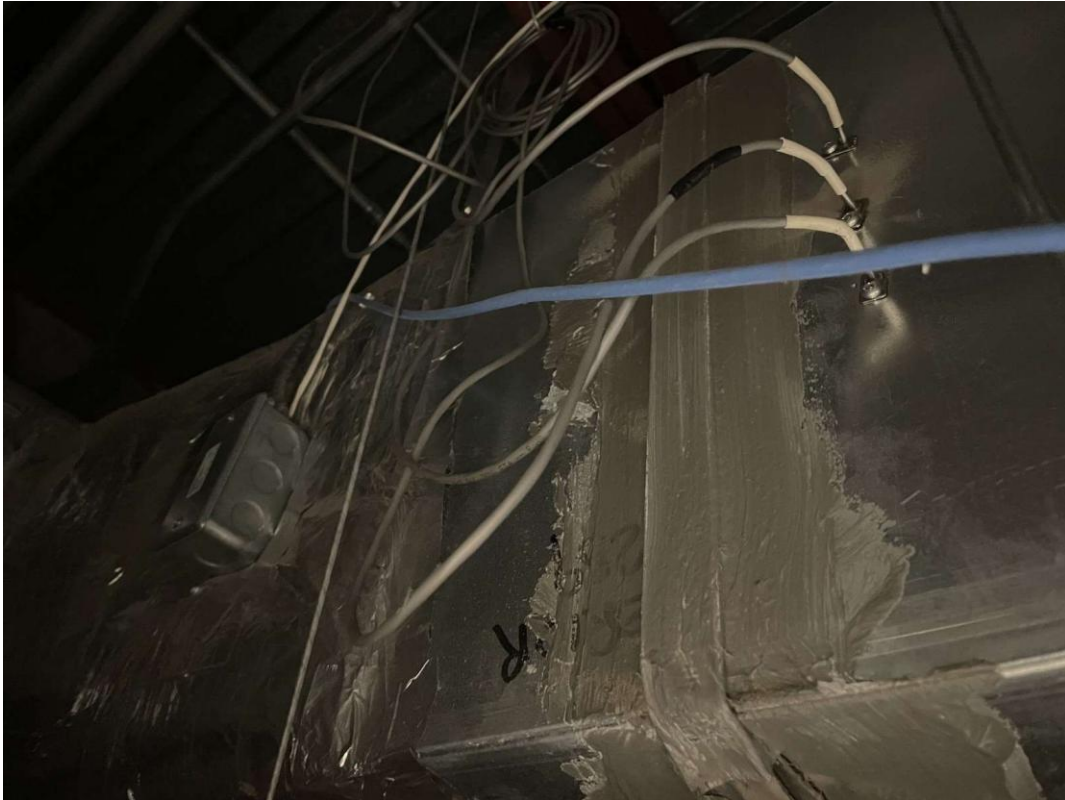
S0006A (None), Duct, Mastic, Grey, Corridor (Location #: 9074)
