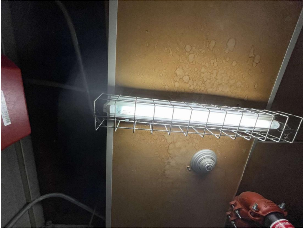
Mercury, V9000(Yes), Light Fixture, Sprinkler Room (Location #: 9040)
