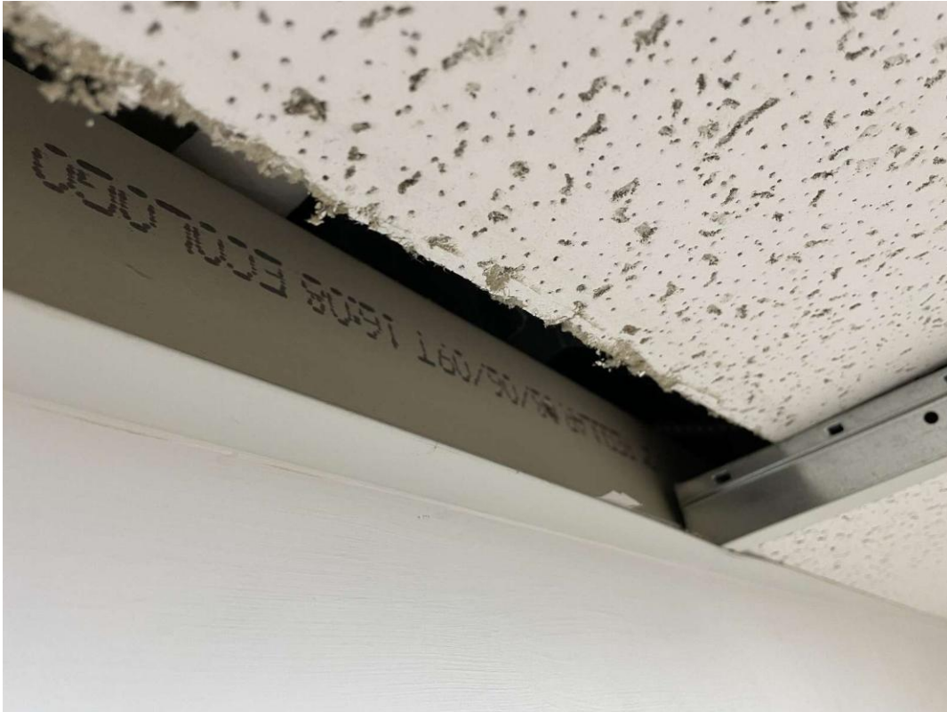
V0000 (None), bulkhead and ceiling (2009 date stamp), Ceiling, Drywall and joint compound, Lobby (Location #: 9073)
