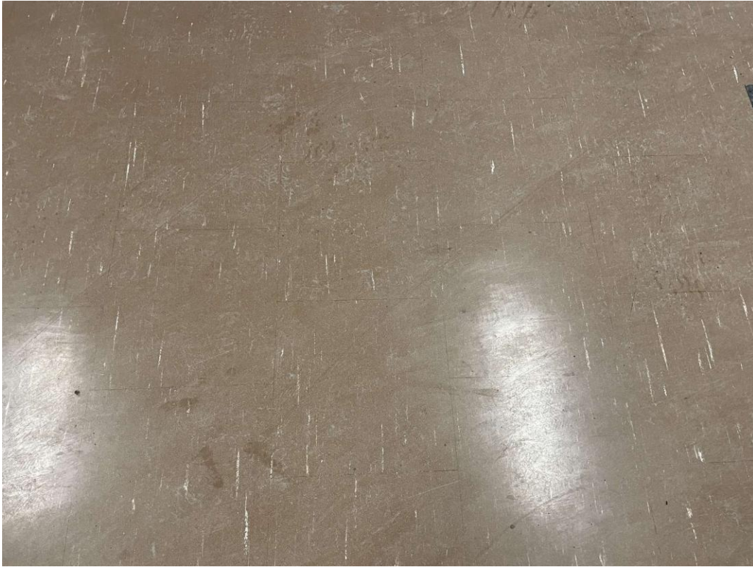
V9500 (Presumed Asbestos), 12x12 brown with white streaks, Floor, Vinyl Floor Tile and Mastic, Corridor (Location #: 9076)
