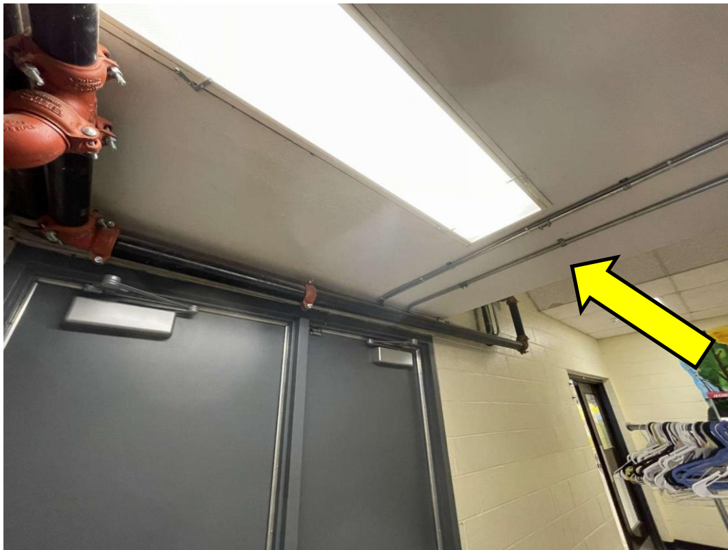
V9000 (Confirmed Asbestos), Textured, Ceiling, Plaster, Stairs (Location #: 9039)
