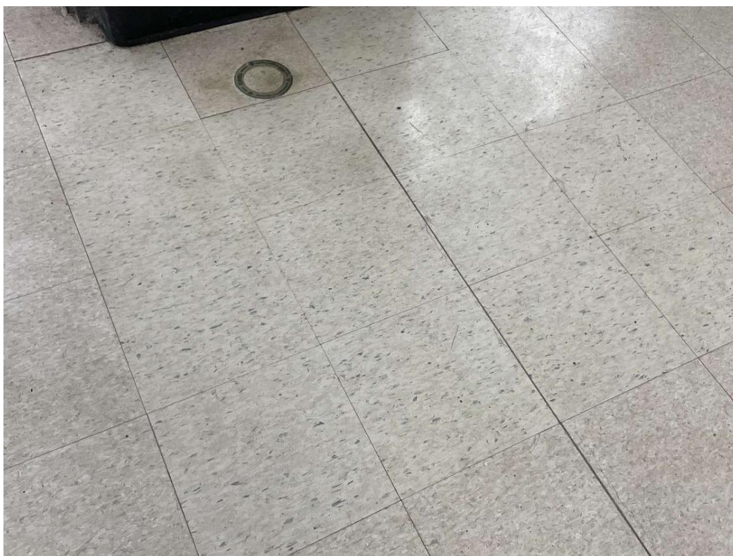
V9500 (Presumed Asbestos), 12x12 white with blue streaks, Floor, Vinyl Floor Tile and Mastic, Corridor (Location #: 9077)
