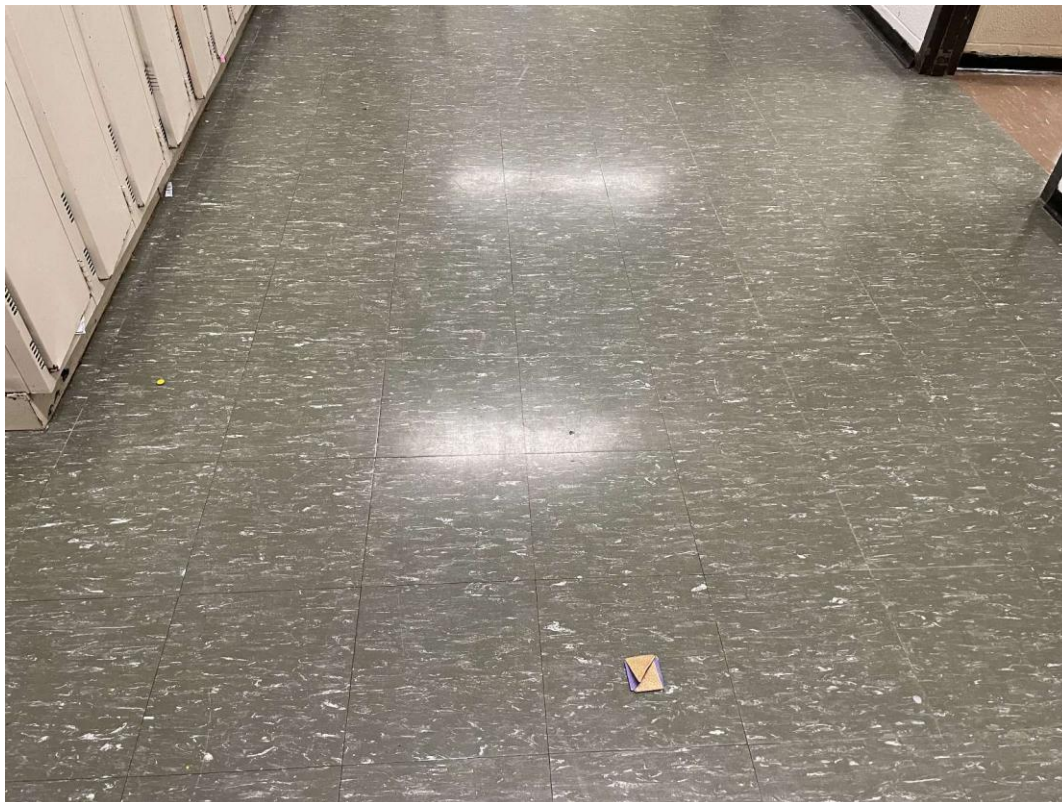
V9500 (Presumed Asbestos), 12x12 green with white streaks, Floor, Vinyl Floor Tile and Mastic, Corridor (Location #: 9072)
