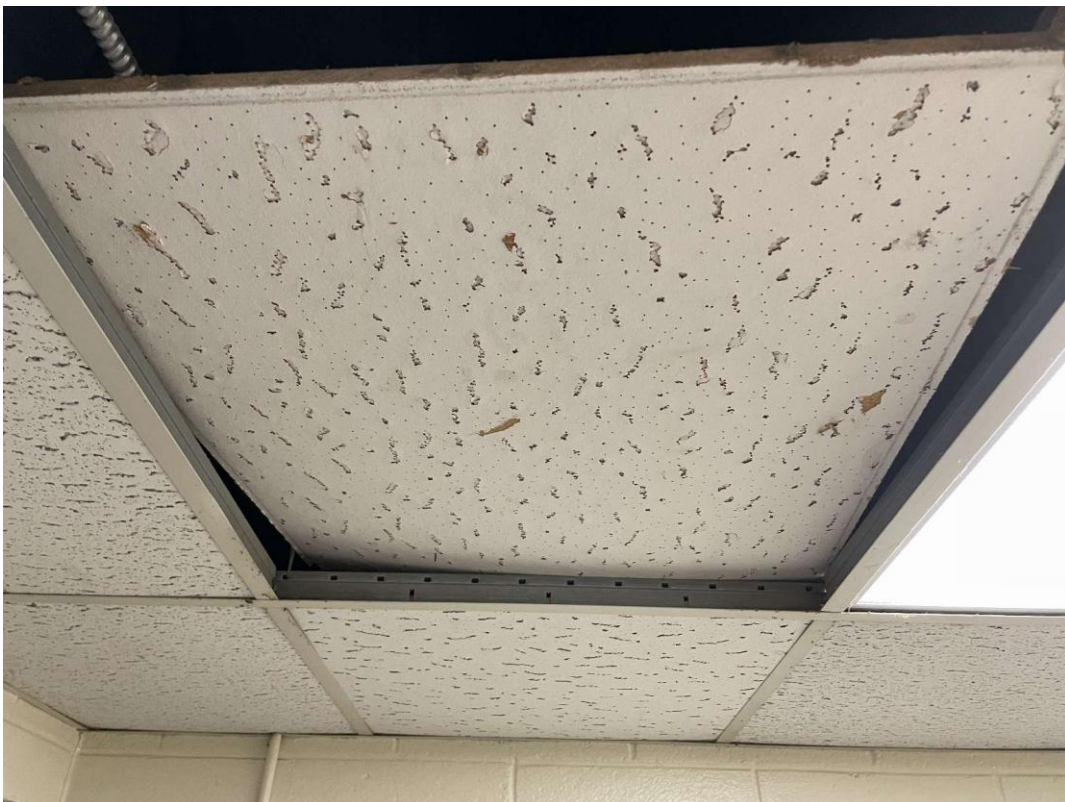
V0000 (None), 24x48 pinhole with length-wise fissure (particle board), Ceiling, ACOUSTIC TILE, Ceiling Tiles (lay-in), Stairs (Location #: 9039)
