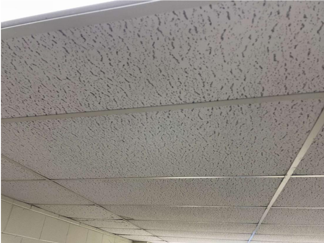
S0001A (None), 24x48 pinhole with width-wise fissure (Armstrong Fire Guard), Ceiling, ACOUSTIC TILE, Ceiling Tiles (lay-in), Stairs (Location #: 9039)
