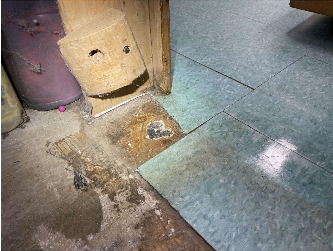
S0013A (Confirmed Asbestos), Floor, Mastic, Gym (Location #: 1032)
