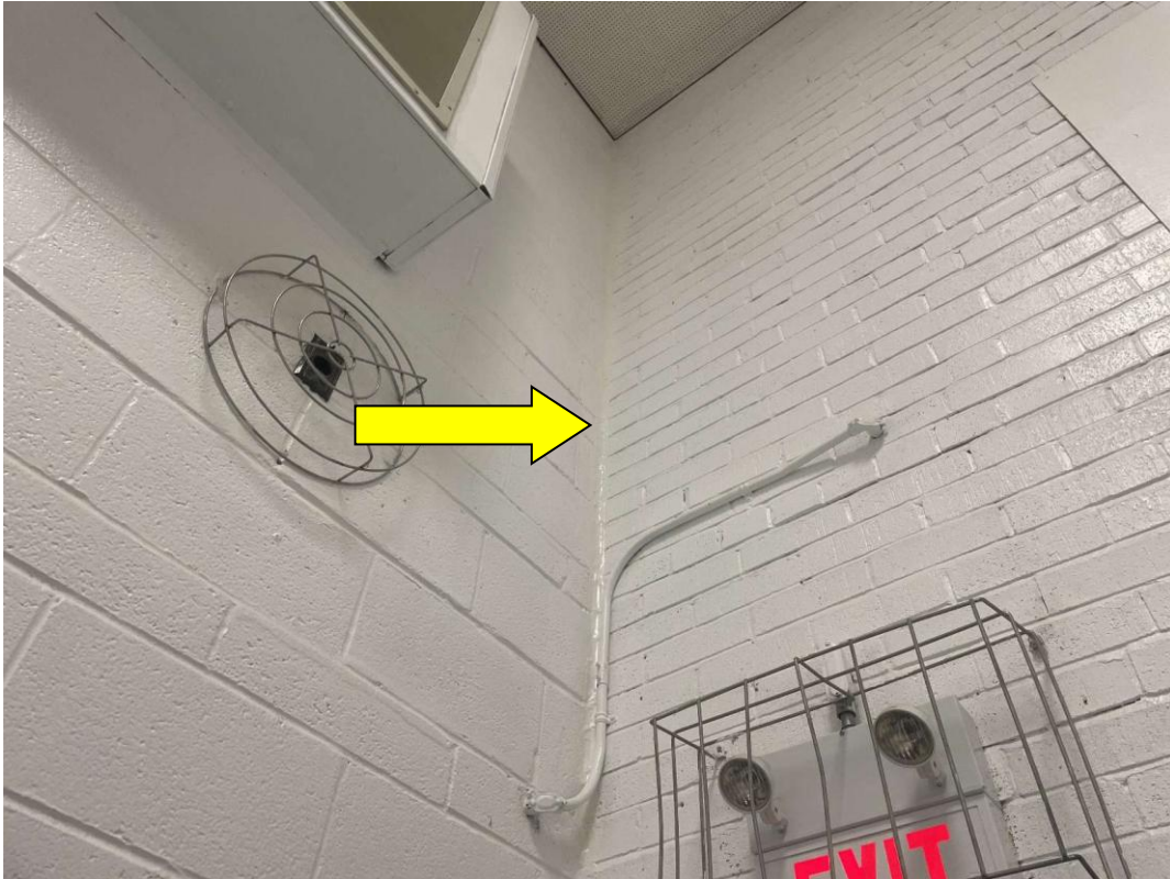
S0045A (None), Wall, Expansion Joint, Caulking, Gym (Location #: 1032)
