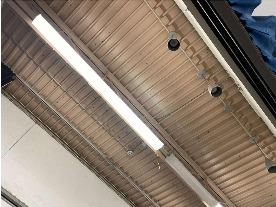
V0002(Lead, High), red, assumed present below beige paint (no access), Structure, Stage (Location #: 1033)
