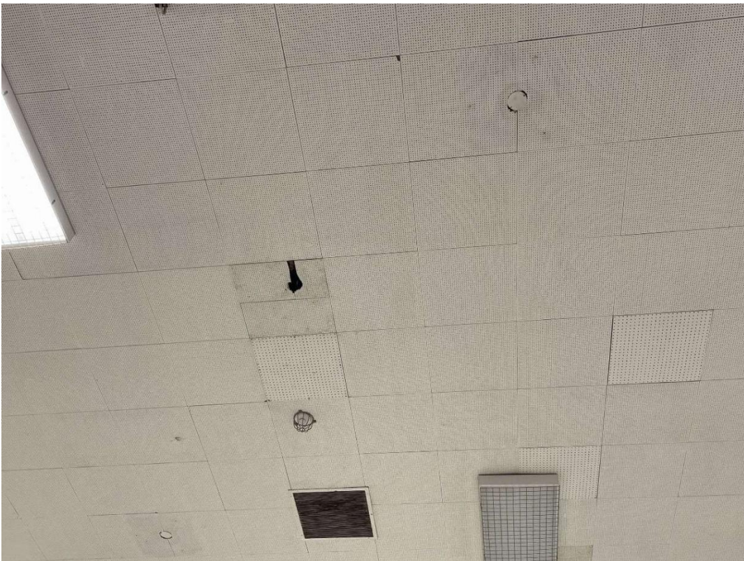
V9500 (Presumed Asbestos), 24x24 perforated, Ceiling, ACOUSTIC TILE, Cement Product, Gym (Location #: 1032)
