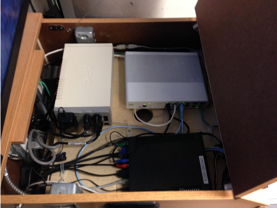
Fig 3.0.3: Top view of a clean TSJr installation – note presence of UPS and Network Switch.
