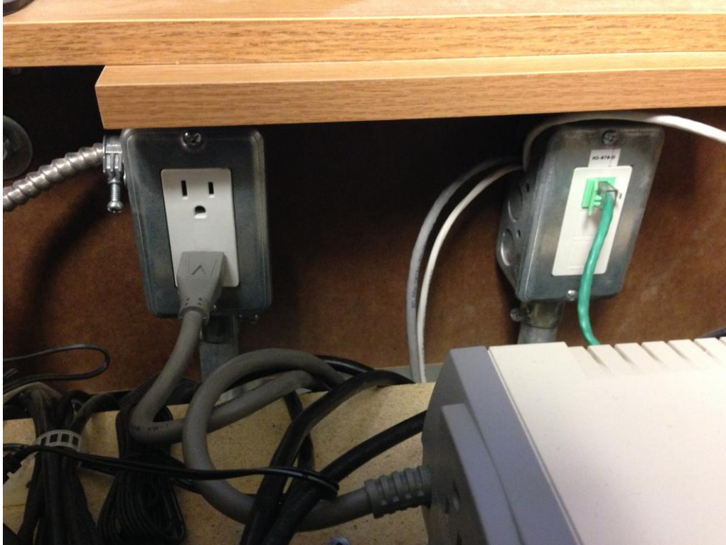
Fig 3.0.4: AC and data termination inside TSJr.
