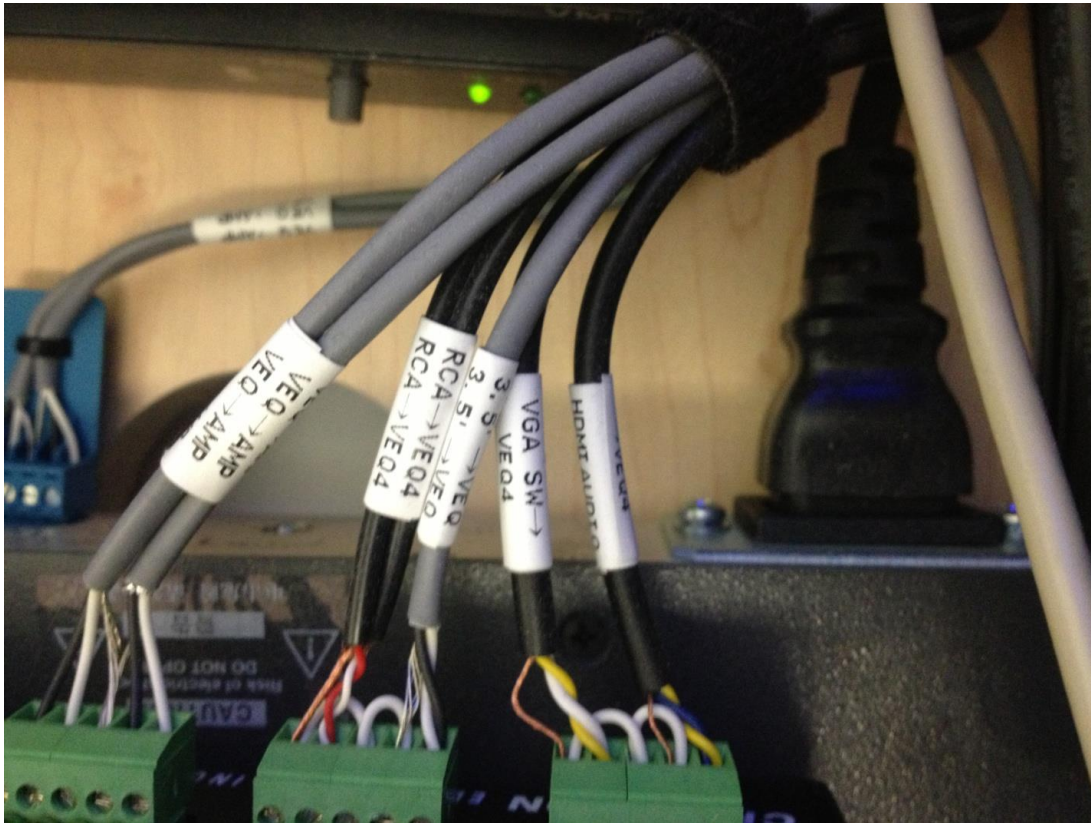
Fig 3.0.3: Inside a well installed TSJr. Note the clear cable labeling, cleanly integrated wire blocks, and Velcro tie for bundling.
