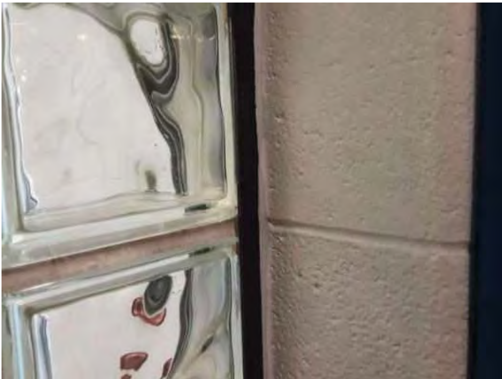
S0005B (None), Wall, Window, Caulking, Kan eff Auditorium (Location #: 6) Between wall and windowframe
