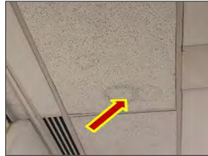
Photo 18: View of water-stained acoustic ceiling tiles (48"x24" small fissures and pinholes) present in Men's Pool Change Room (Loc. 17).
