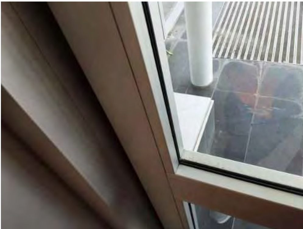
S0002A (None), Other, Door, Caulking, Entrance Corridor (Location #: 2) Between door frame and glass
