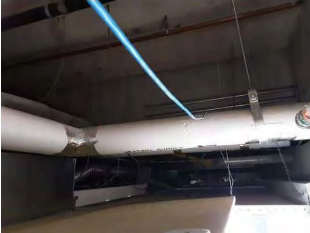
V0000 (None), Piping, Fibreglass, Entrance Corridor (Location #: 2) Heating supply and return
