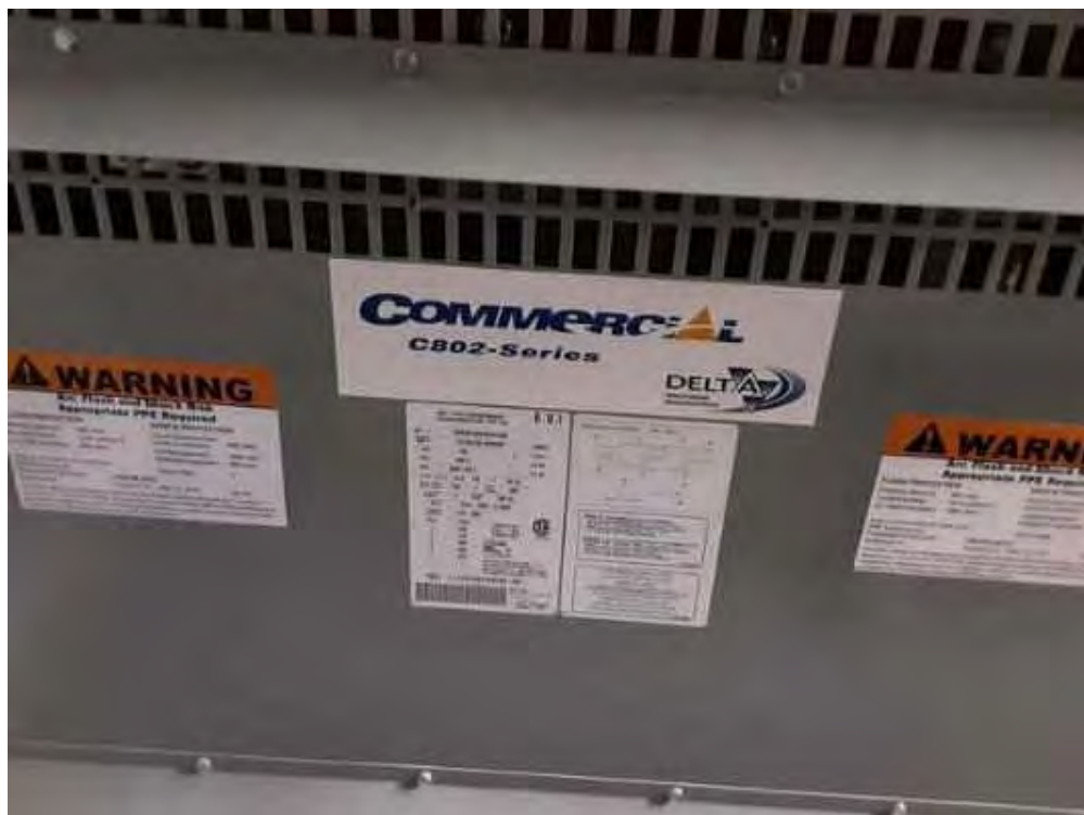
PCB, Electrical Room (Location #: 53)
