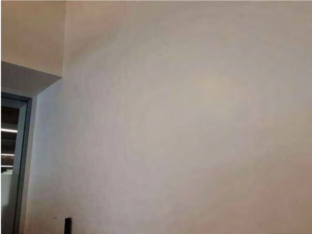
Drywall and joint compound, White, V0002, Fitness Studio (Location #: 51)
