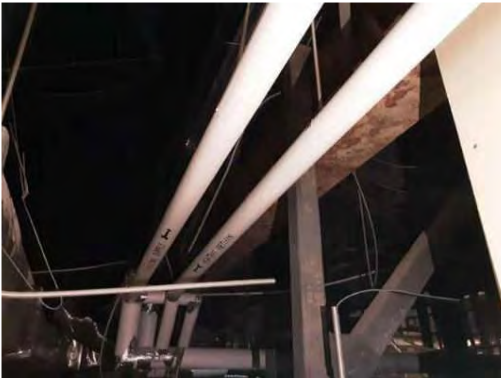
V0000 (None), Piping, Fibreglass, Program Room (Location #: 48)
