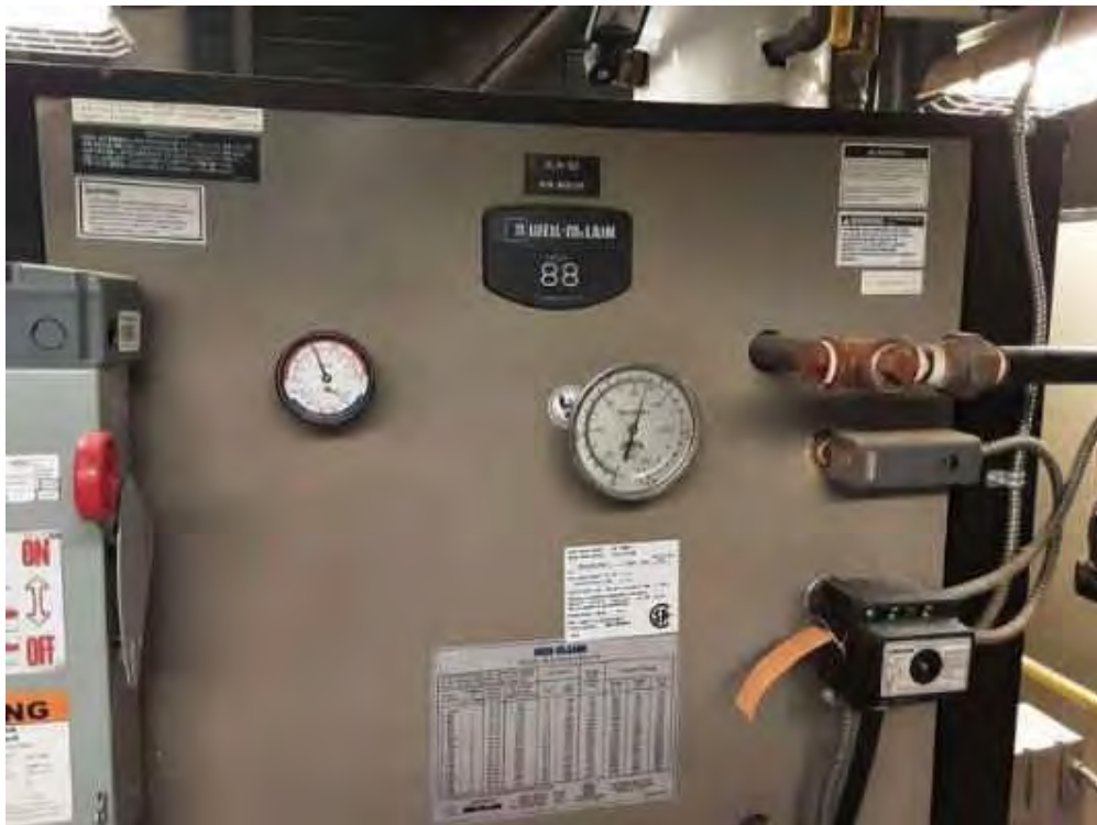
V0000 (None), Mechanical Equipment, Boiler, Not Insulated, Mechanical Room 2 (Location #: 55)
