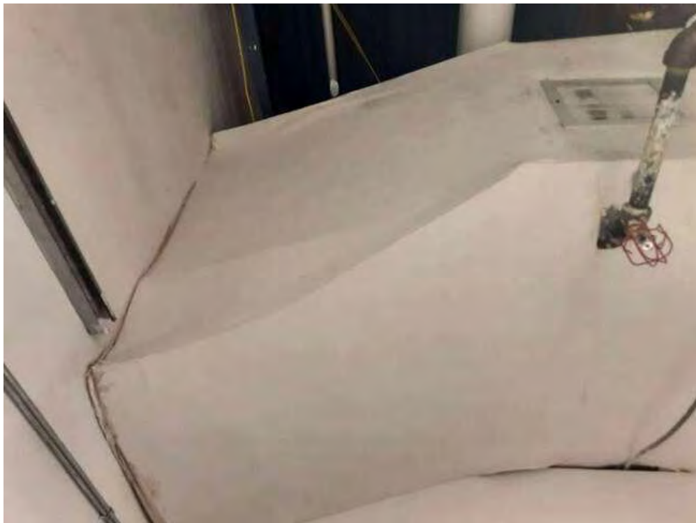
V0000 (None),Duct,Fibreglass,Electrical Room (Location#: 53)
