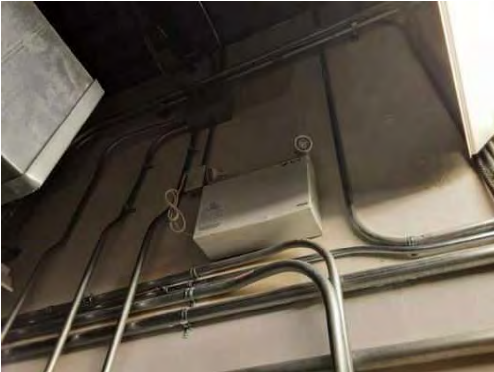
Pb Products, Electrical Room (Location #: 53)
