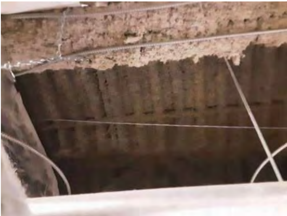
V0000 (None), Structure, All, Fireproofing (Fibrous), Men's Fitness Change Room (Location#: 15)
