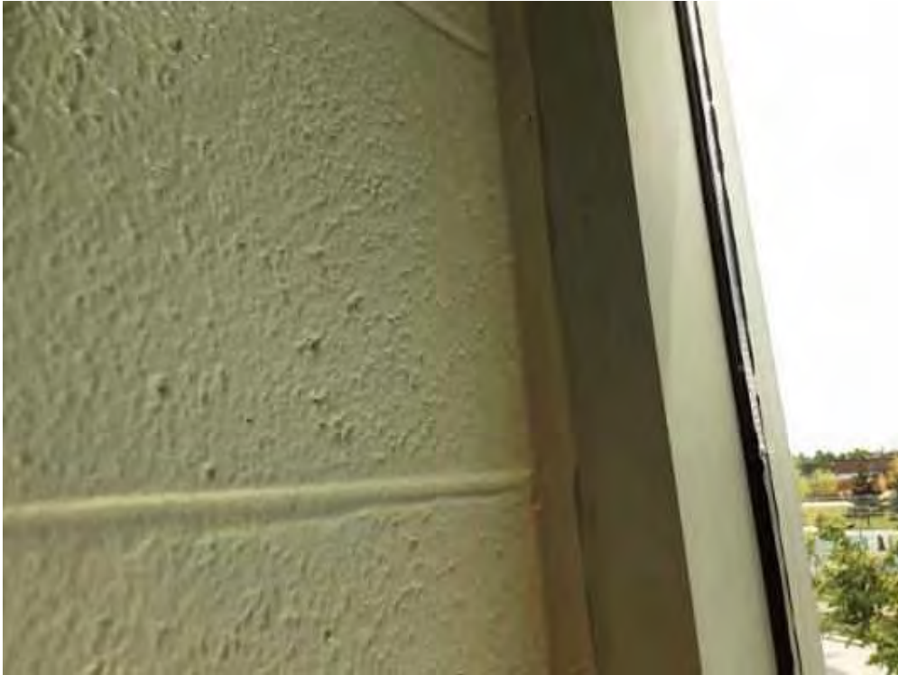
S0003C (None), Wall, Window, Caulking, Fitness Center (Location #: 50) Between wall and windowframe
