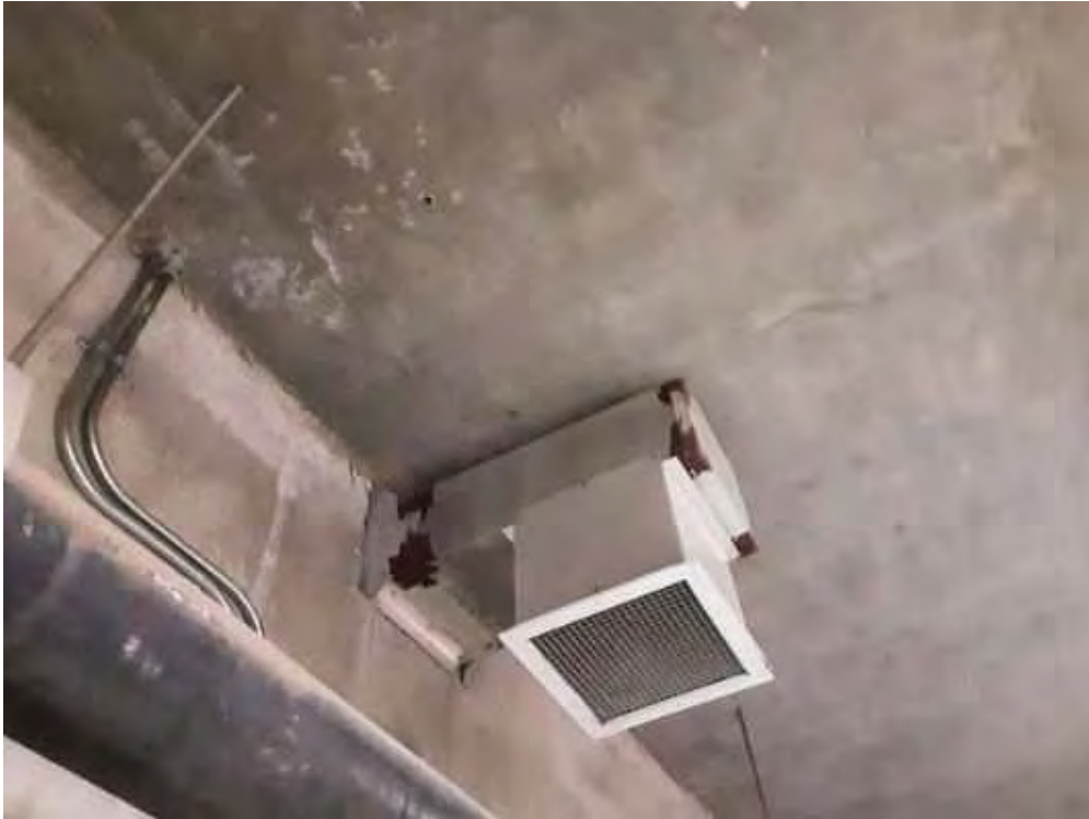
V0010 (None), Duct, Mastic, Storage (Location #: 43) 2 duct connections
