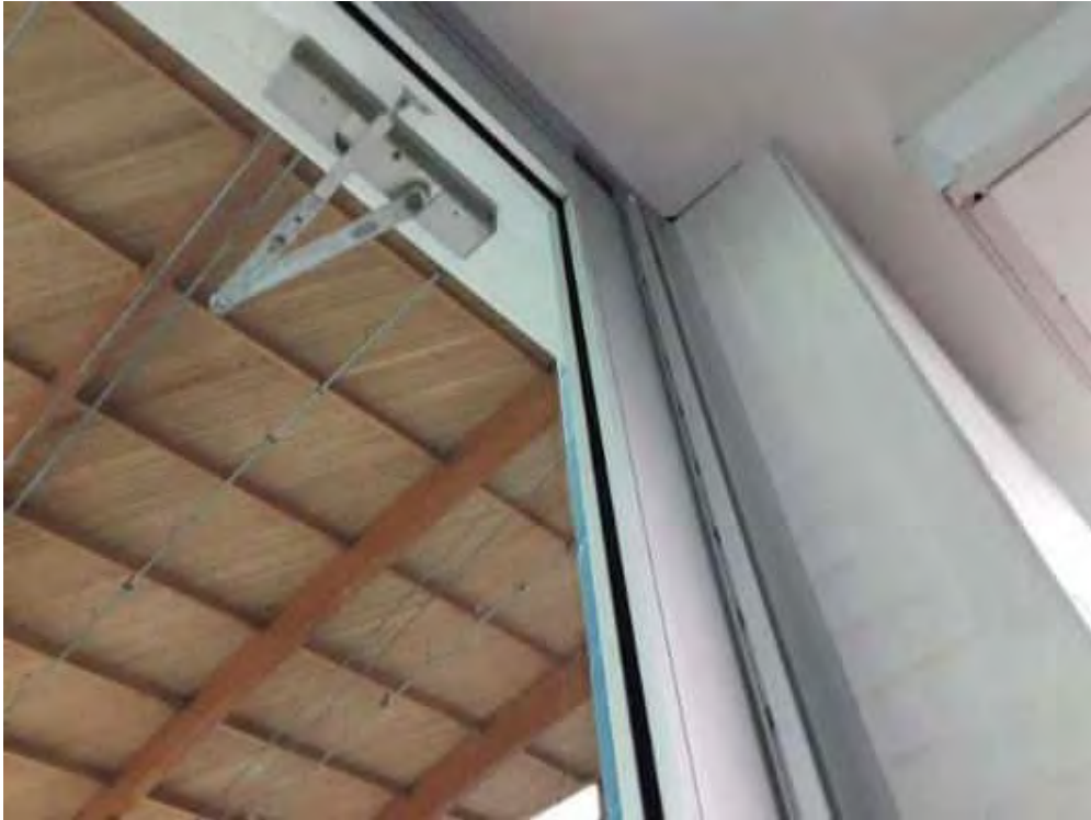
V0002 (None), Other, Door, Caulking, Lobby (Location #: 3) Between door frame and glass , pool door
