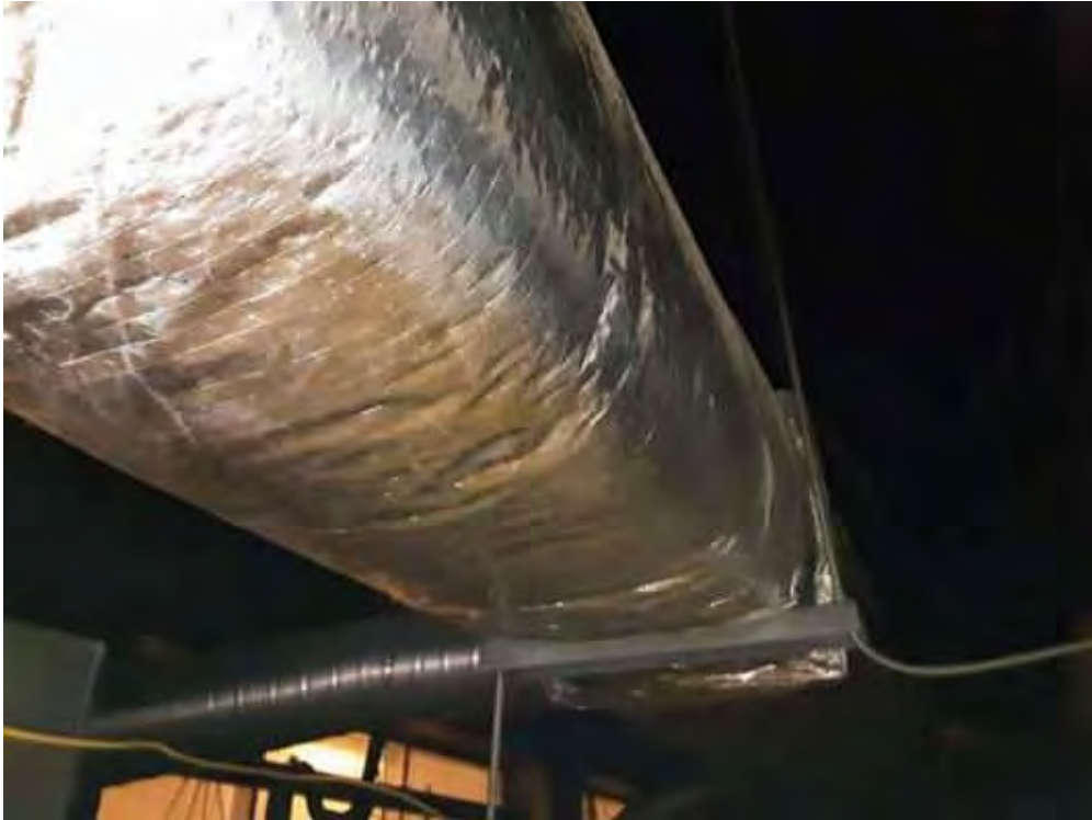
V0000 (None), Duct, Fibreglass, Program Room (Location #: 48)
