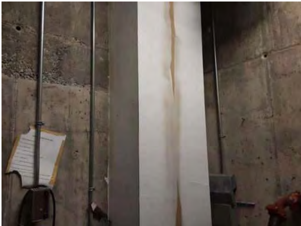
V0000 (None), Structure, Column, Elevator Room (Location #: 42) Drywall joint compound
