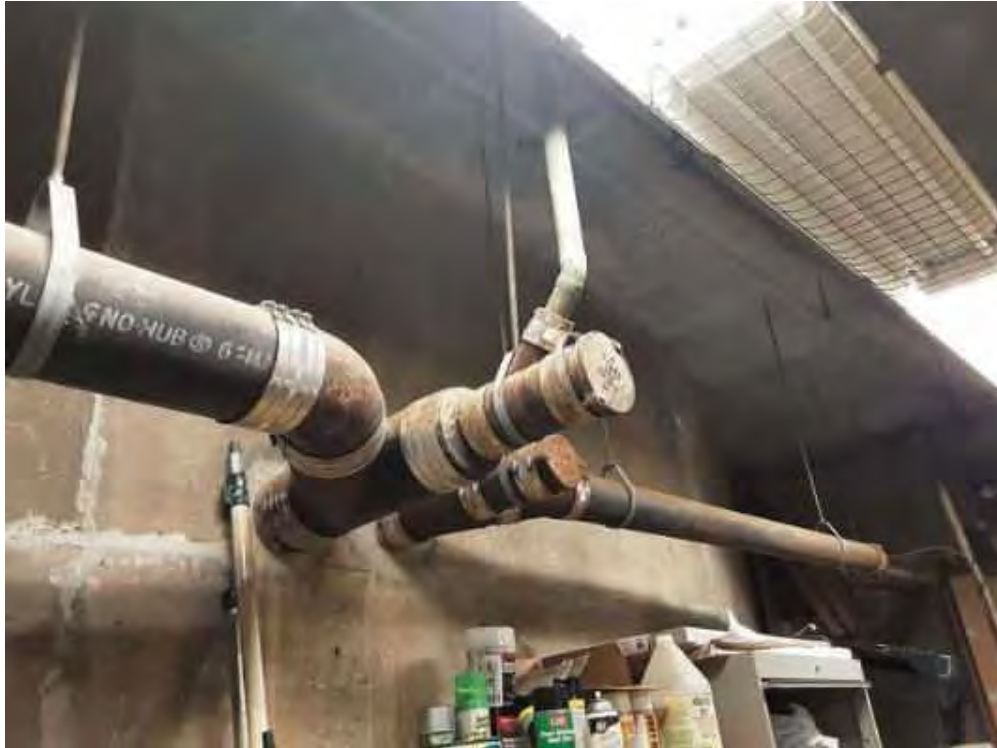
V0000 (None), Piping, Rainwater Leader, Not Insulated, Storage (Location #: 43)
