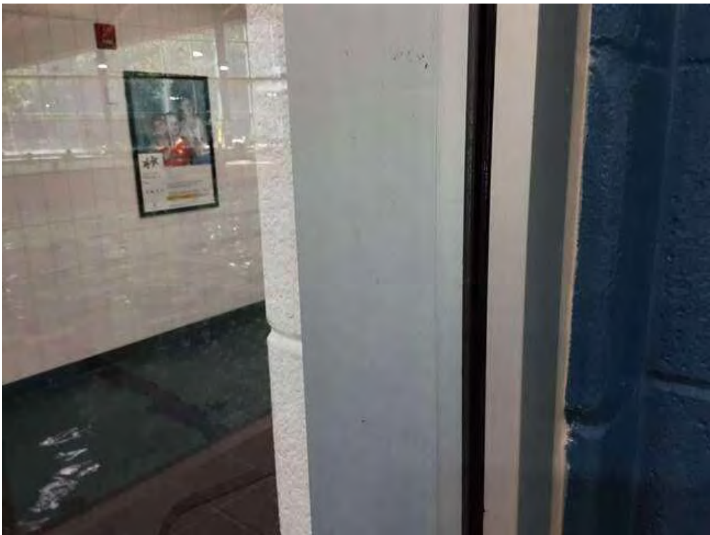
V0004 (None), Other, Window, Caulking, Pool (Location #: 62) between window frame and glass
