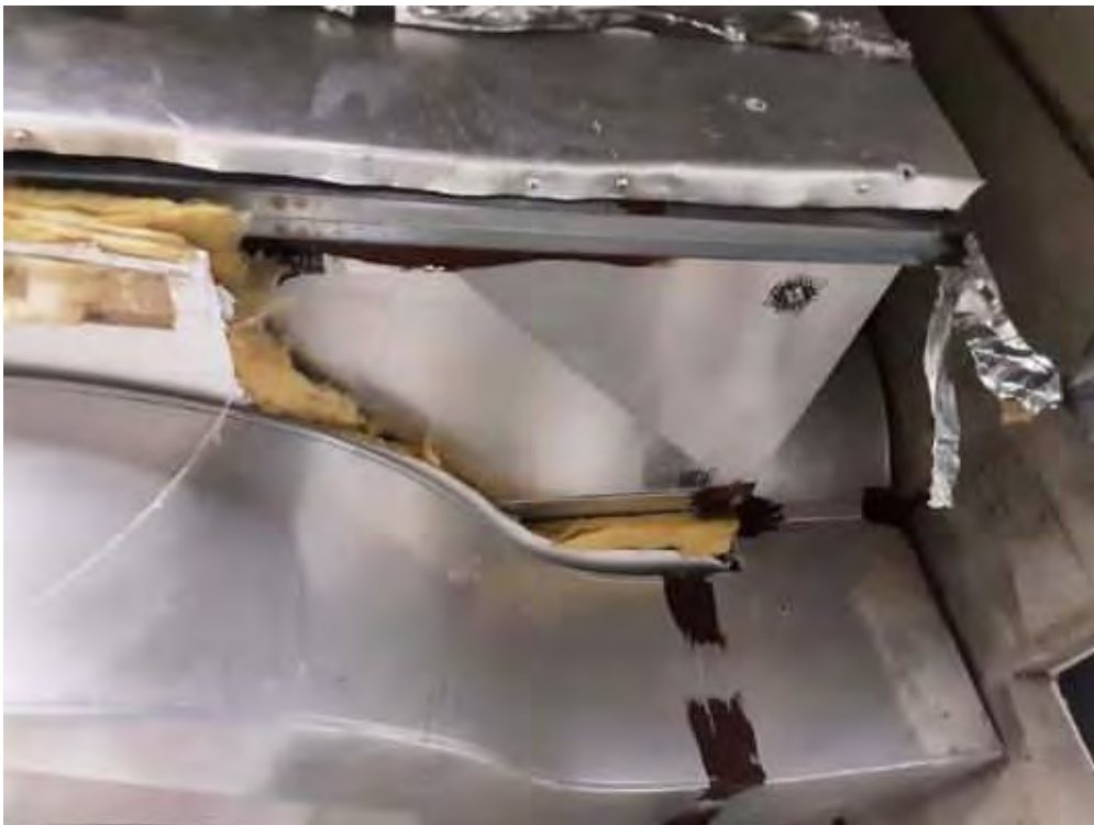
S0010B (None), Duct, Mastic, Filtration Room (Location #: 44) 40 duct connections
