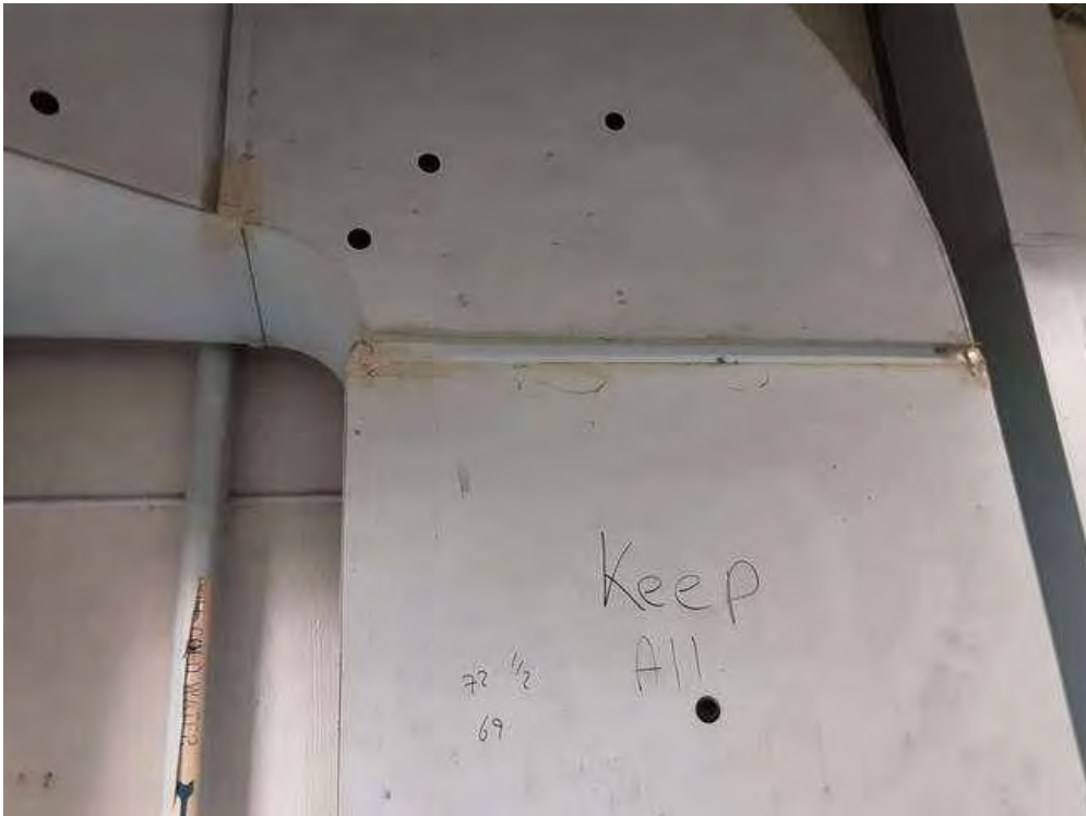
Metal, Sky blue, V0004, Mechanical Room 2 (Location #: 55)
