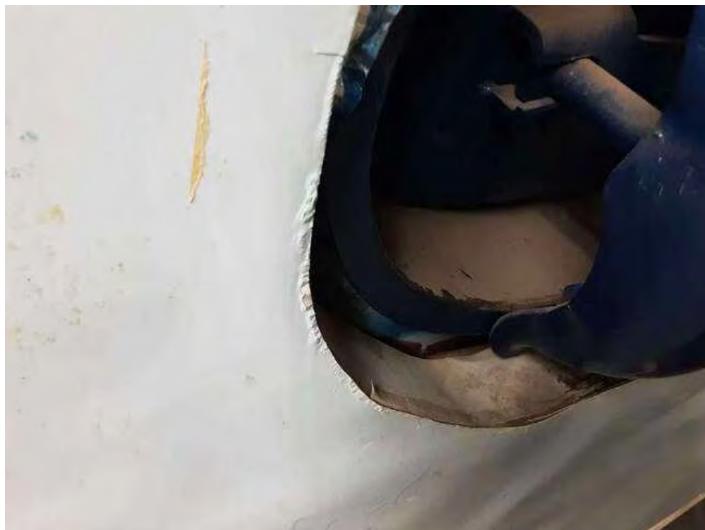
V0000 (None), Mechanical Equipment, Tank, Fibreglass, MechanicalRoom2 (Location #: 55) Storage tank
