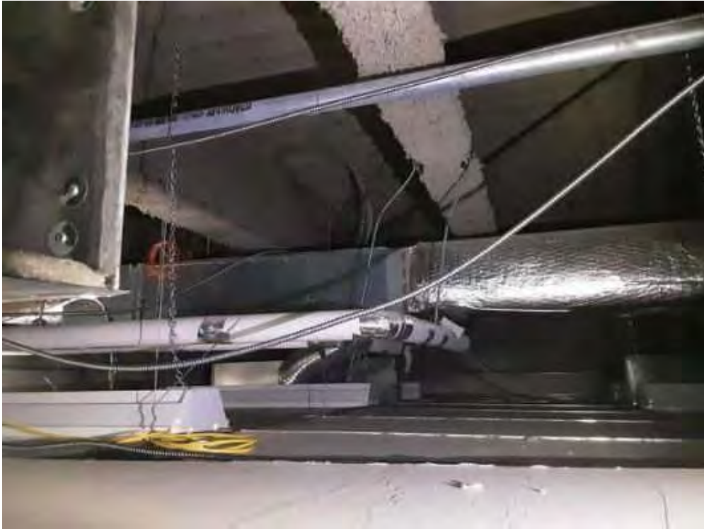
V0000 (None), Piping, Fibreglass, Staff Offices (Location #: 22)
