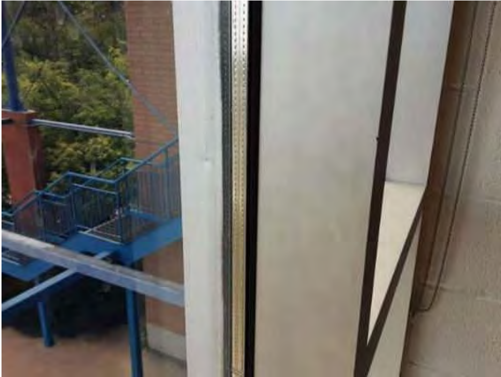
V0002 (None), Other, Window, Caulking, Fitness Center (Location #: 50) Between window frame and glass
