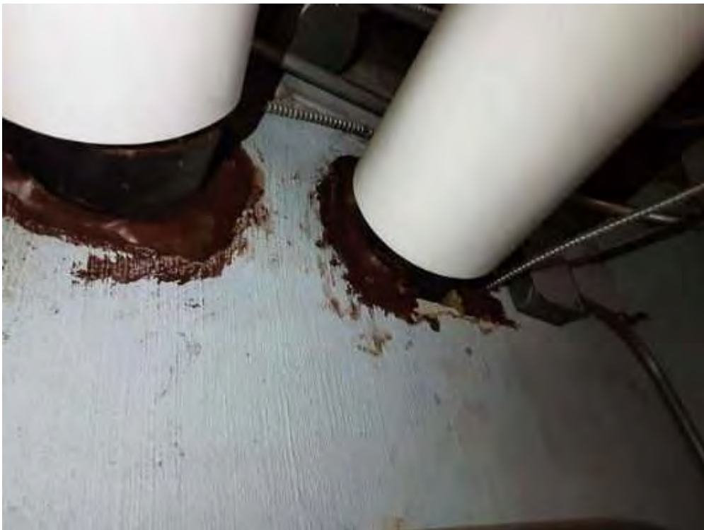
S0012B (None), Piping, Fire Stop, Caulking, Mechanical Room 1 (Location # 57)
