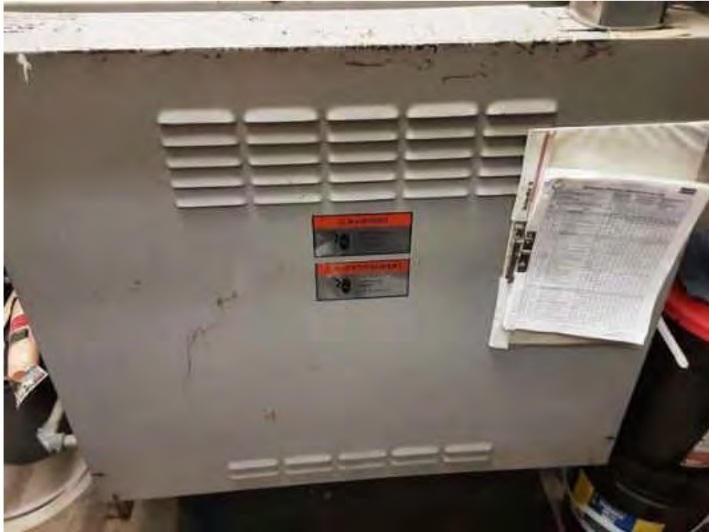
V0000 (None), Mechanical Equipment, Generator Unit, Not Insulated, Elevator Room (Location #: 42) Hydraulic Elevator machine
