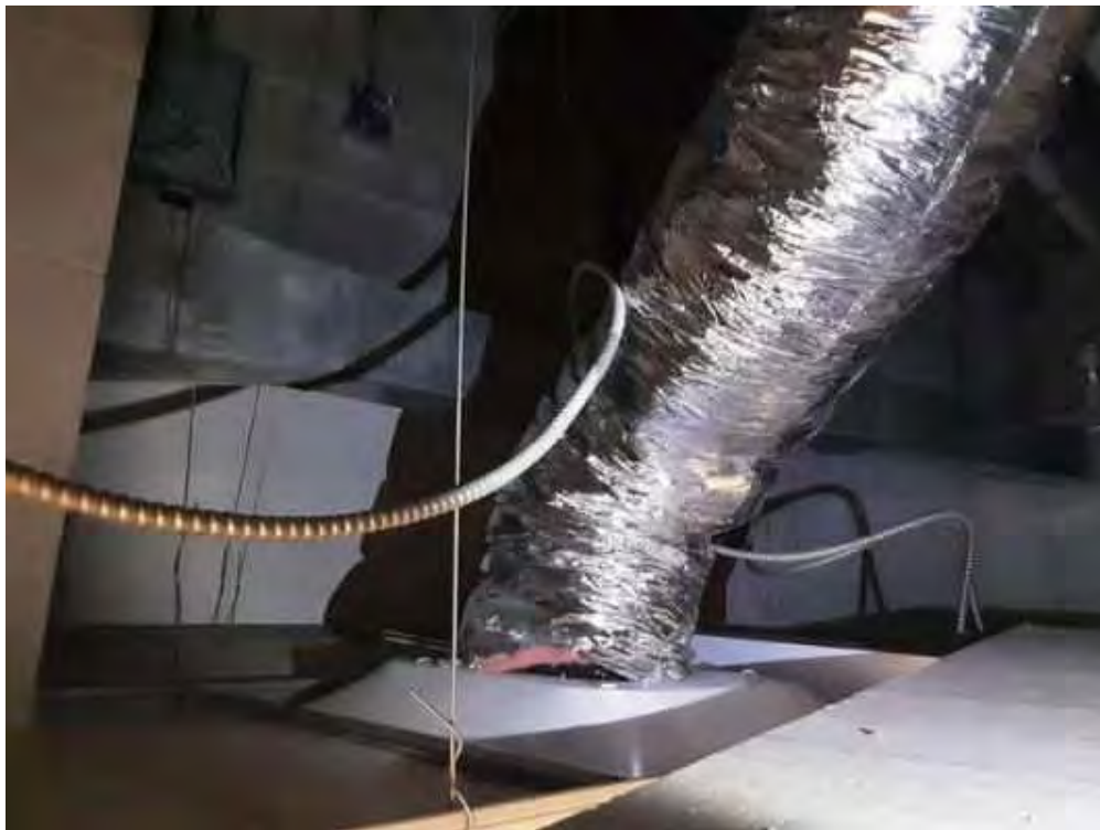
V0000 (None), Duct, Fibreglass, Washrooms (Location # 37)
