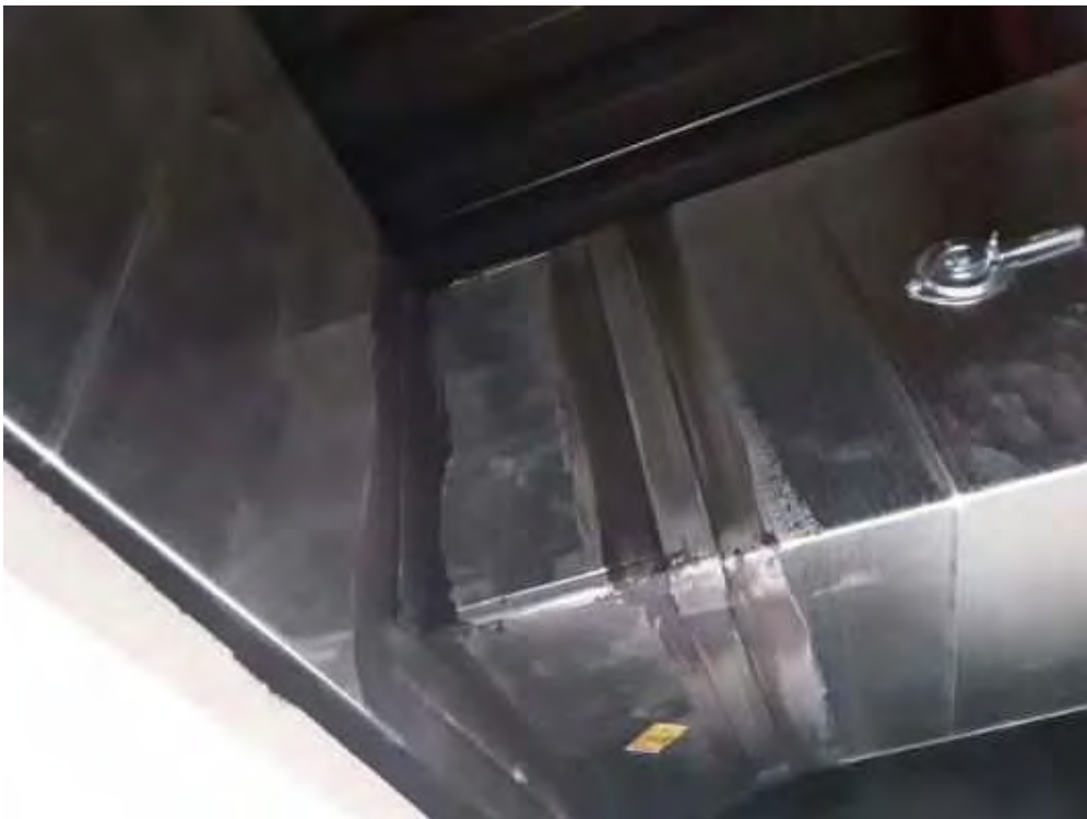
V0009 (None), Duct, Mastic, Grey, Seniors Room (Location #: 38) Approx 8 duct connections
