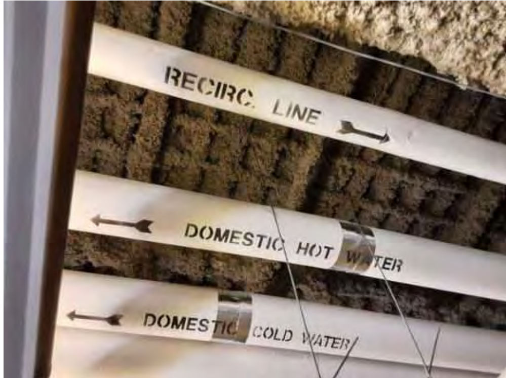
V0000 (None), Piping, Fibreglass, Men's Pool Change Room (Location#: 18) D.C.W, D.H.W, heating supply and return, recirc. line
