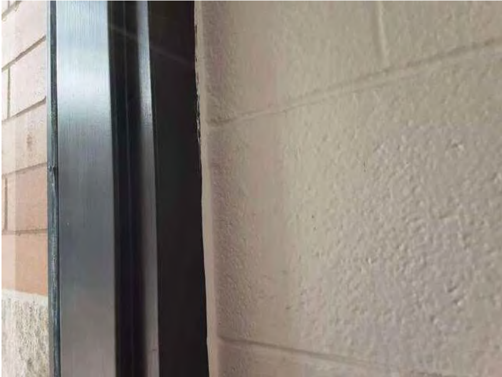
V0008 (None), Wall, Window, Caulking, Rear Vestibule (Location #: 40) Between wall and windowframe
