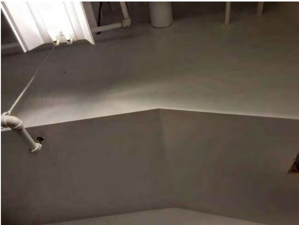
V0000 (None), Ceiling, Bulkhead, Drywall and joint compound, Janitor (Location #: 52)
