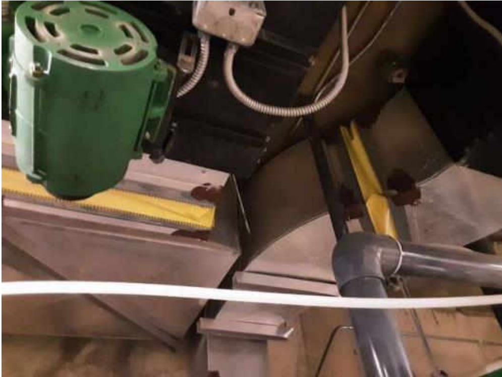
V0000 (None), Duct, Duct Connector, Textile, Filtration Room (Location #: 44)
