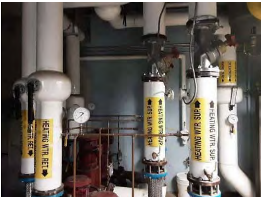
V0000 (None), Piping, Fibreglass, Mechanical Room 2 (Location #: 55)
