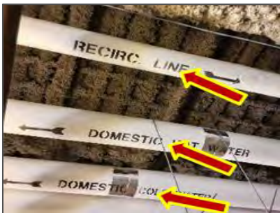
Photo 3: View of non-asbestos fibreglass insulated piping present in the Men's Pool Change Room (Loc. 18).
