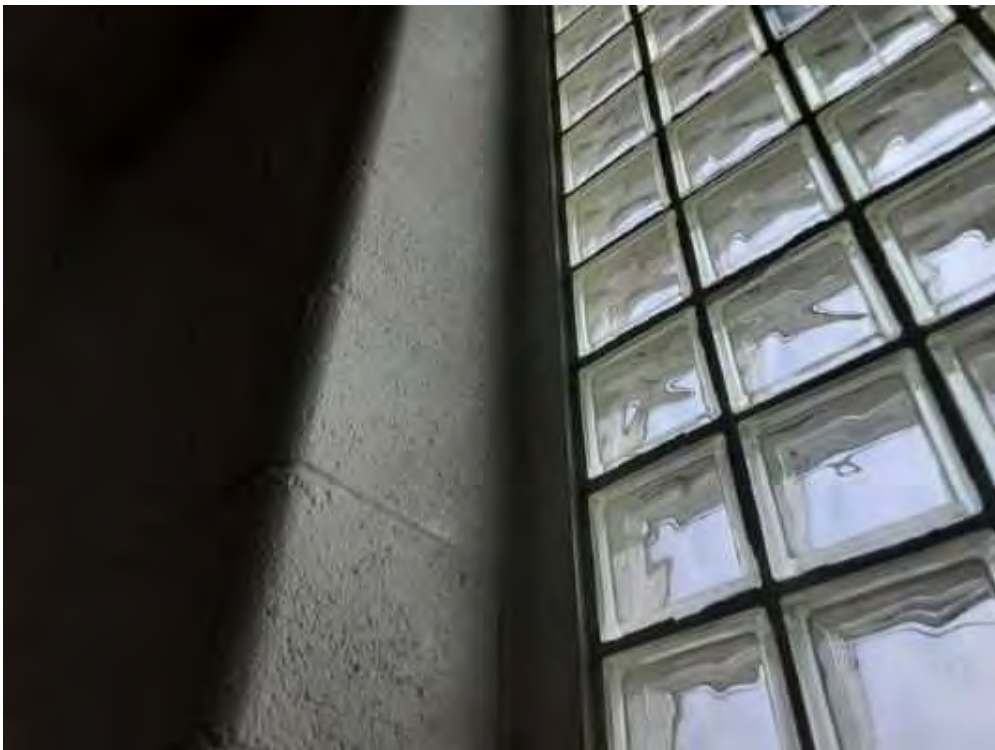
V0008 (None), Wall, Window, Caulking, Staircase (Location #: 21) Between wall and windowframe
