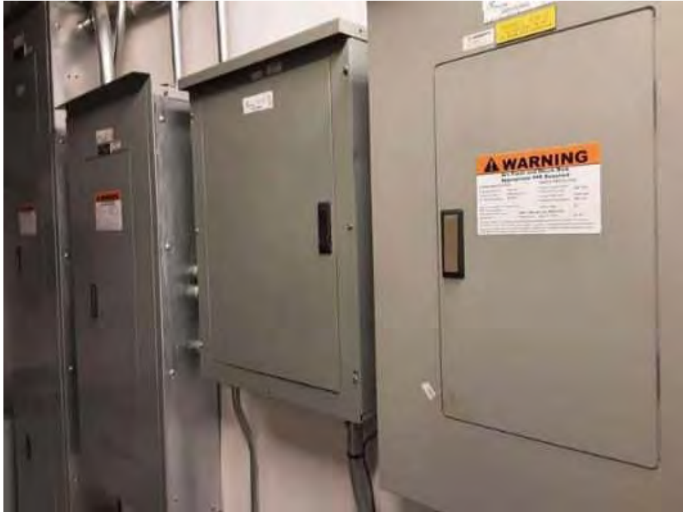
V0000 (None),Other,Electrical Panel,Not Insulated,Electrical Room (Location#: 53)
