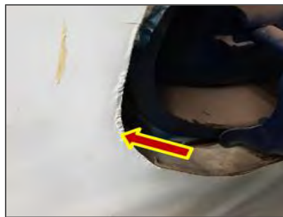
Photo 10: View of fibreglass insulated tank present in the Mechanical Room 2 (Loc. 55).
