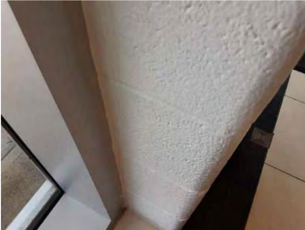
S0001A (None), Wall, Window, Caulking, Entrance Corridor (Location #: 2) Between window frame and wall
