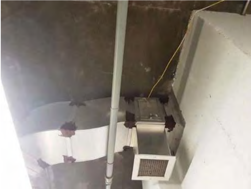
V0010 (None), Duct, Mastic, Basement Corridor (Location#: 41) 8 duct connections
