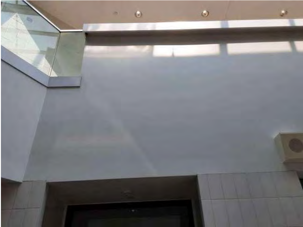
V0000 (None), Wall, All, Drywall and joint compound, Lobby (Location #: 3)
