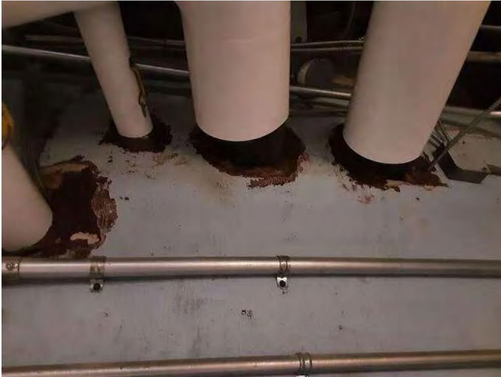
S0012A (None), Piping, Fire Stop, Caulking, Mechanical Room 1 (Location # 57)
