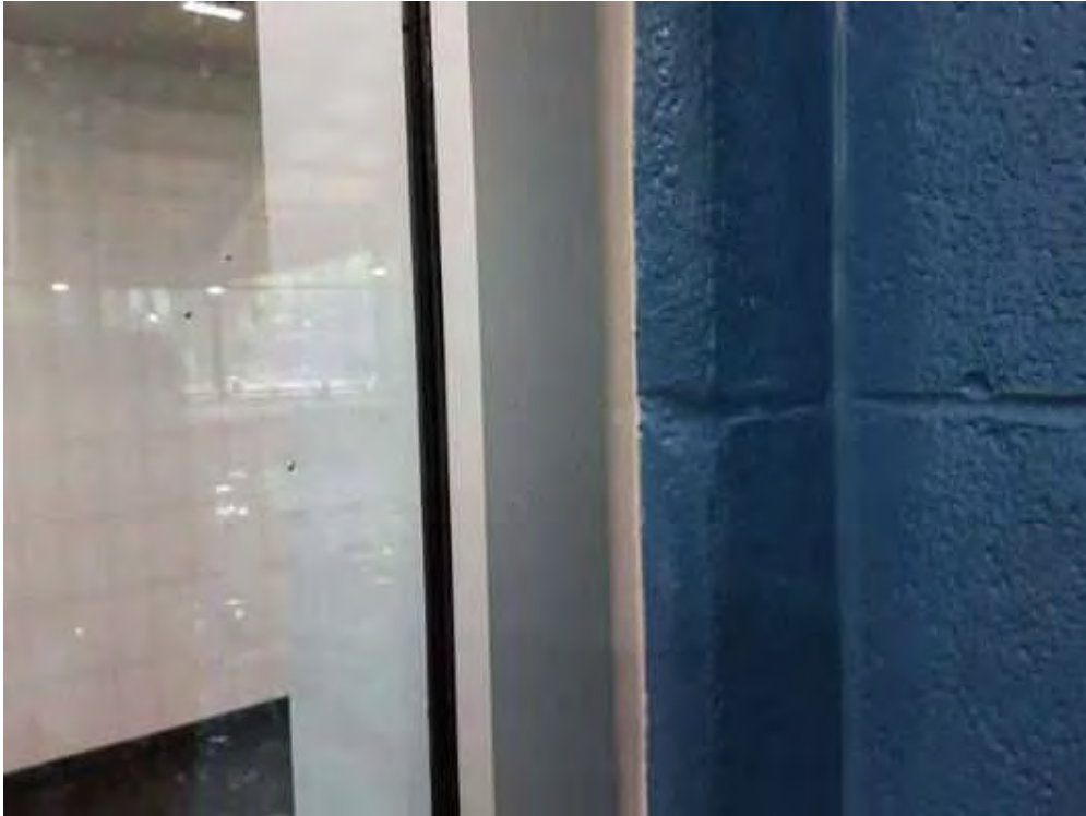
V0001 (None), Wall, Window, Caulking, Pool (Location #: 62) Between window frame and wall
