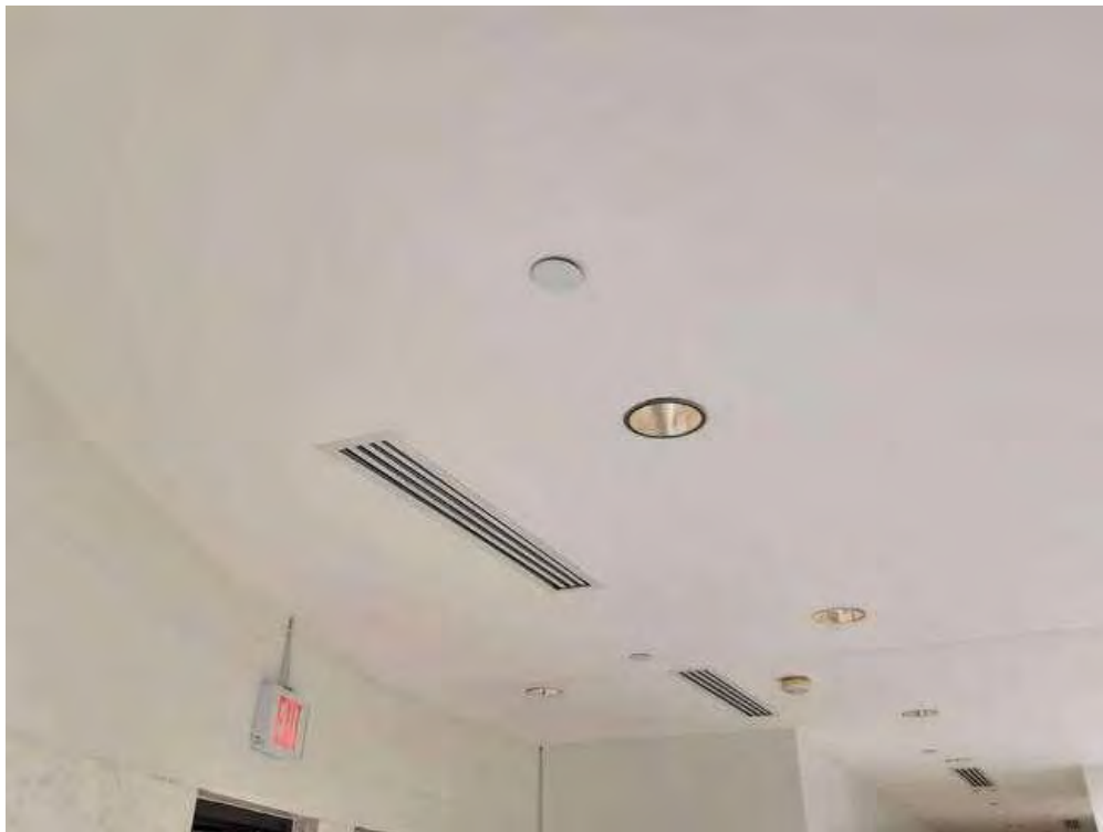
V0000 (None), Ceiling, Drywall and joint compound, Upper Lobby (Location #: 47)
