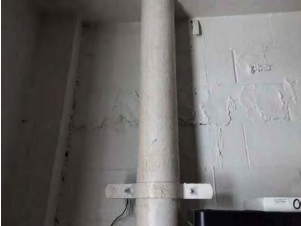
V0000 (None), Piping, Rainwater Leader, Not Insulated, Coat Check (Location #: 4)
