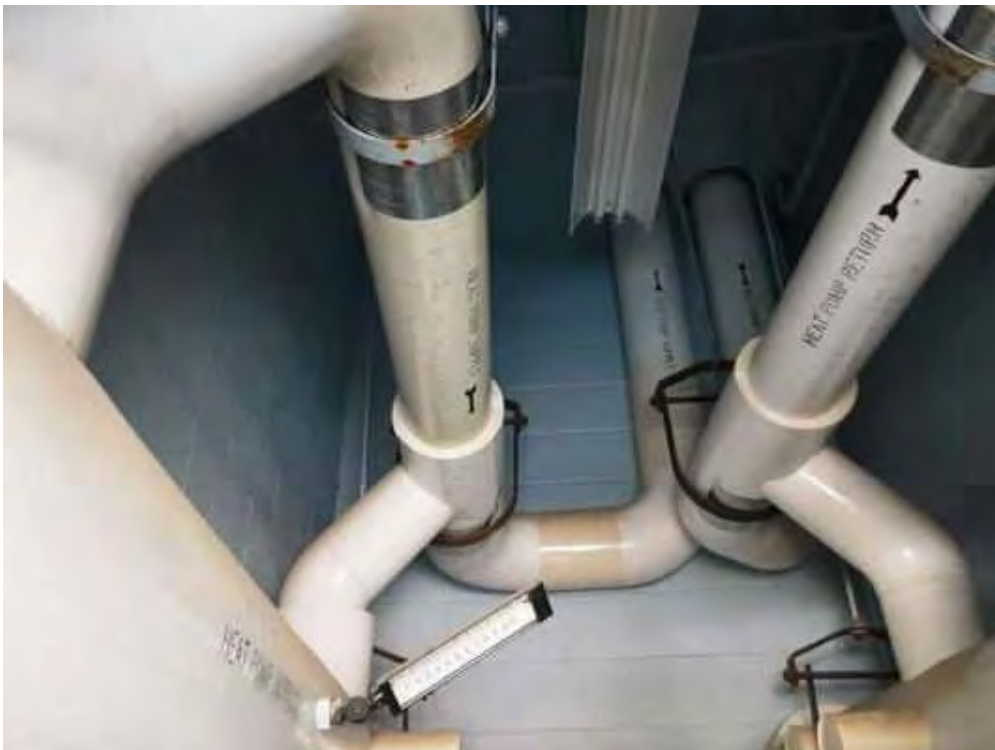
V0000 (None), Piping, All, Fibreglass, Supply Room (Location #: 24) Heat pump supply and return
