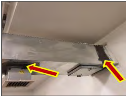
Photo 5: View of non-asbestos grey coloured duct mastic on uninsulated duct present in the Janitor (Loc. 52).
