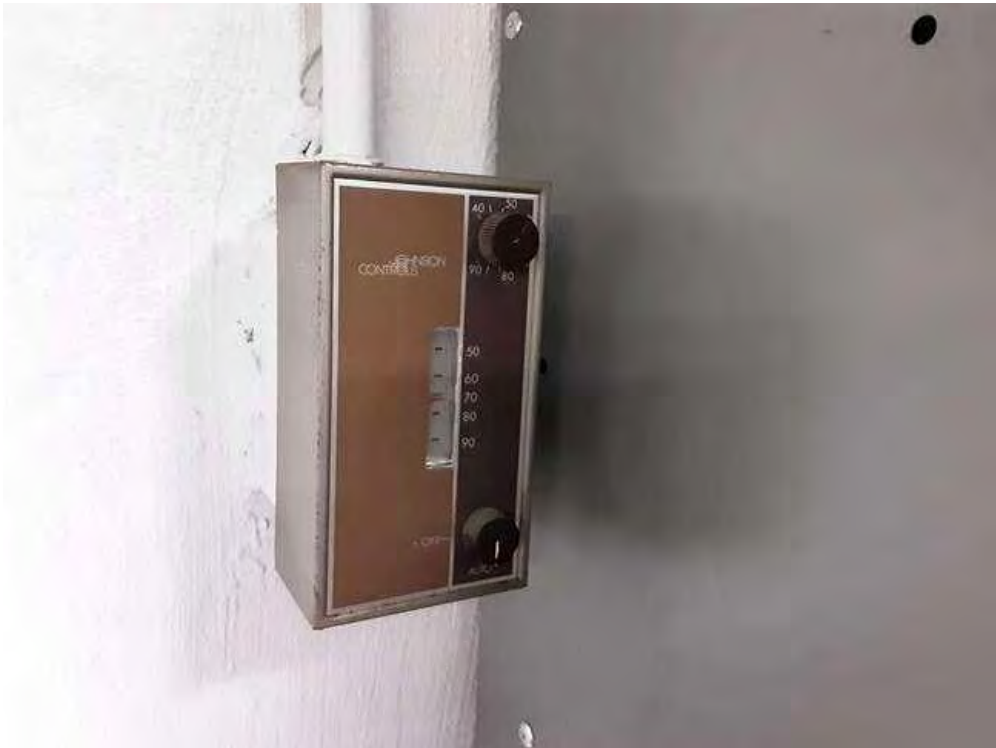
Mercury, Mechanical Room 2(Location #: 55)
