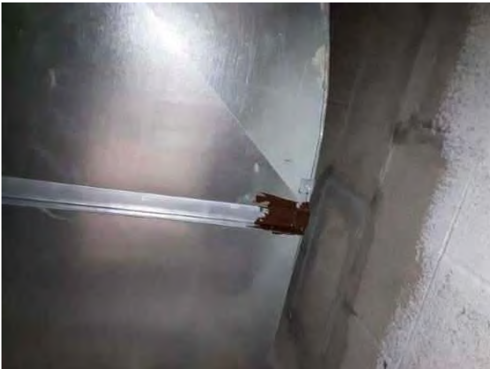
S0010A (None), Duct, Mastic, Seniors Room (Location #: 38) Accessible in kitchen area, 8 duct connections
