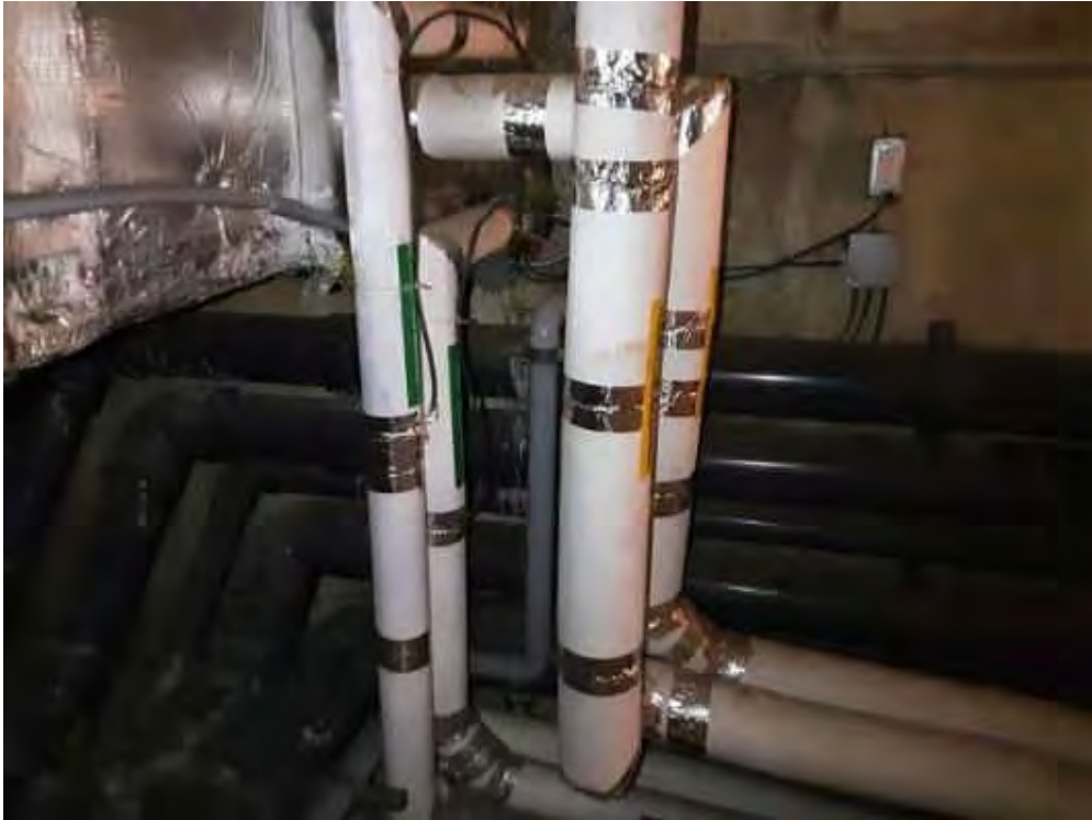
V0000 (None), Piping, Fibreglass, Tunnel (Location #: 45)
