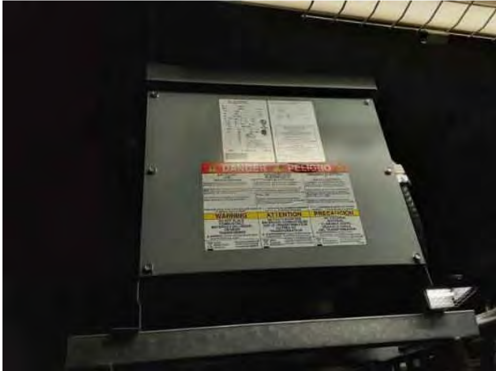
PCB, Filtration Room (Location #: 44)
