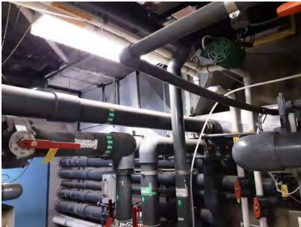
V0000 (None), Piping, Polyvinylchloride (PVC), Filtration Room (Location #: 44)
