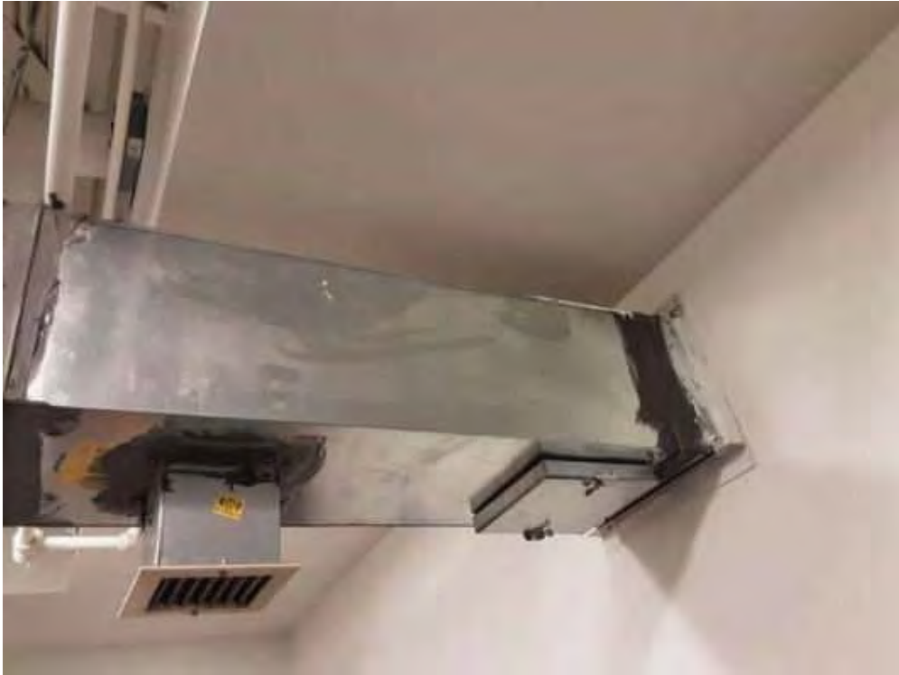
S0009C (None), Duct, Mastic, Grey, Janitor (Location #: 52) 6 duct connections
