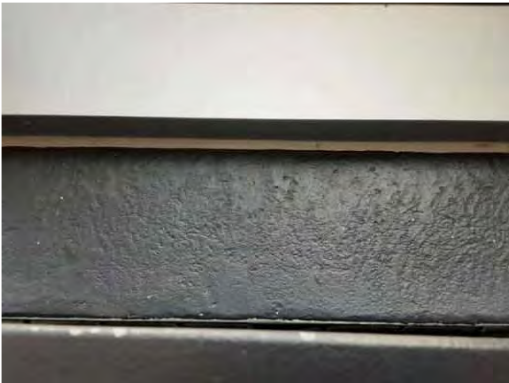
V0001 (None), Wall, Window, Caulking, Fitness Studio (Location #: 51) Between window frame and floor
