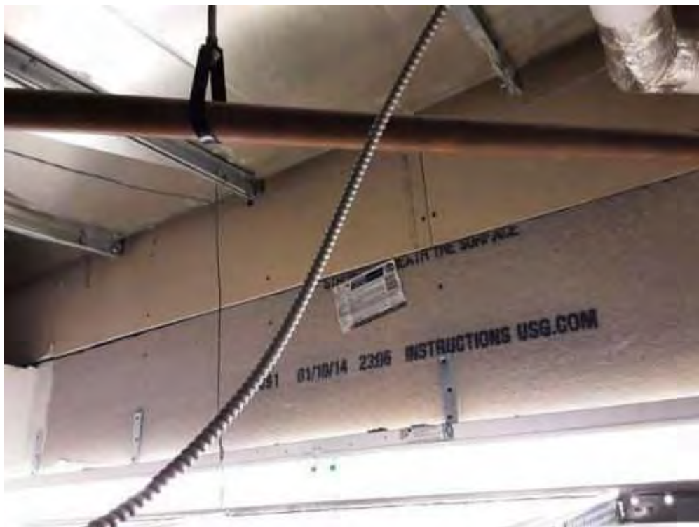
V0000 (None), Wall, Cement Product, Universal Washrooms (Location #: 49) Cement board, dated 01/10/14, contains silica
