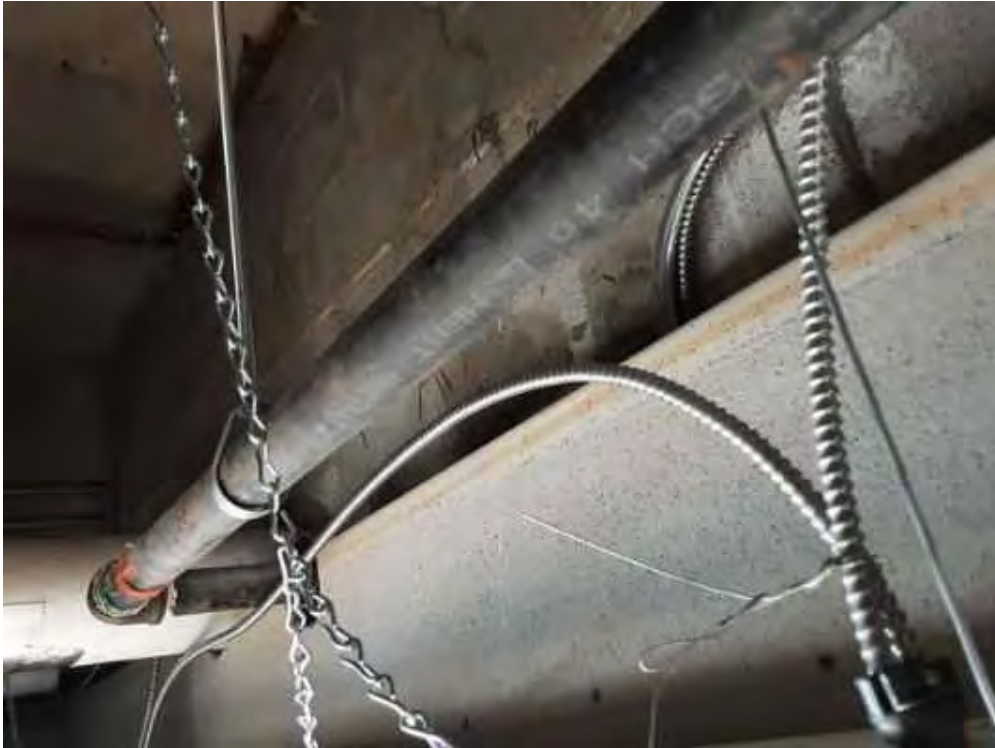
V0000 (None), Piping, Sprinkler, Not Insulated, Entrance Corridor (Location #: 2)
