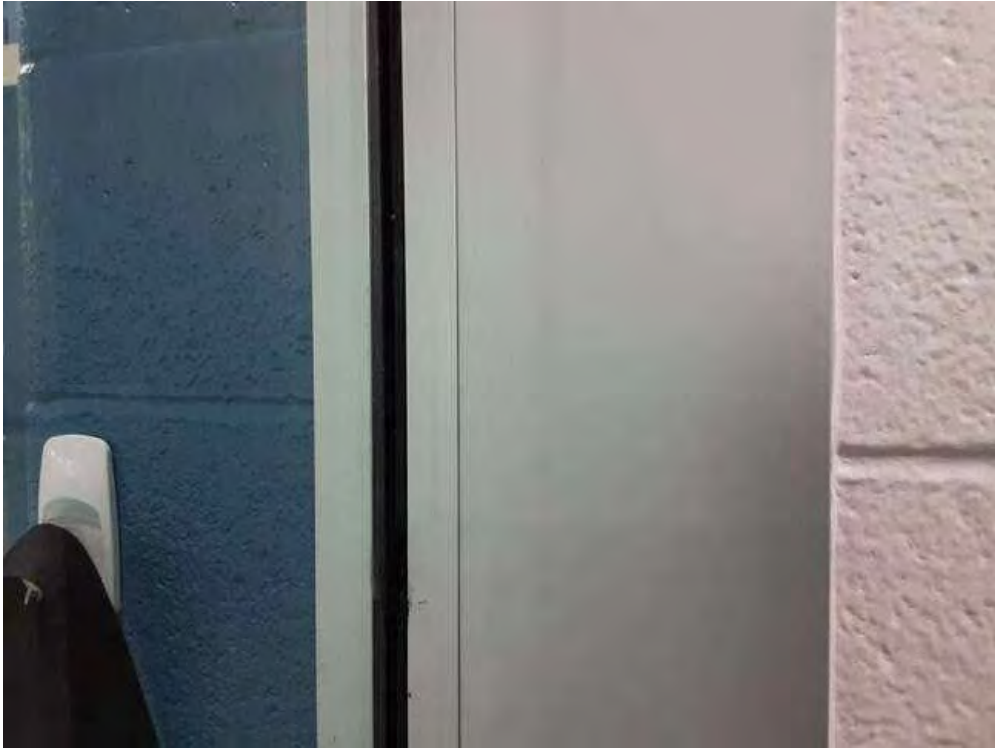
S0004A (None), Other, Window, Caulking, Lobby (Location #: 3) between window frame and glass
