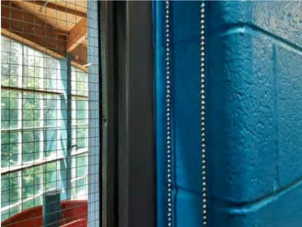
V0008 (None), Wall, Window, Caulking, Fitness Center (Location #: 50) Between window frame and wall
