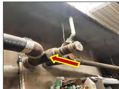
Photo 4: View of uninsulated piping present in the Storage (Loc.43).
