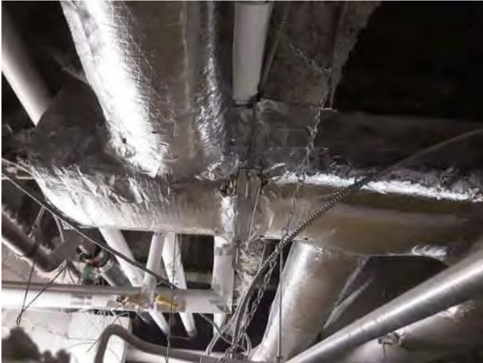
V0000 (None), Piping, Fibreglass, Men's Fitness Change Room (Location #: 15) D.C.W, D.H.W, heating supply and return, recirc. line
