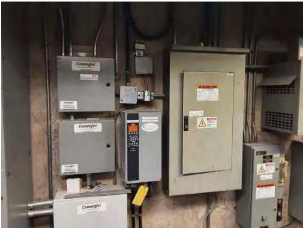
V0000 (No ne), Other, Electrical Panel, Not Insulated, Filtration Room (Location #: 44)
