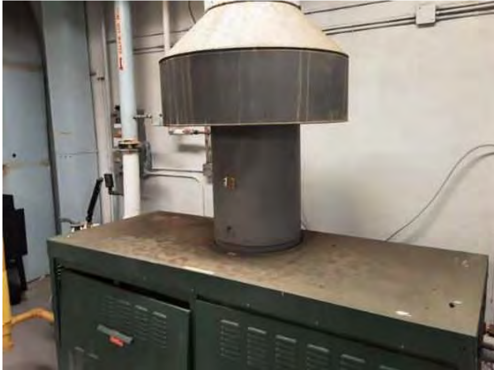
V0000 (None), Mechanical Equipment, Not Insulated, Mechanical Room 2 (Location #: 55)
