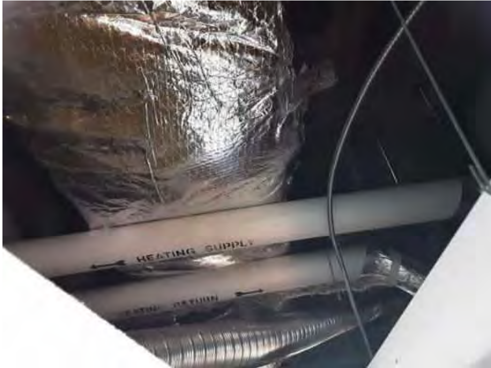
V0000 (None), Piping, Fibreglass, Lobby (Location #: 3) Heating supply and return
