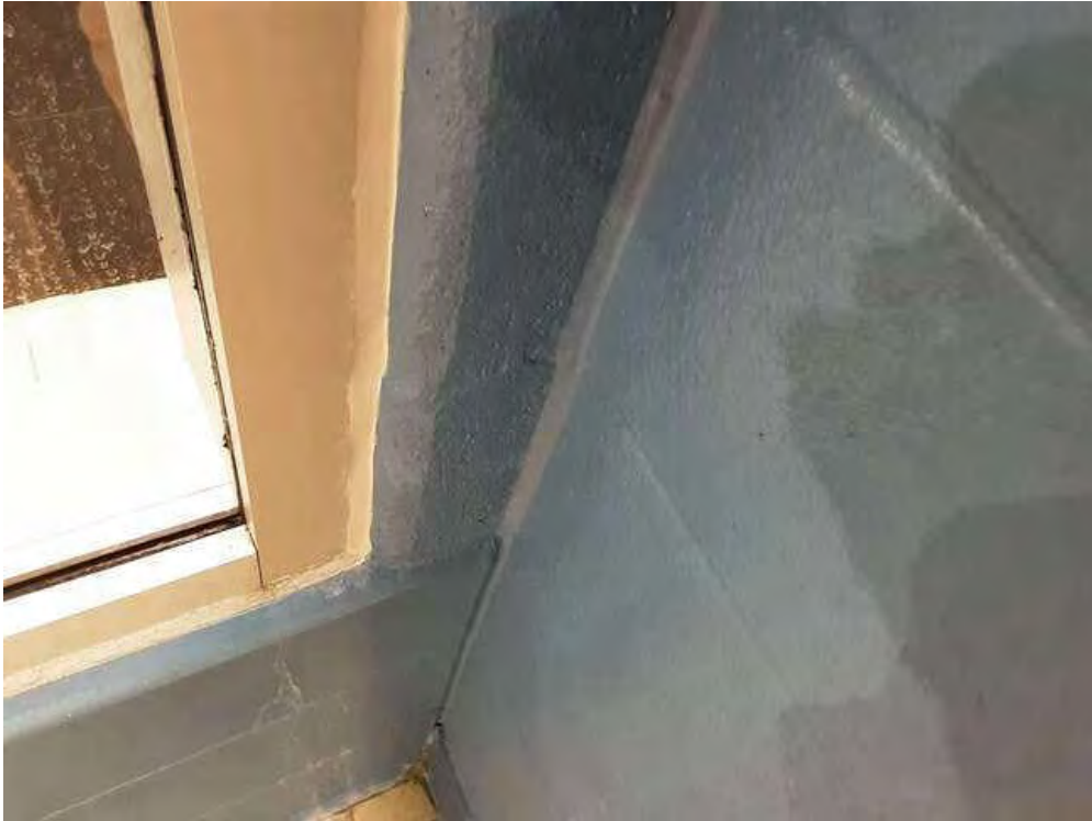
V0008 (None), Wall, Window, Caulking, Pool (Location #: 62) Between window frame and wall
