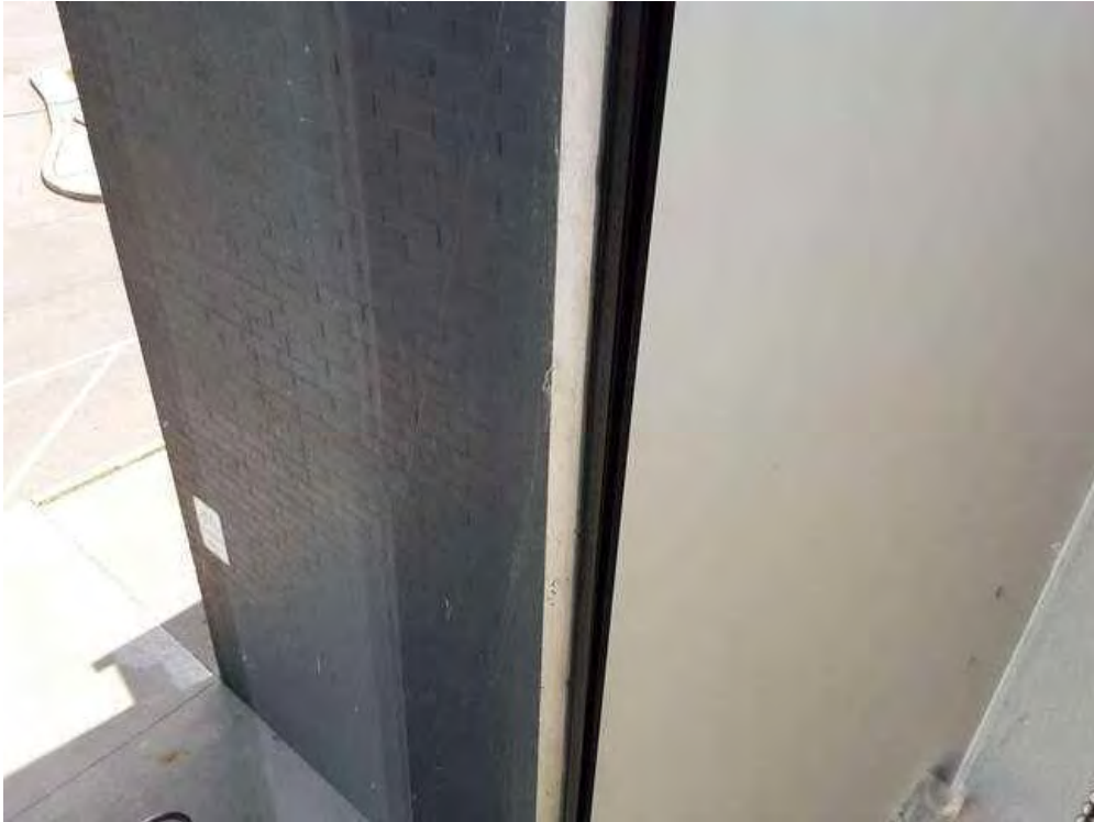
V0000 (None), Other, Window, Styrofoam, Fitness Studio (Location #: 51) Type of foam, between window frame and glass
