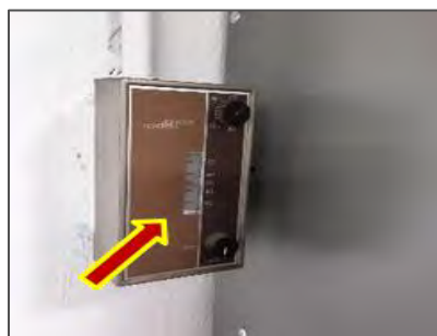
Photo 16: View of non-mercury containing thermostat present in the Mechanical Room 2 (Loc. 55).
