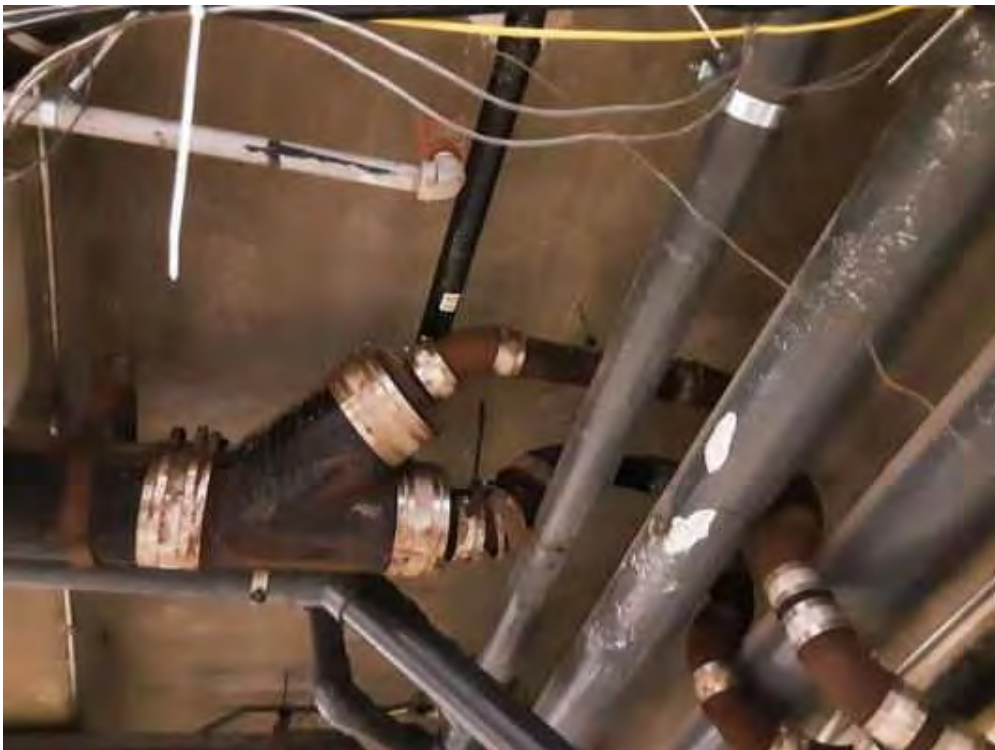
V0000 (None), Piping, Rainwater Leader, Not Insulated, Filtration Room (Location #: 44)
