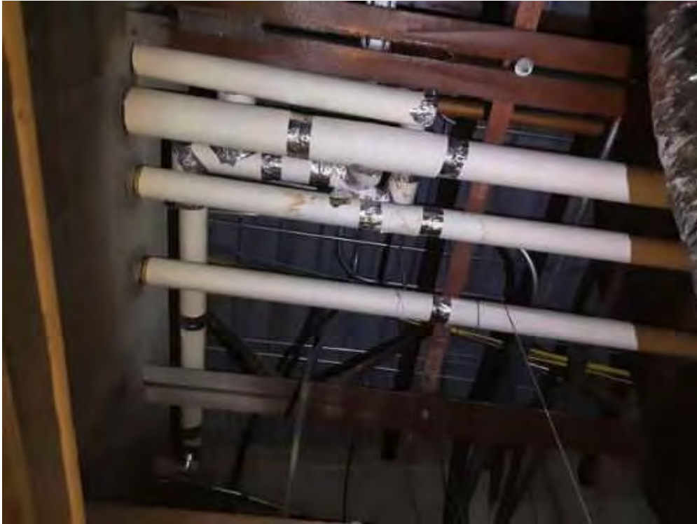
V0000 (None), Piping, Fibreglass, Washrooms (Location #: 37)
