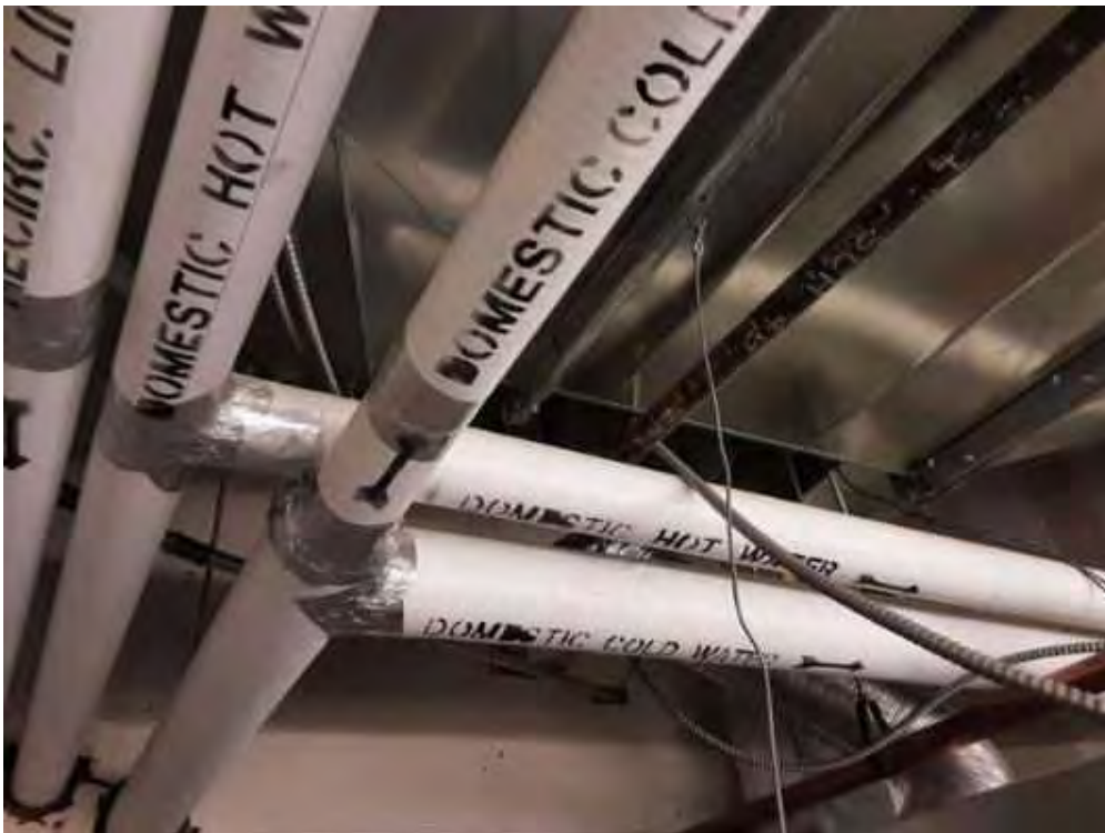
V0000 (None), Piping, Fibreglass, Universal Washrooms (Location #: 49)
