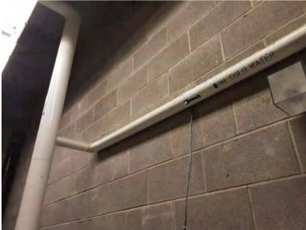
V0000 (None), Piping, All, Fibreglass, Sprinkler Room (Location #: 36) D.C.W
