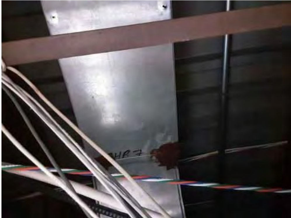
V9500 (Presumed Asbestos), Duct, Mastic, Burt Arts Studio (Location #. 29) Not accessible with 6ft ladder
