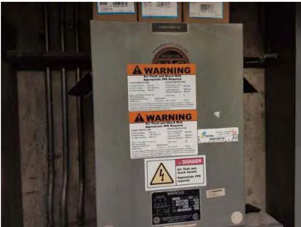
PCB, Filtration Room (Location #: 44)
