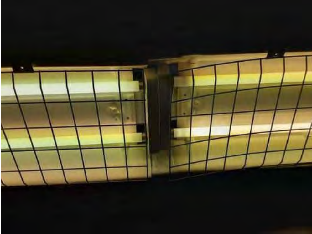
Mercury, Mechanical Room 2(Location #: 55)
