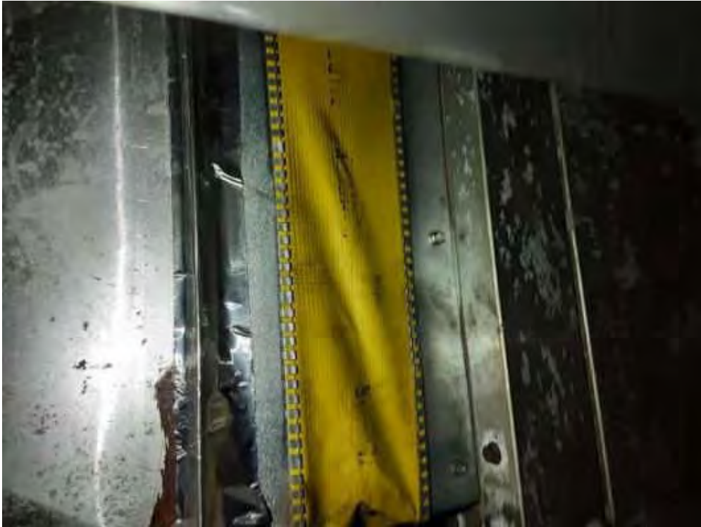
V0000 (None), Duct, Duct Connector, Textile, Tunnel (Location #: 45)
