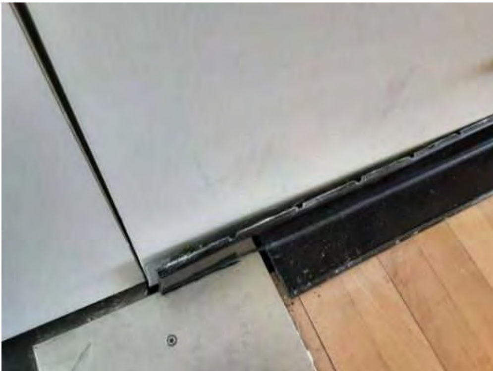
S0011B (None), Wall, Base, Mastic, Fitness Studio (Location #: 51)
