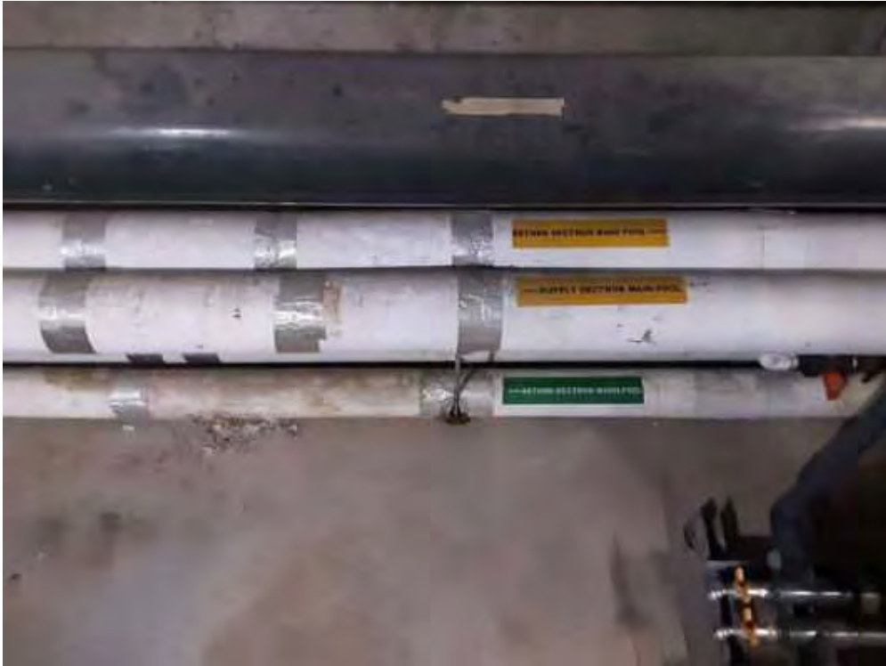
V0000 (None), Piping, Fibreglass, Filtration Room (Location #: 44)
