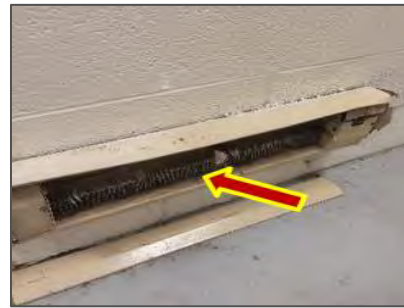
Photo 9: View of uninsulated unit heater present in the Youth Storage (Loc. 35).
