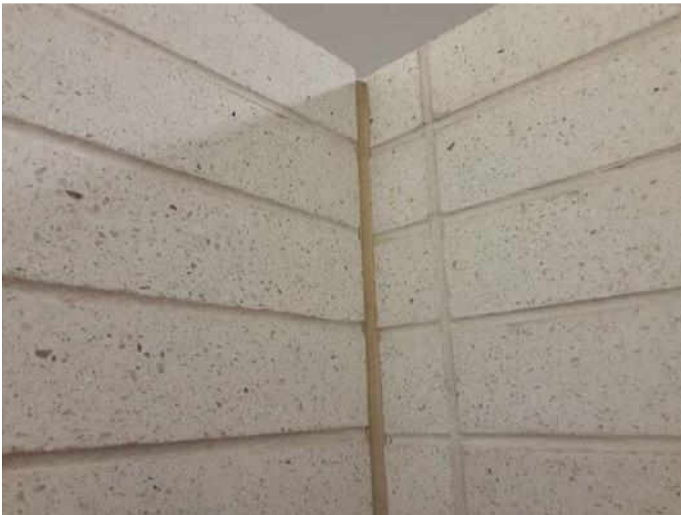
S0003B (None), Wall, Expansion Joint, Caulking, Family Change Room (Location #: 13)
