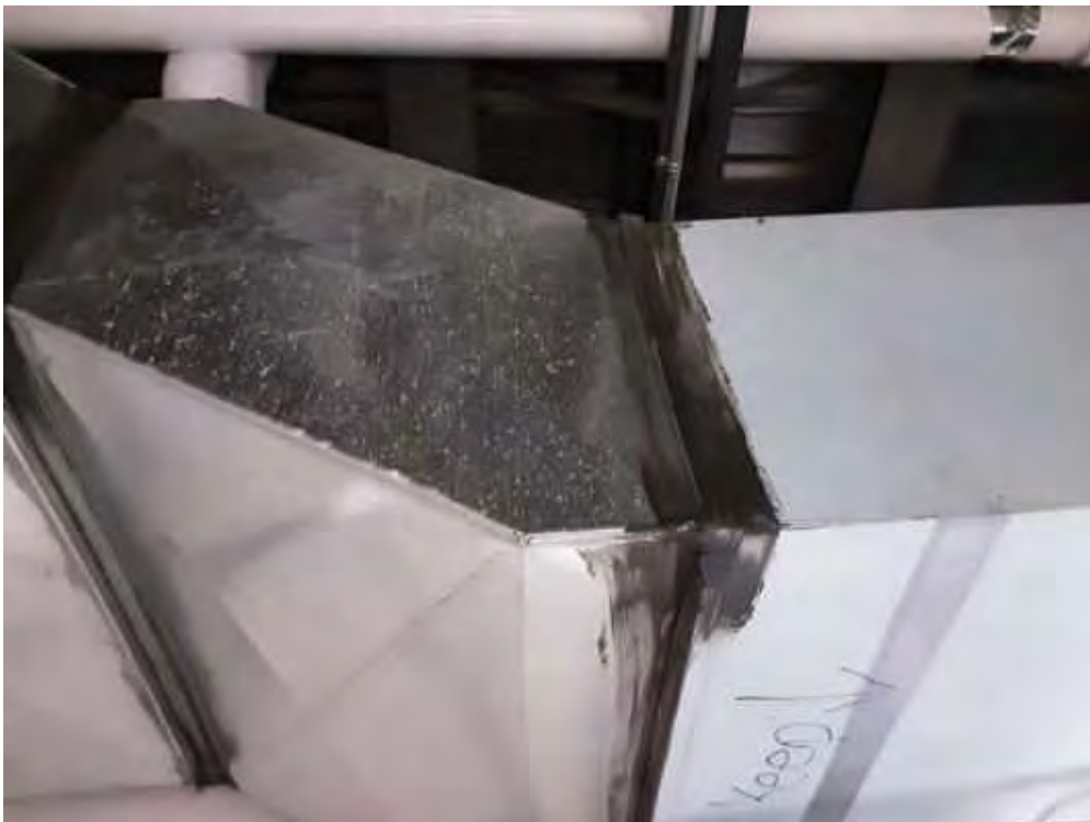
V0009 (None), Duct, Mastic, Mechanical Room 2 (Location #: 55) 5 duct connections
