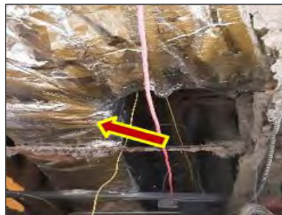
Photo 7: View of non-asbestos fibreglass in insulated duct present in the Lobby (Loc. 3).
