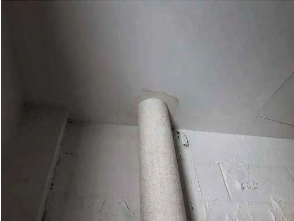
V0000 (None), Ceiling, All, Drywall and joint compound, Coat Check (Location #: 4) Water staining observed
