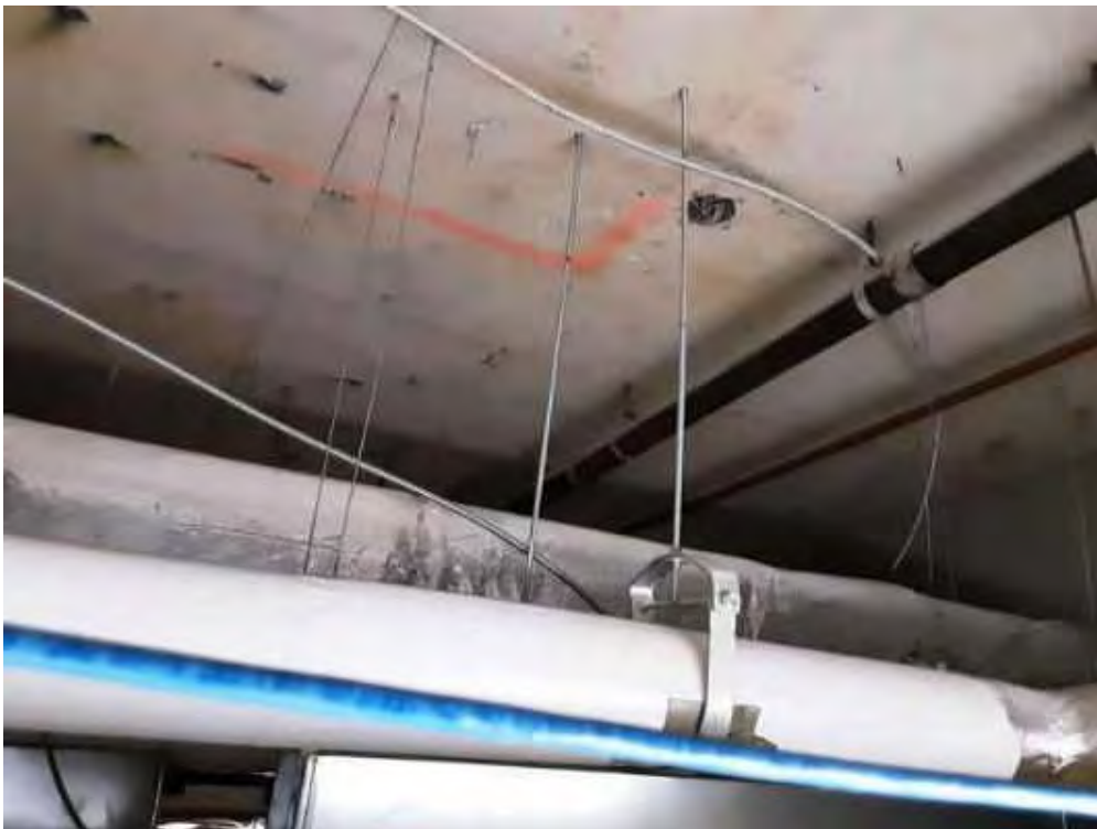
V0000 (None), Duct, All, Fibreglass, Entrance Corridor (Location #: 2)
