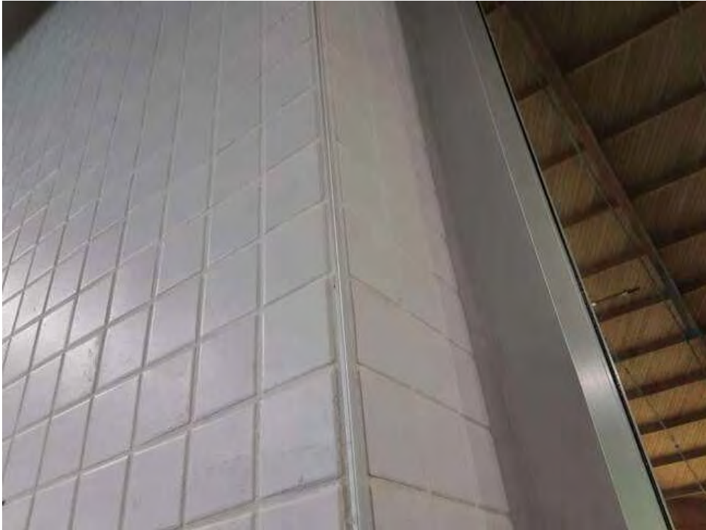
V0001 (None), Wall, Window, Caulking, Lobby (Location #: 3) Between window frame and wall
