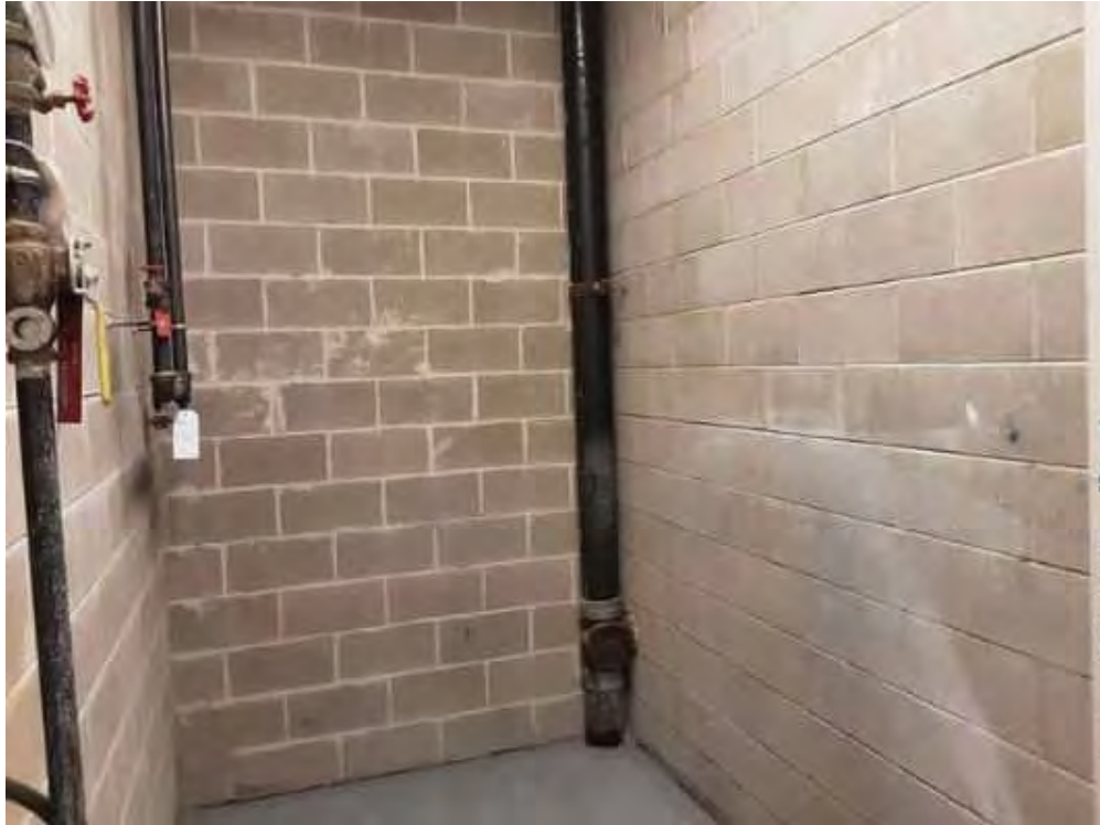
V0000 (None), Piping, Rainwater Leader, Not Insulated, Sprinkler Room (Location # 36)
