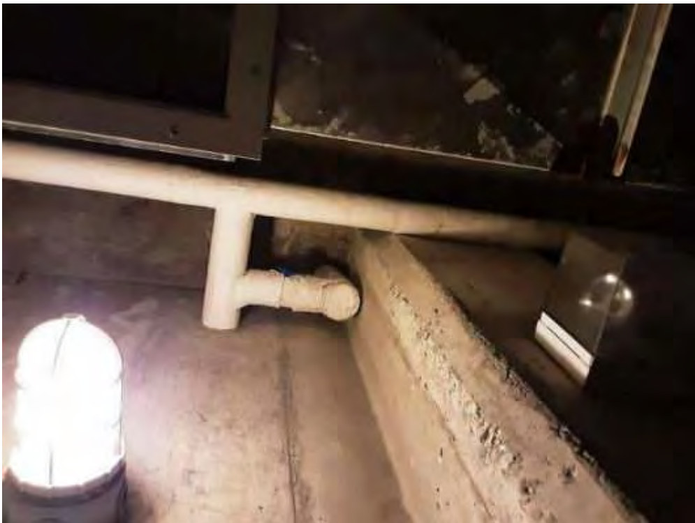
V0000 (None), Piping, Fibreglass, Tunnel (Location #: 45)
