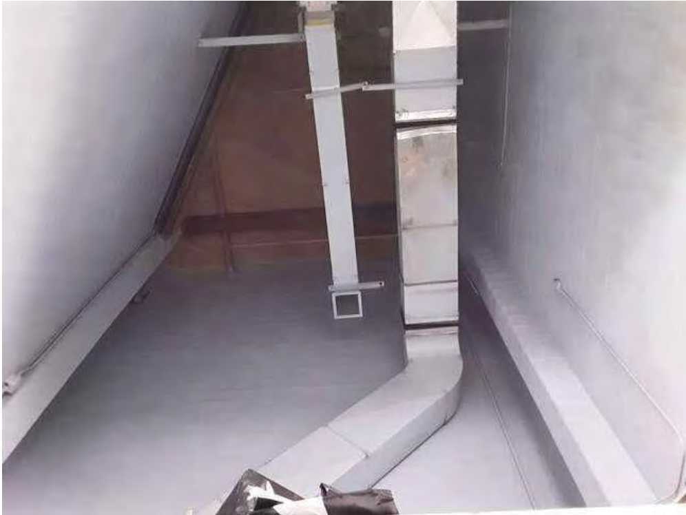
Metal,, V0004, Pool Storage1 (Location #: 63)
