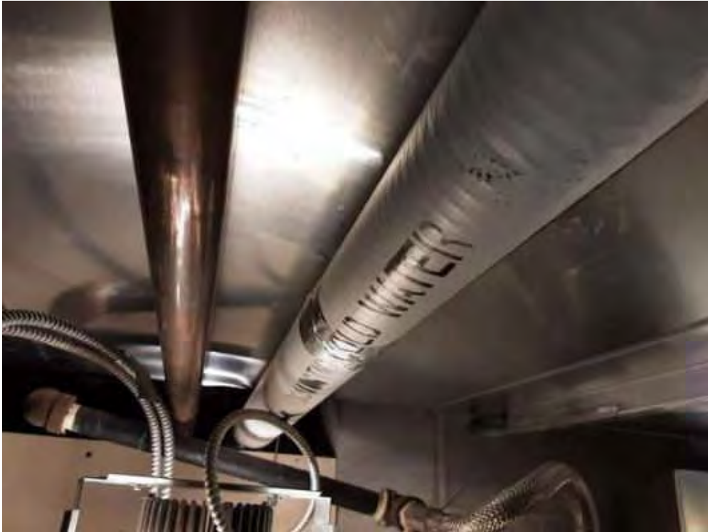
V0000 (None), Piping, Fibreglass, Men's Washroom (Location #: 10) D.C.W
