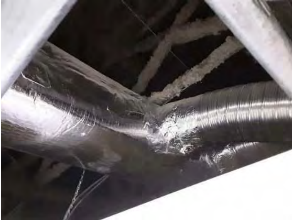
V0000 (None), Duct, Fibreglass, Men's Fitness Change Room (Location#: 15)
