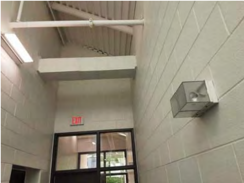
Pb Products, Corridor 4 (Location #: 31)
