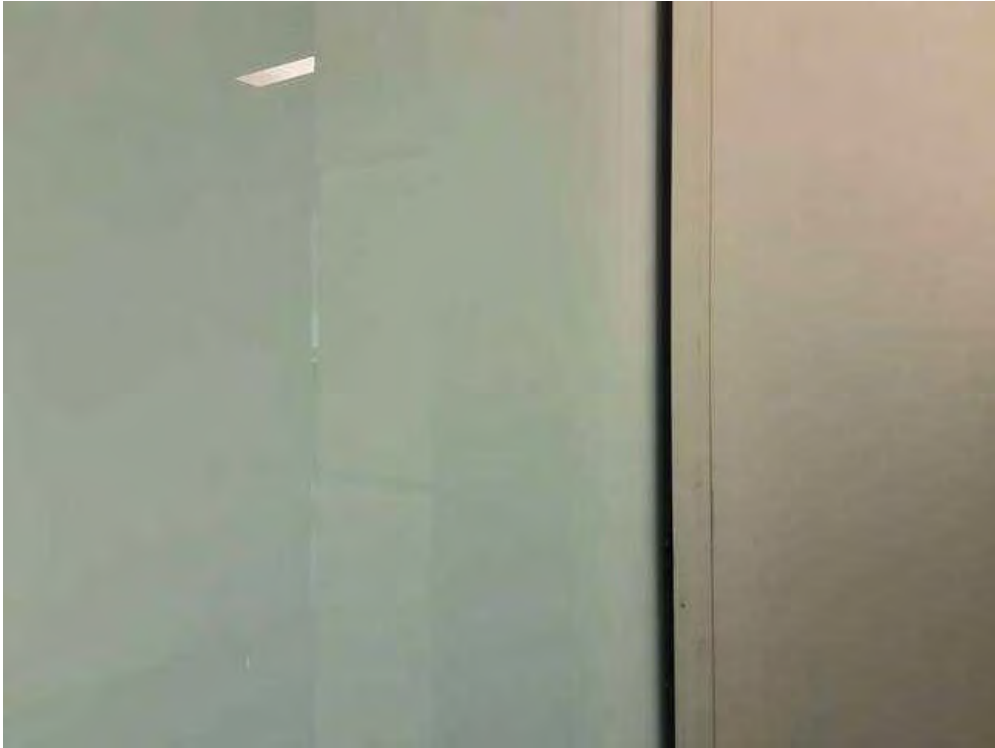
S0004C (None), Other, Window, Caulking, Program Room (Location #: 48) between window frame and glass
