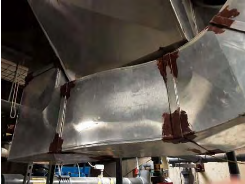
V0010 (None), Duct, Mastic, Filtration Room (Location #: 44)
