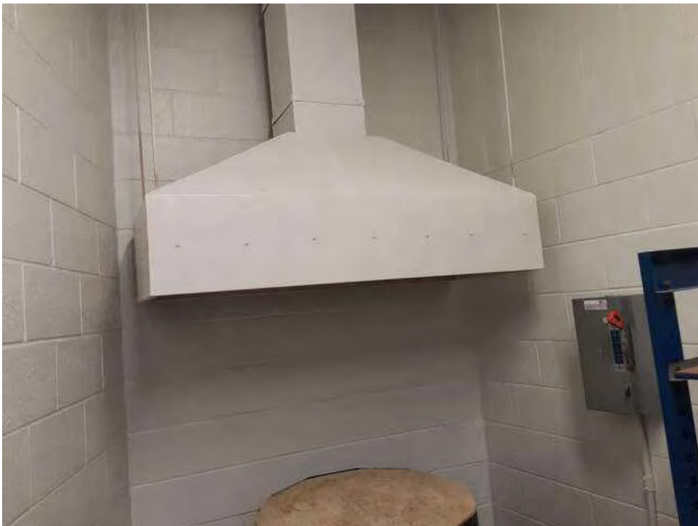
V0000 (None), Mechanical Equipment, Fume hood, Drywall (no compound), Kiln And Storage Room (Location #. 32) In kiln room
