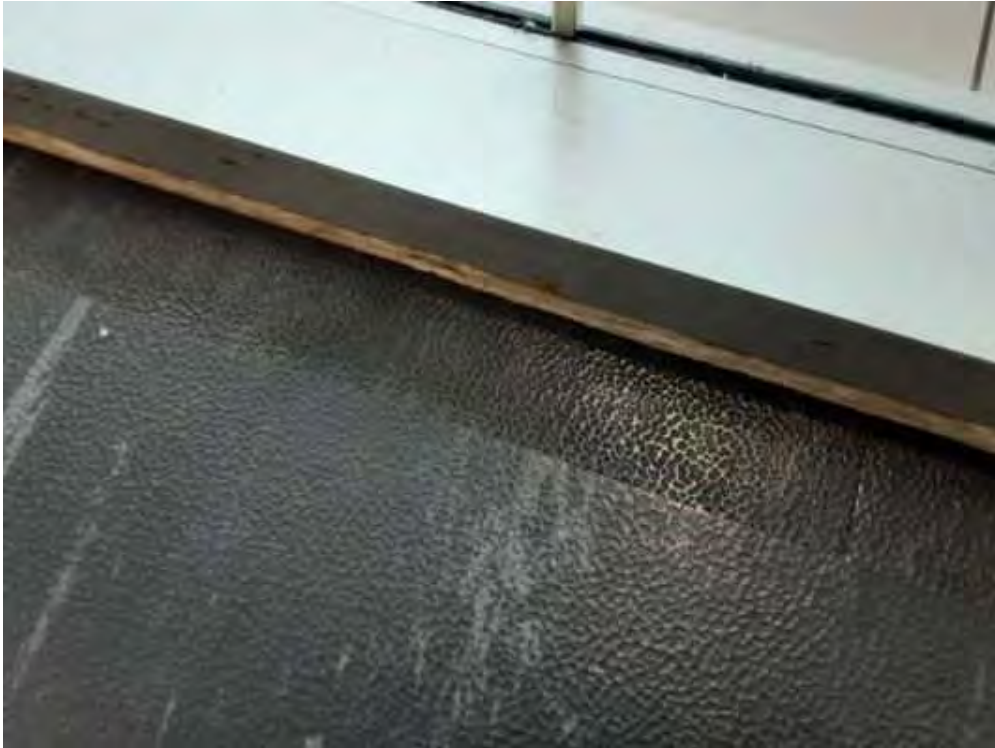
V0003 (None), Wall, Window, Caulking Program Room (Location #: 48) Between window frame and floor
