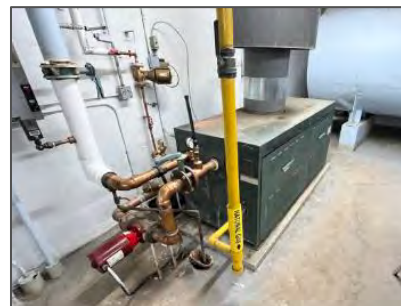
Uninsulated Boiler, Mechanical Room 2 (Loc.55).
