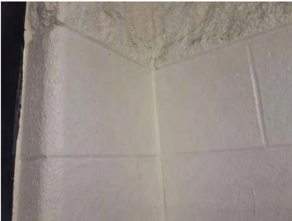
V0003 (None), Wall, Expansion Joint, Caulking, Fitness Center (Location #: 50)
