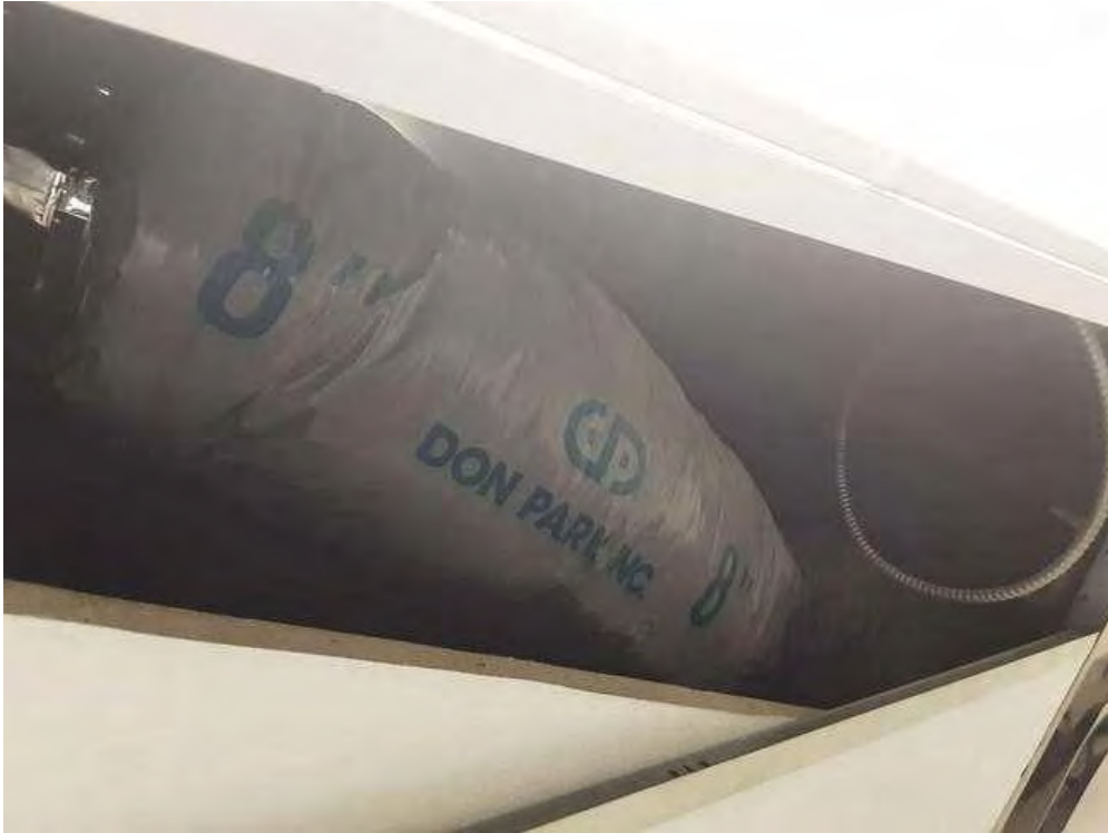
V0000 (None), Duct, Fibreglass, Washrooms (Location #: 28)
