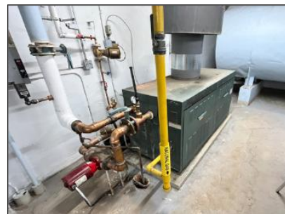
Uninsulated Boiler, Mechanical Room 2 (Loc.55).
