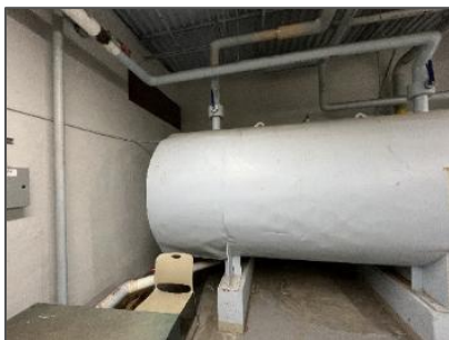
Fibreglass insulation on hot water tank, Mechanical Room 2 (Loc.55).
