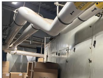
Fibreglass insulation on pipe, Mechanical Room 1 (Loc.57).
