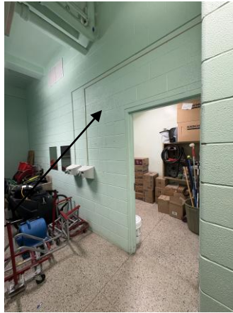
Figure 1: View of Lead-containing Paint on Concrete Block wall within Girl's Washroom - 1128
